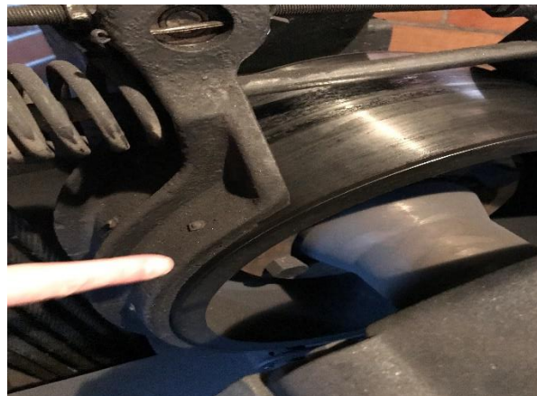
Photo #6 View of elevator brake pad. Asbestos presumed.
