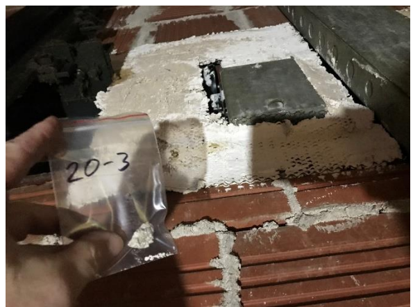
Photo #4 View of the 1 st Floor North Side Plaster Patch sampled, no asbestos detected.
