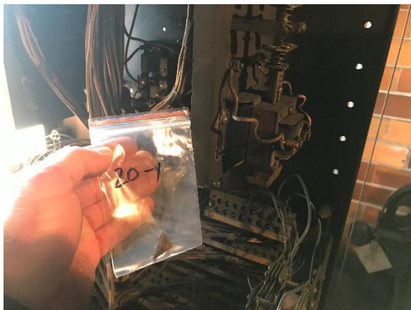
Photo #1 View of the Upper Circuit Breaker Board sampled, contains 8% asbestos.
