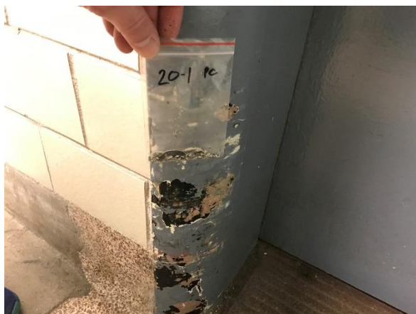
Photo #3 View of the Lead-Containing Paint on the 1 st Floor Elevator Door Frame.
