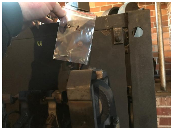
Photo #2 View of the Lower Circuit Breaker Board sampled, contains 8% asbestos.
