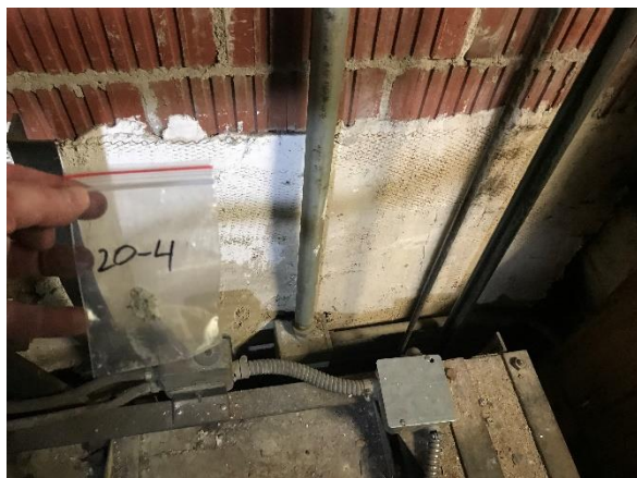
Photo #5 View of the B-1 North side Plaster Patch sampled, no asbestos detected.
