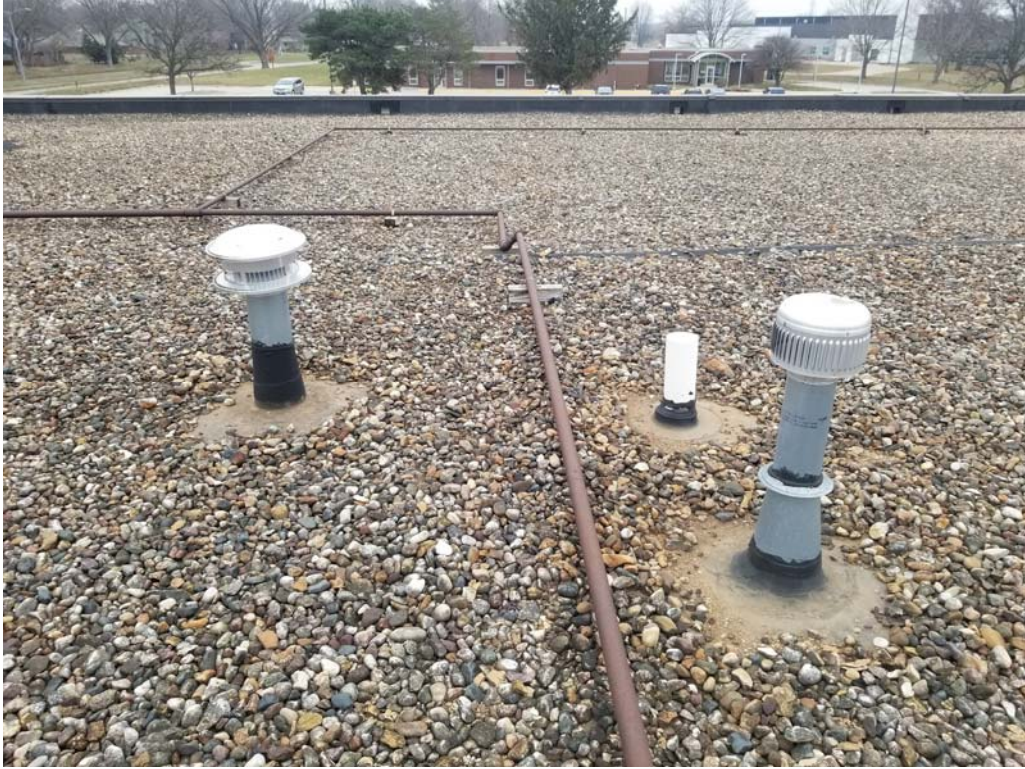
CENTER - VENTS & GAS PIPING
