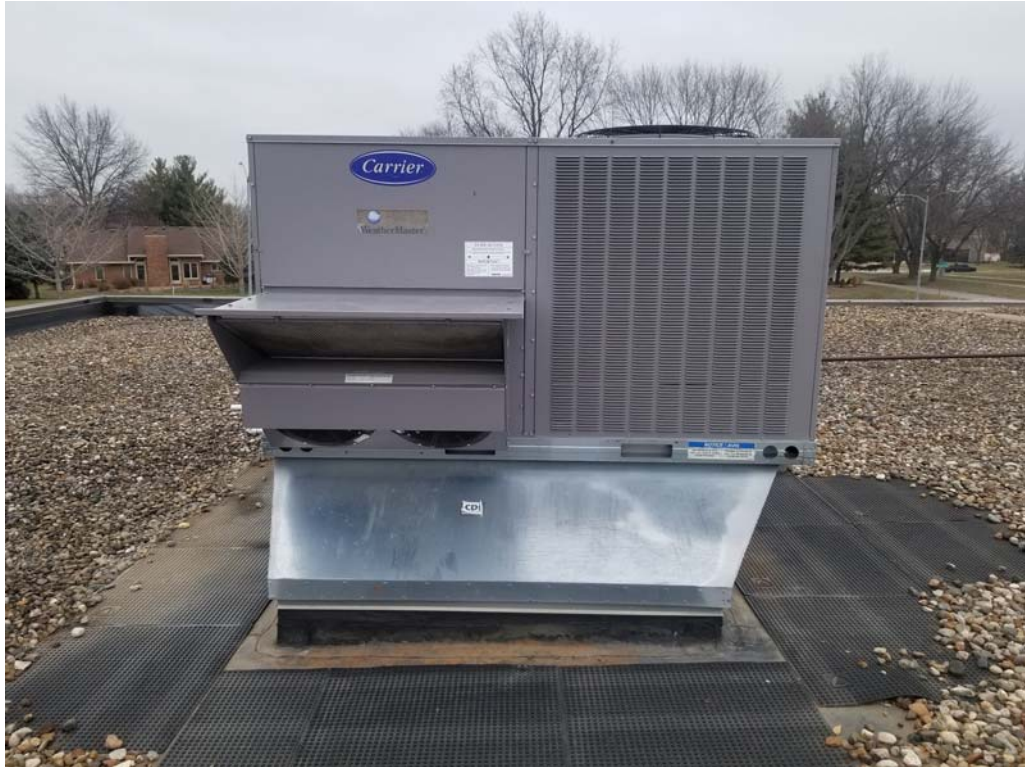
ROOF TOP HVAC UNIT
