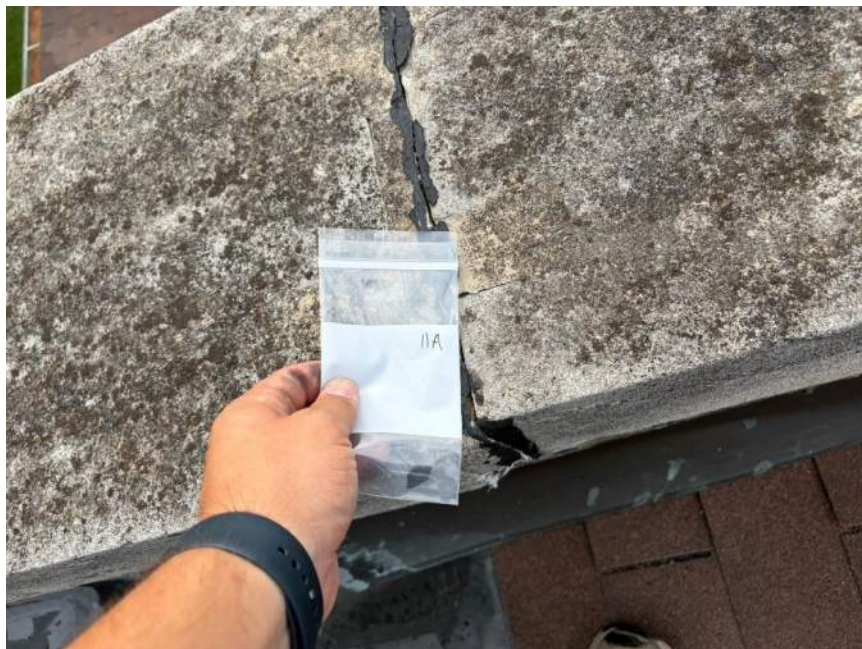
11A-Roofing Tar, Middle Upper Roof Northern Parapet Seam-Chrysotile 3%
