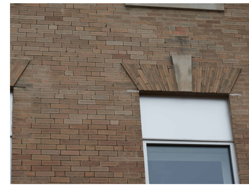
H1 LEVEL 1 - MORTAR DETERIORATION NTS
