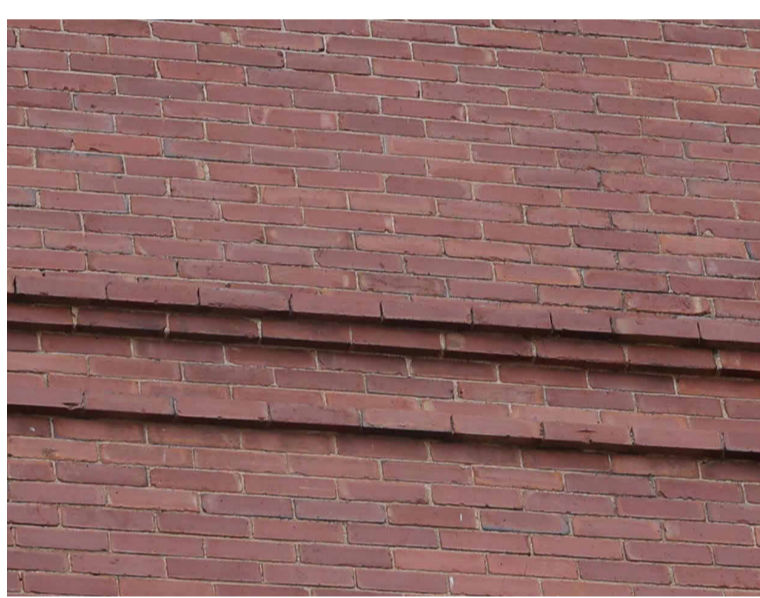
H11 LEVEL 1 - MORTAR DETERIORATION NTS
