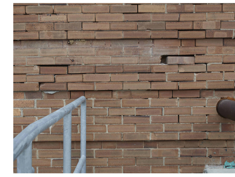
H11 LEVEL 3 - MORTAR DETERIORATION NTS
