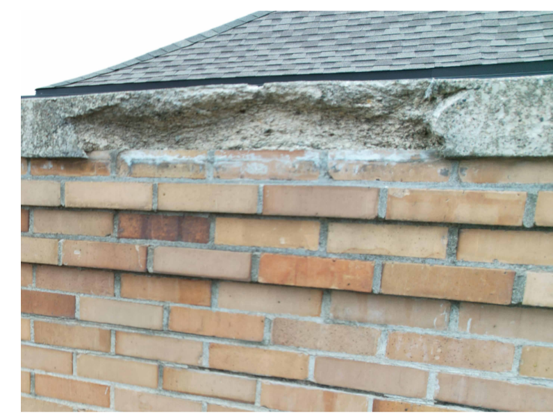
D1 DAMAGED STONE CAP NTS
