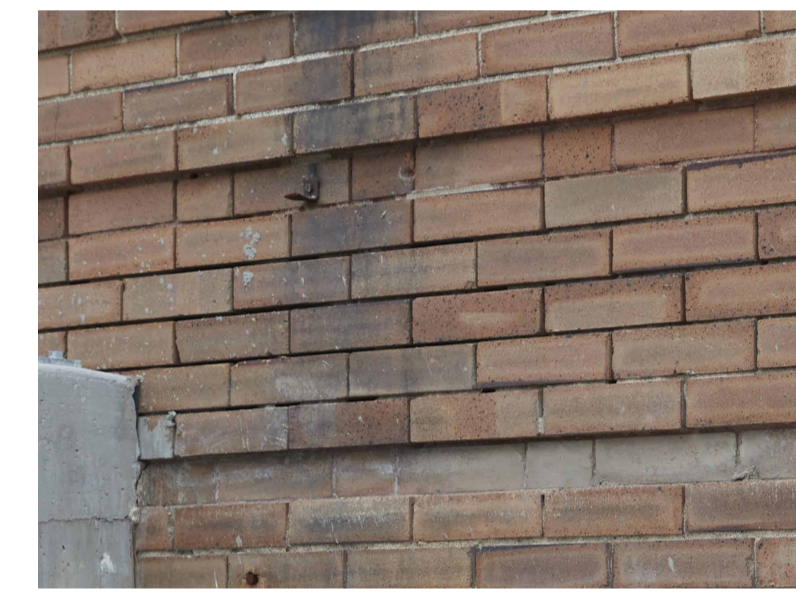
H6 LEVEL 2 - MORTAR DETERIORATION NTS
