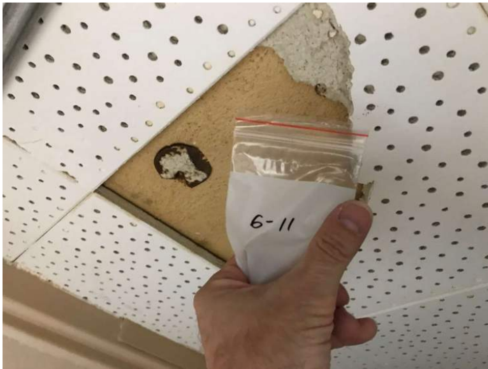
View of asbestos containing Brown Puck (Sample 5/6-17 – 5% Anthophyllite).
