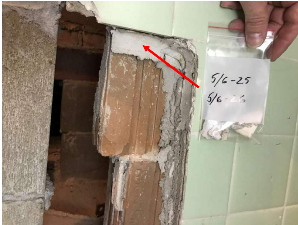
View asbestos containing light gray paper on old duct. (5/6-26 – 65% Chrysotile)
