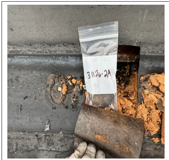
Sample 31126-2A: Flashing on canopy roof positive for asbestos.
