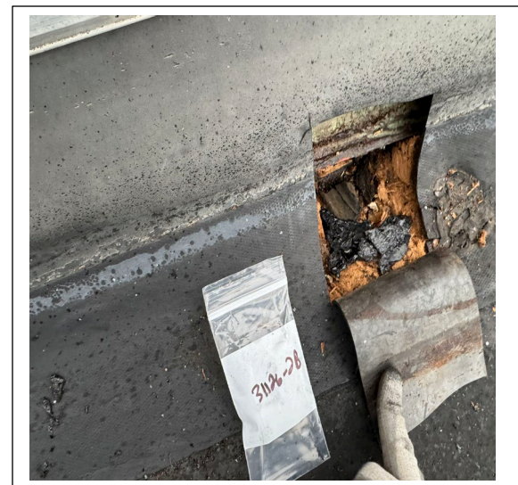
Sample 31126-2B: Flashing on canopy roof positive for asbestos.
