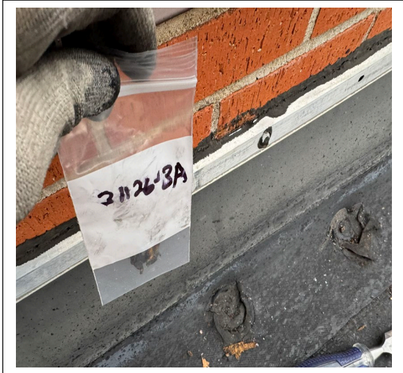
Sample 31126-3A: Caulking on flashing termination bar negative for asbestos.
