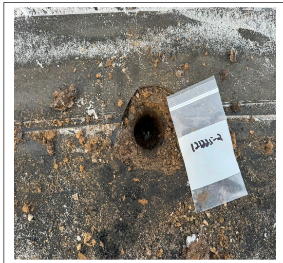
Sample 121225-2: Vapor barrier under flashing on West edge, main roof of warehouse negative for asbestos.
