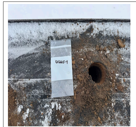
Sample 121225-4: Vapor barrier on East edge, main roof below flashing negative for asbestos.
