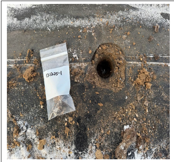
Sample 121225-1: Flashing on West edge, main roof of warehouse negative for asbestos.
