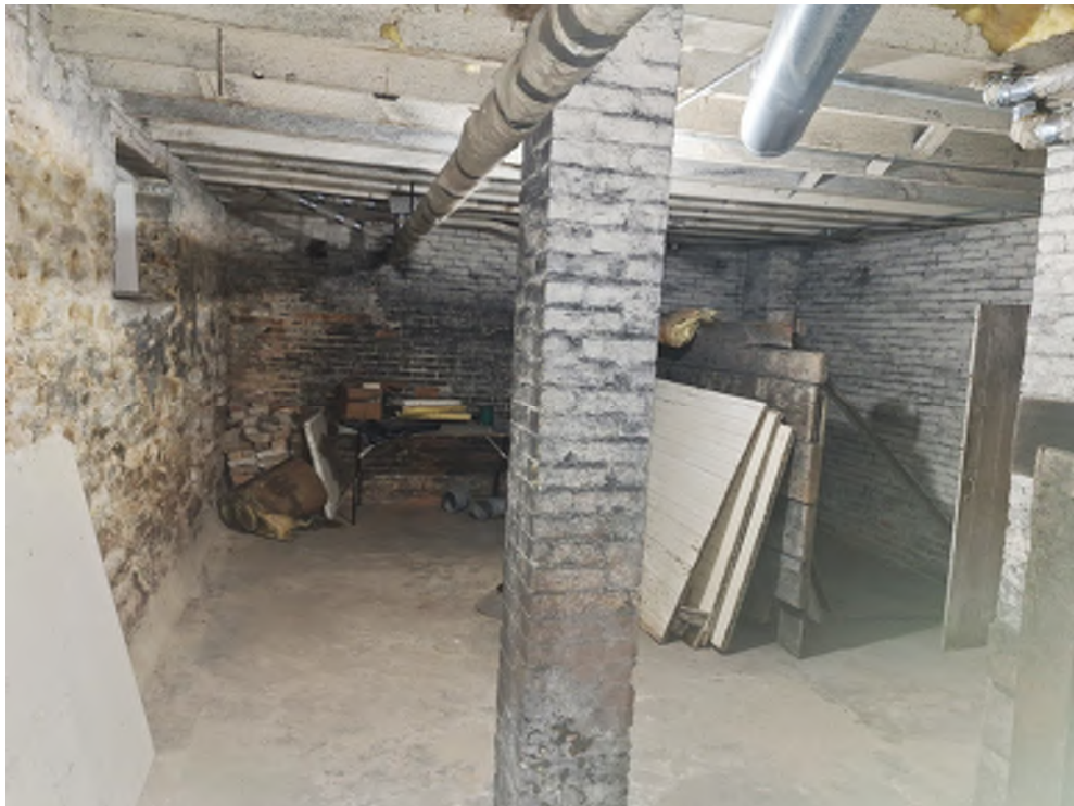
EAST MANSION BASMENT ROOM - CORNER FOR DEHUMIDIFIER
