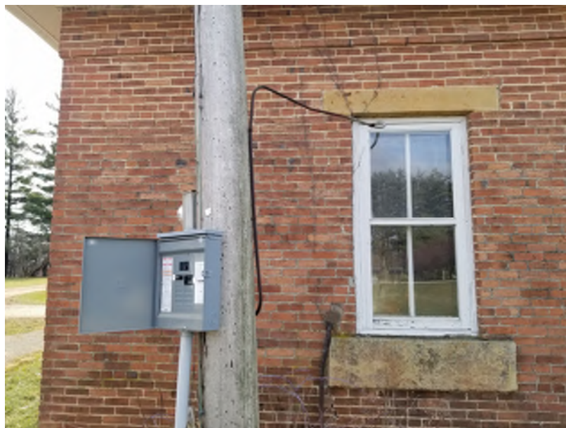
ELECTRICAL BOX OFF OVERHEAD POLE TO WORKSHOP
