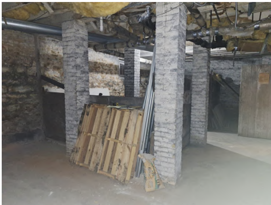
EAST BASMENT ROOM FOR DEHUMIDIFIER
