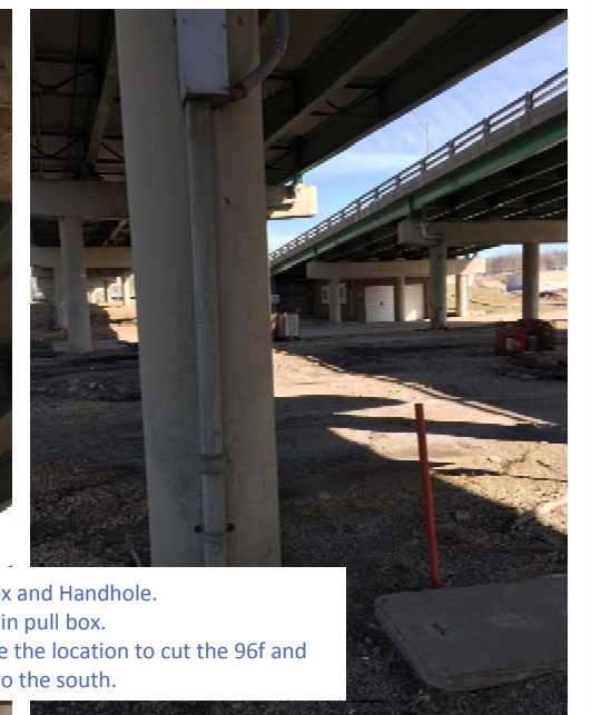
Pier 30 Gilbert St – Ex. I-74 Riser & Handhole
