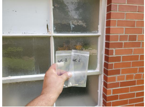
Photo #2 Sample WC-8. Asbestos Containing White Window Caulk Around Window of Area H Building.
