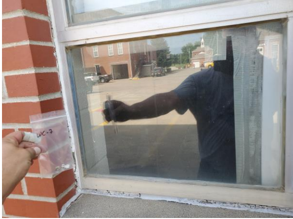
Photo #1 Sample WC-7. Asbestos Containing White/Tan Window Caulk Around Windows of Area I Building (receiving).
