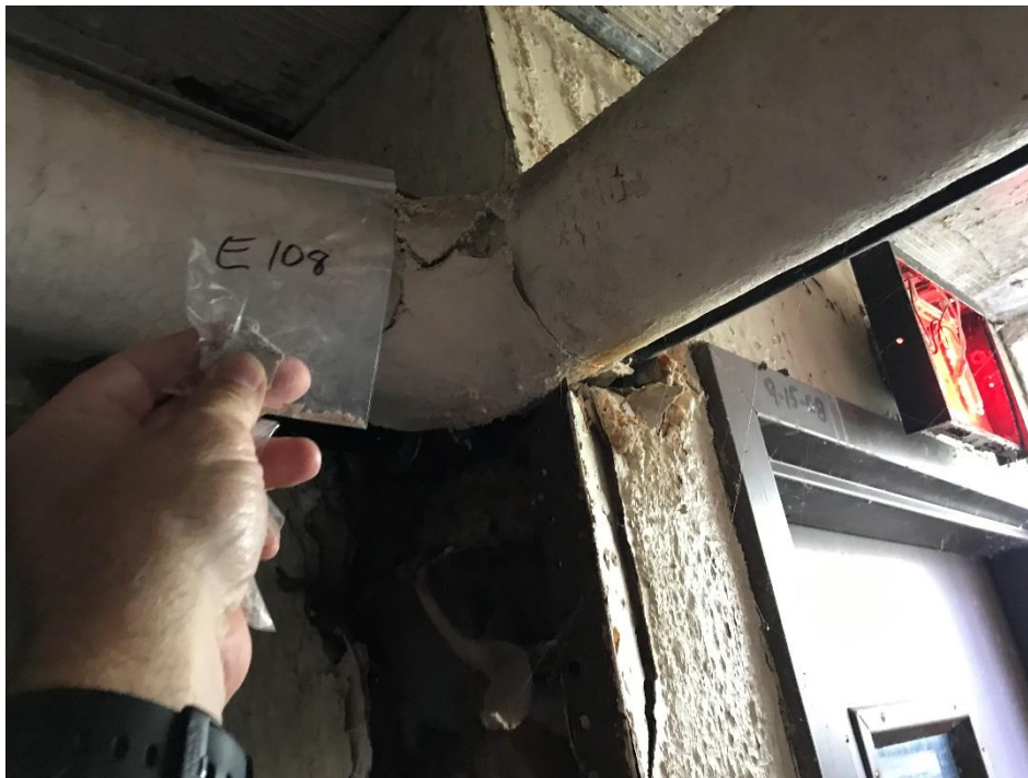
View of the Asbestos Containing TSI Elbow & Texture. (E 108, 55% & 2% Chrysotile)
