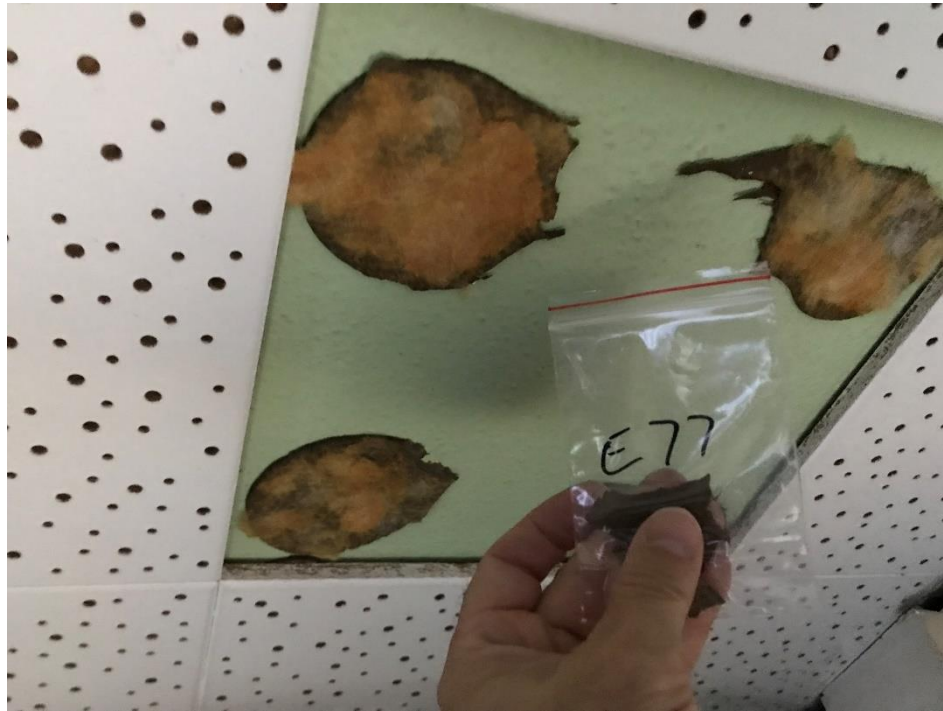
View of the Asbestos Containing Brown Pucks. (E 77, 4% Chrysotile)
