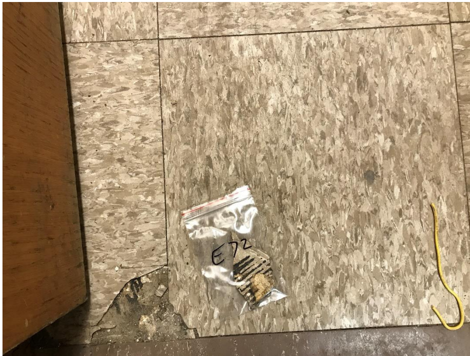
View of the Asbestos Containing Black Mastic. (E 72, 4% Chrysotile)
