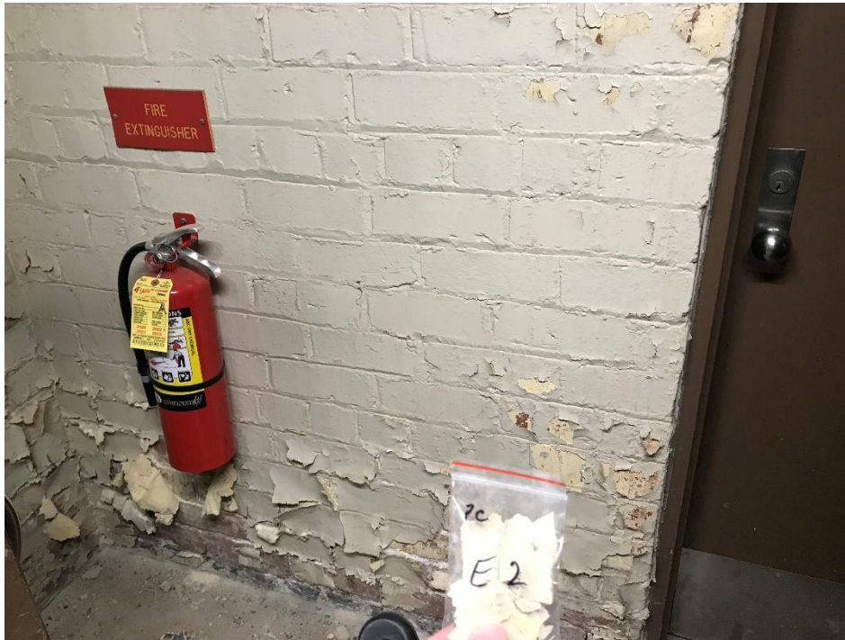
View of the Dull Green Lead Containing Paint. (PC E 2, 0.15% Pb)
