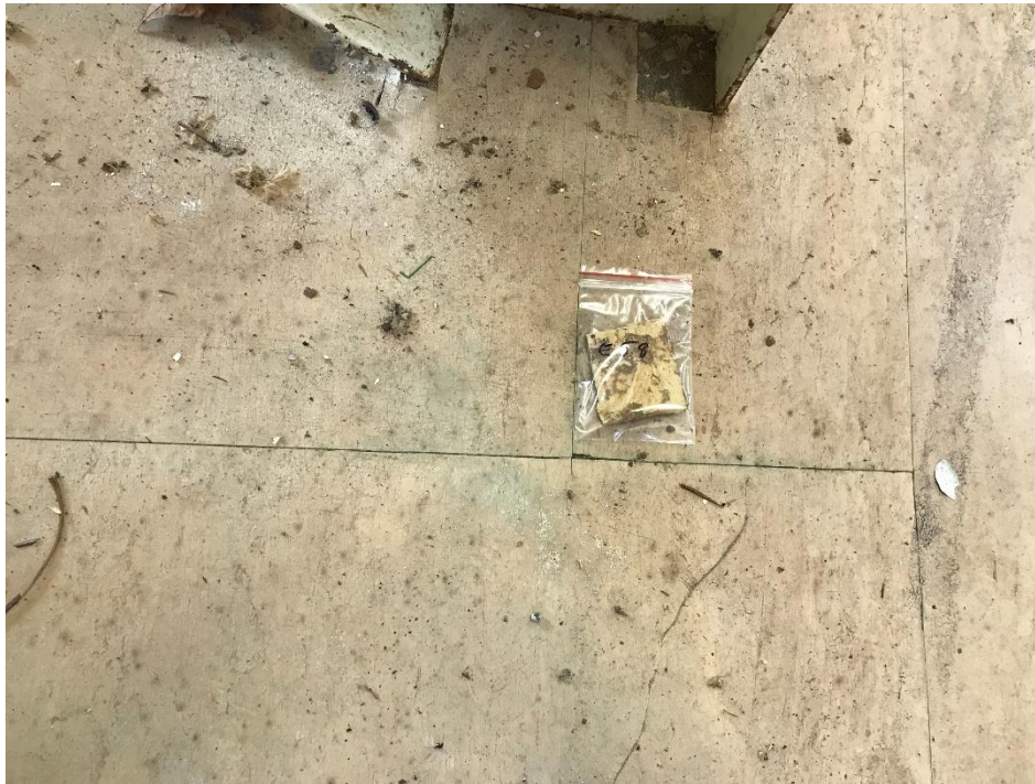
View of the Asbestos Containing Yellow/Brown Mastic & Gray Backing. (Under Lt Brown Flooring) (E 58, 1% & 25% Chrysotile)
