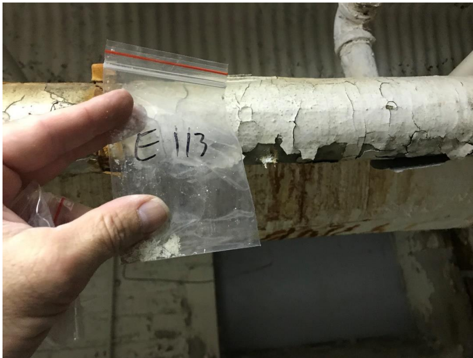
View of the Asbestos Containing TSI Run. (E 113, 15% Amosite 30% Crocidolite)
