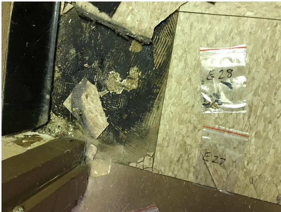
View of the Asbestos Containing Black Mastic and Gray Backing. (E 28, 3% & 25% Chrysotile)
