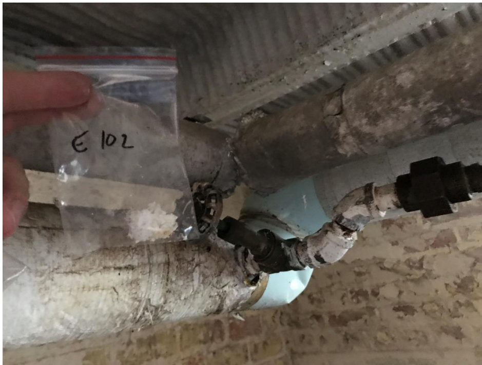
View of the Asbestos Containing TSI Elbow. (E 102, 15% Amosite & 20% Chrysotile)
