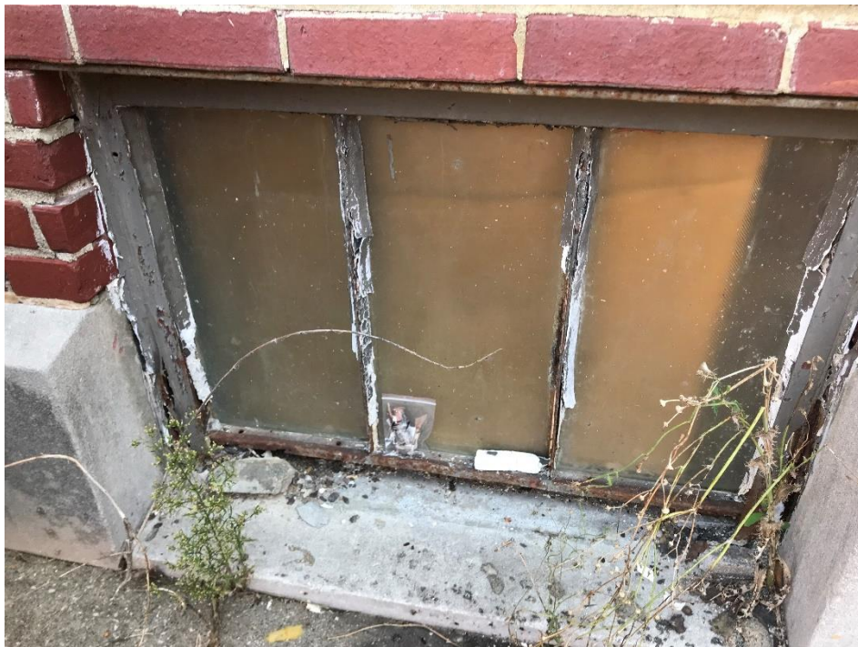
View of the Asbestos Containing Window Glazing. (E 1, 3% Chrysotile)
