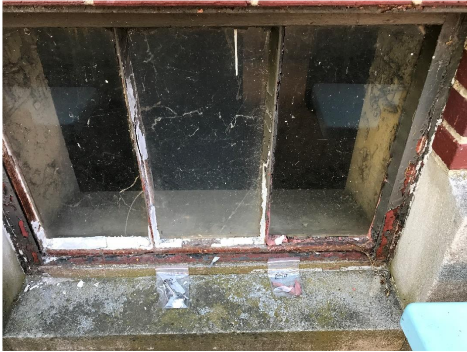
View of the Asbestos Containing Window Glazing. (E 9, 4% Chrysotile)
