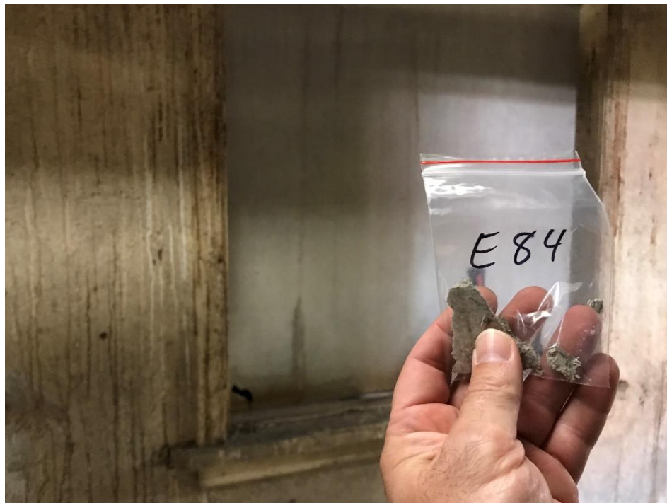
View of the Asbestos Containing Transite Panes. (E 84, 20% Chrysotile)
