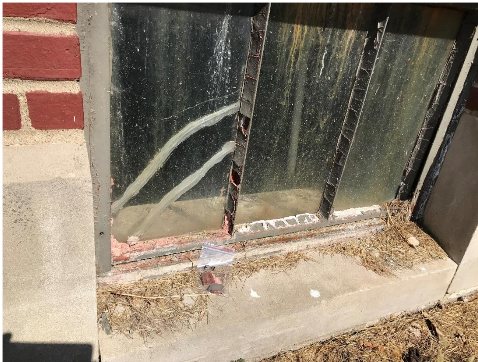
View of the Asbestos Containing Red Window Glazing. (E 8, 2% Chrysotile)
