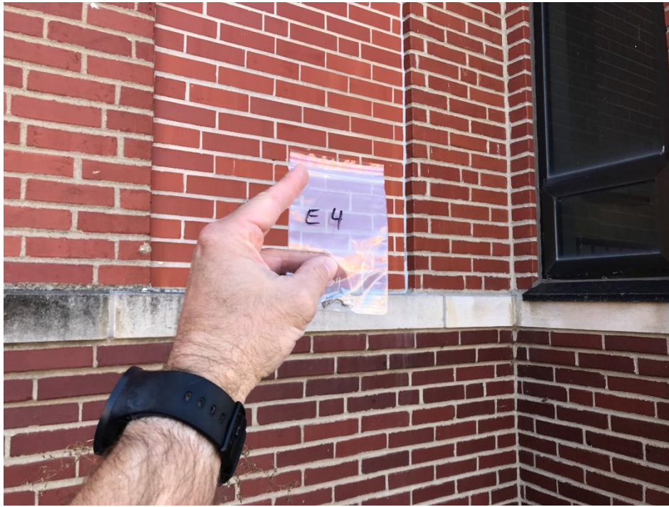
View of the Asbestos Containing Gray Caulk. (E 4, 4% Chrysotile)
