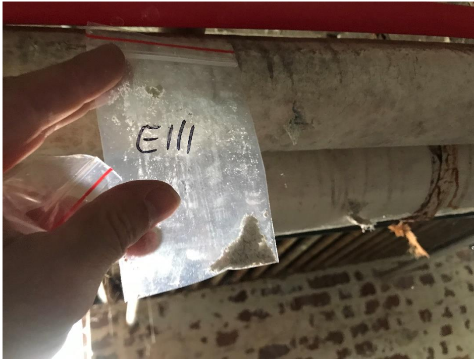
View of the Asbestos Containing TSI Run. (E111, 5% Amosite & 35% Crocidolite)
