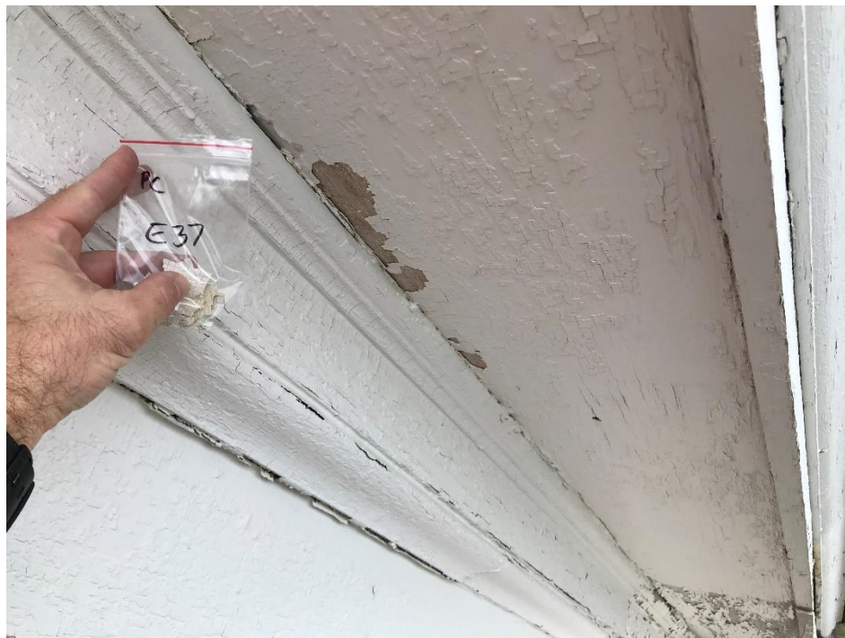
View of the White Lead Based Paint. (PC E 37, 28% Pb)
