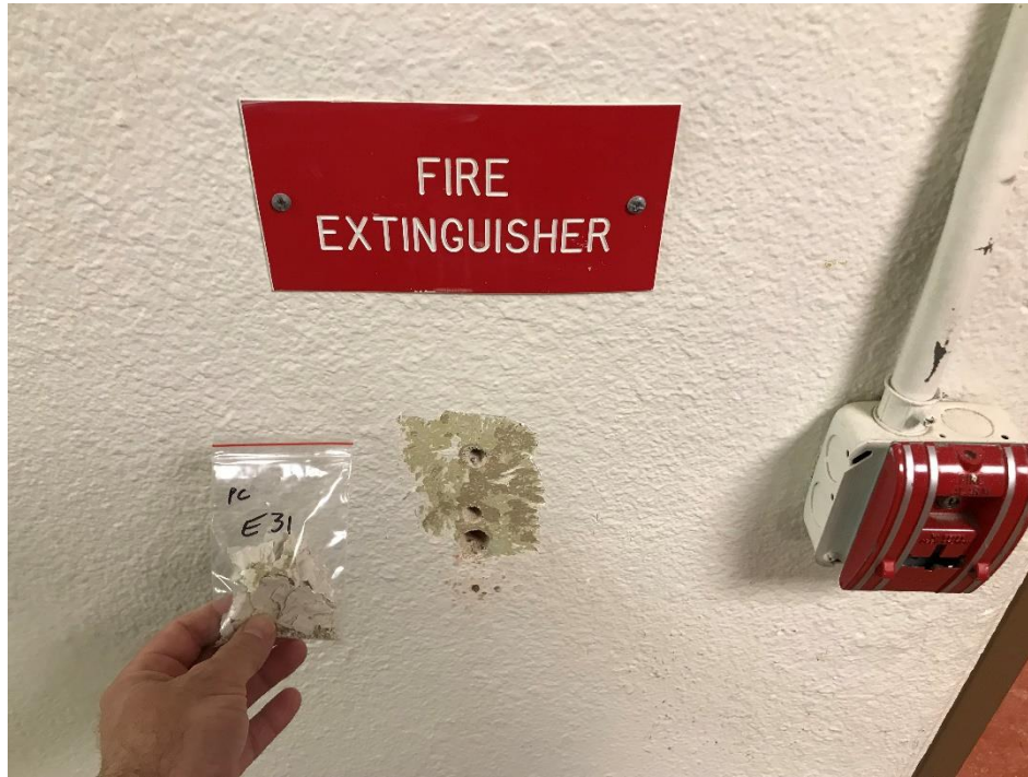
View of the White Lead Based Paint. (PC E 31, 1.7% Pb)
