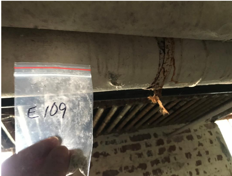
View of the Asbestos Containing TSI Run. (E 109, 30% Amosite & 15% Crocidolite)
