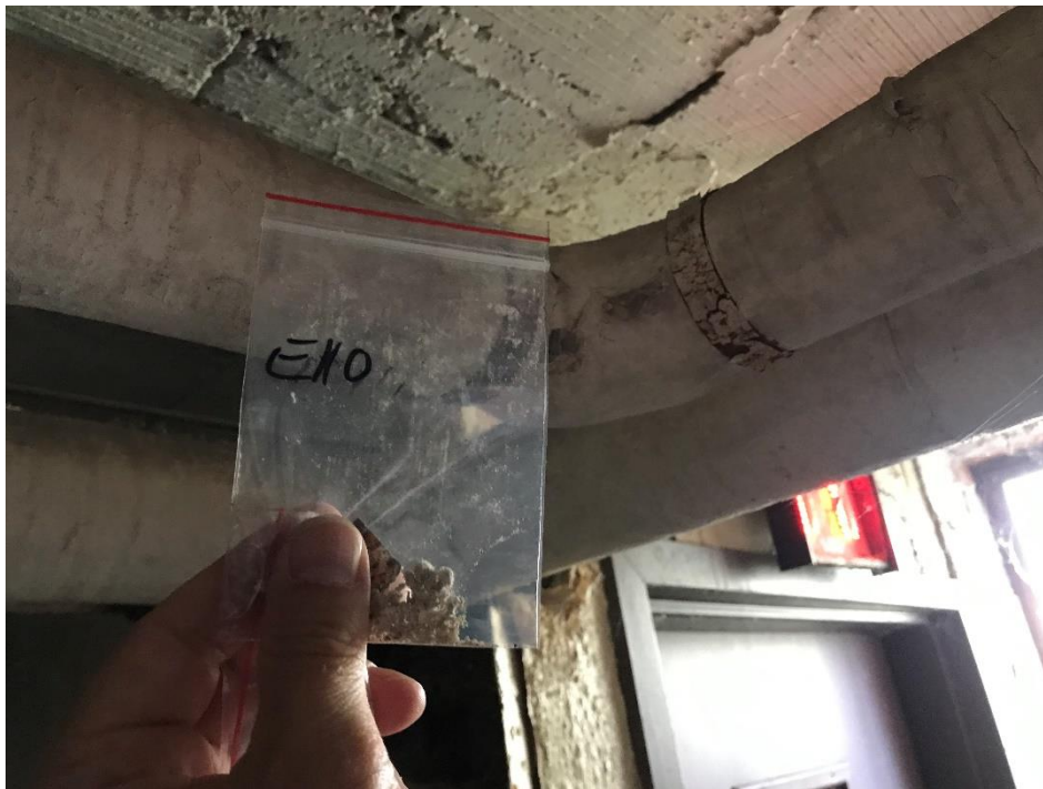
View of the Asbestos Containing TSI Elbow & Texture. (E 110, 60% & ,1% Chrysotile)
