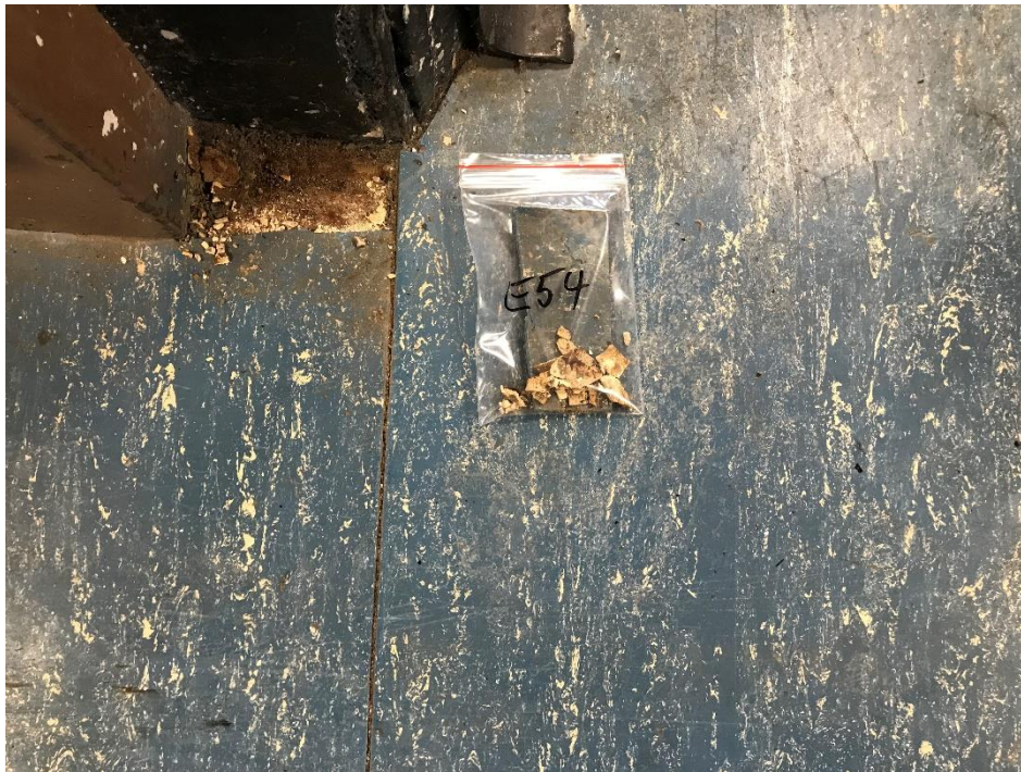
View of the Asbestos Containing Gray Backing. (Under Blue Flooring) (E 54, 15% Chrysotile)
