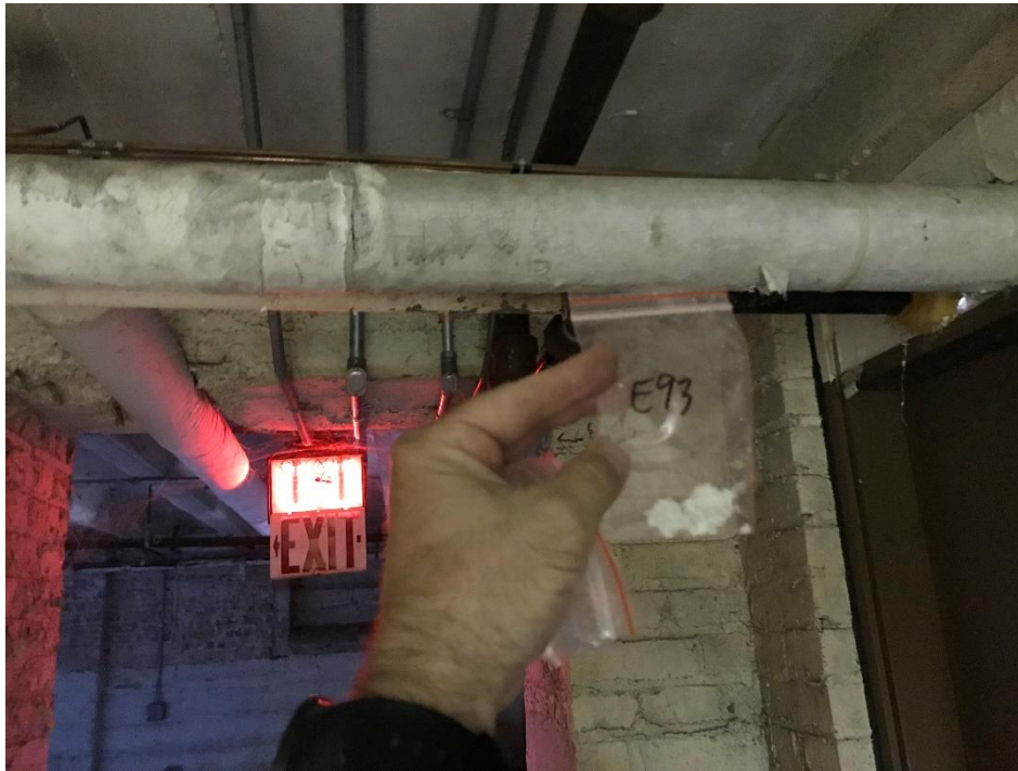
View of the Asbestos Containing TSI Run. (E 93, 15% Amosite & 20% Crocidolite)
