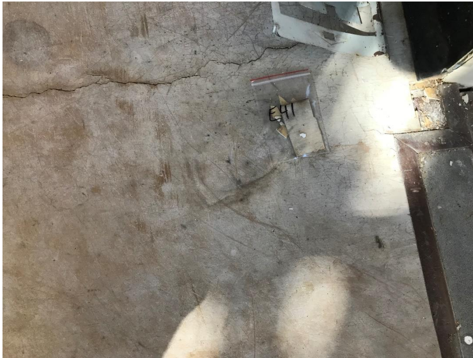
View of the Asbestos Containing Gray Backing (Under Lt Brown Flooring). (E 41, 20% Chrysotile)
