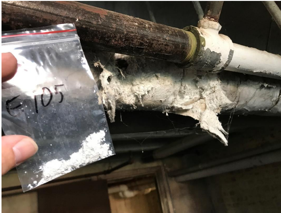
View of the Asbestos Containing TSI Run. (E 105, 35% Amosite & 15% Crocidolite)
