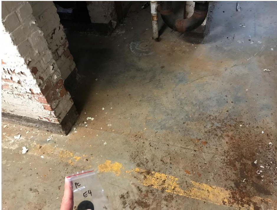
View of the Yellow Lead Based Paint. (PC E 4, 18% Pb)
