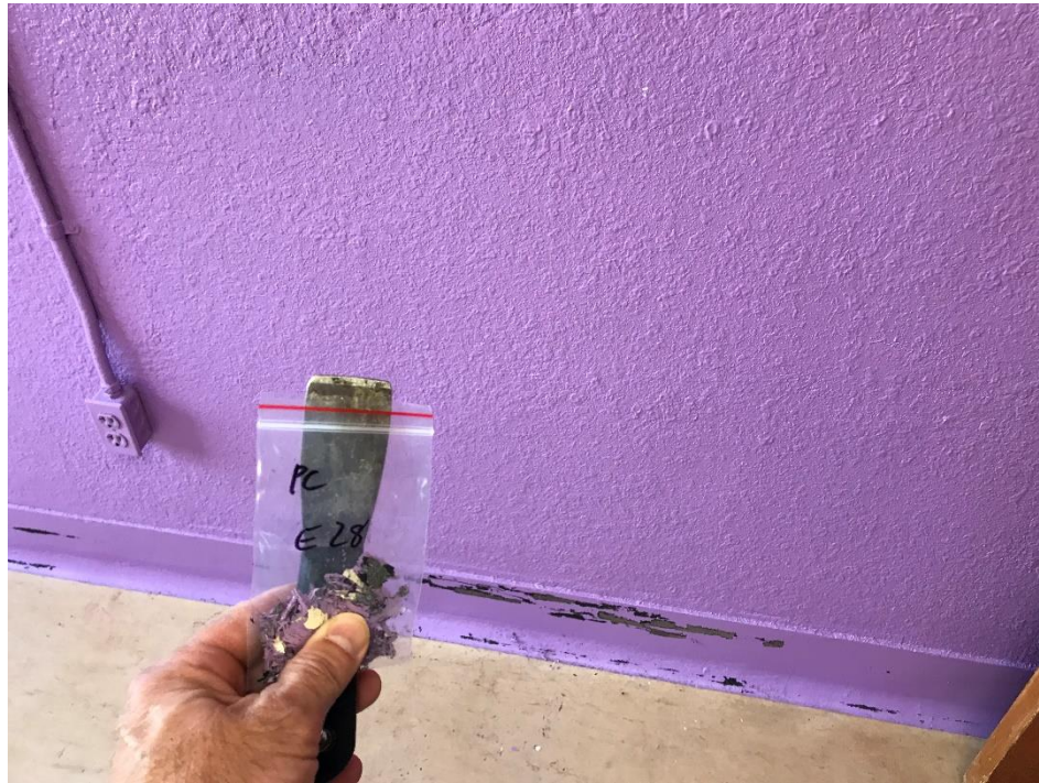
View of the Lavender Lead Containing Paint. (PC E 28, 0.059% Pb)
