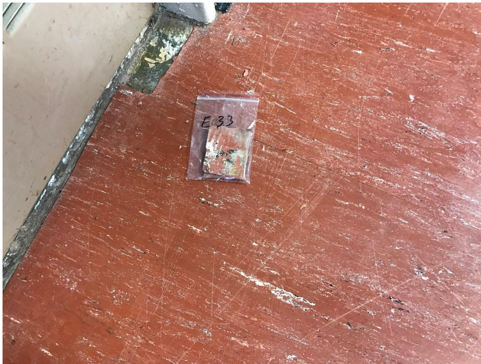
View of the Asbestos Containing Yellow/Black Mastic. (E 33, <1% Chrysotile)
