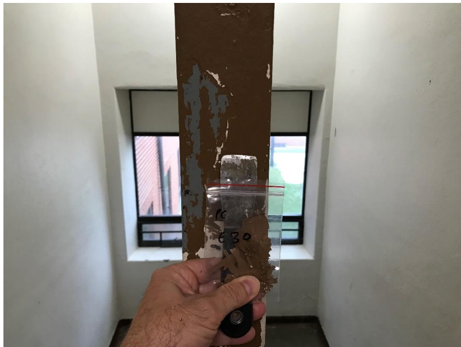
View of the Brown Lead Containing Paint. (PC E 30, 0.11% Pb)
