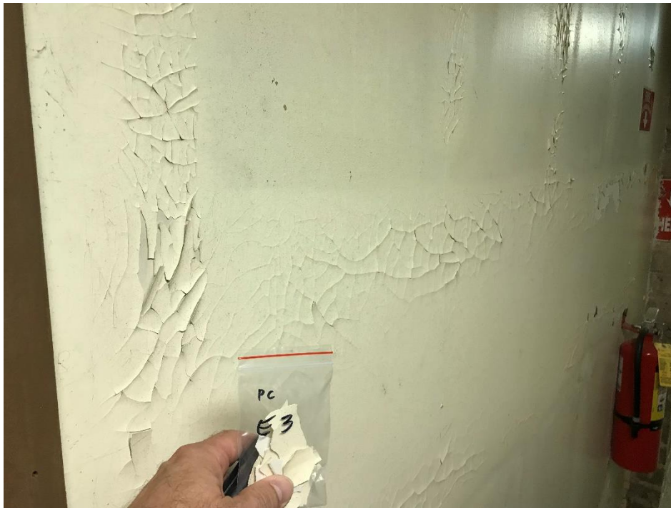
View of the Dull Pale Yellowish White Lead Containing Paint. (PC E 3, 0.027% Pb)
