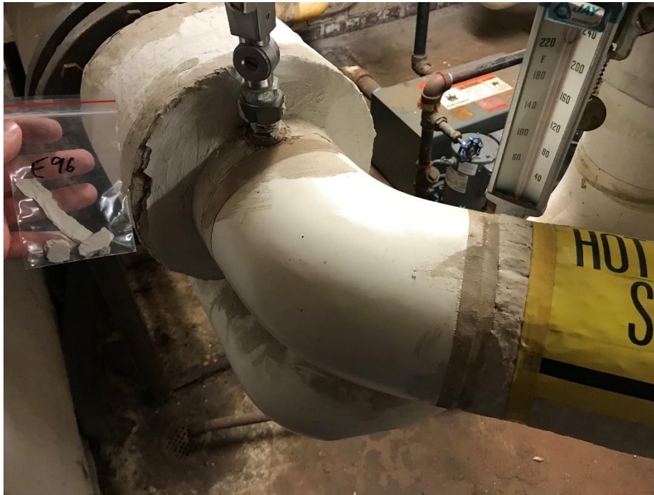
View of the Asbestos Containing Caulk. (E 96, 3% Chrysotile)
