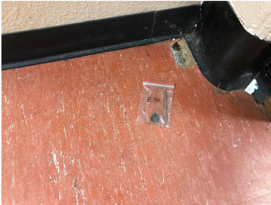
View of the Asbestos Containing Black/Yellow Mastic. (E 31, <1% Chrysotile)
