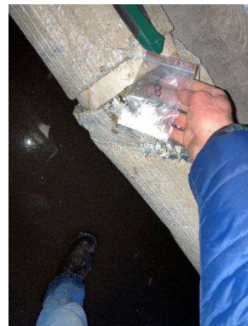
Photo #6 Asbestos: Sample #8 – 6"-8" O.D Straight Pipe Insulation Section #2 Pipe E.
