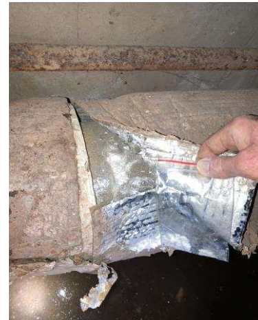
Photo #4 Asbestos: Sample #5 – 6"-8" O.D Straight Pipe Insulation Section #1 Pipe E.
