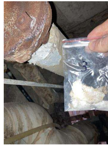
Photo #2 Asbestos: Sample #3 – 4"-6" O.D Straight Pipe Insulation Section #1 Pipe H
