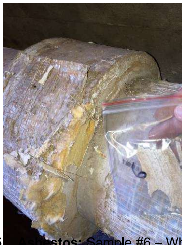
Photo #5 Asbestos: Sample #6 – White Pipe End Caulk/Sealant Section #2 Pipe F.
