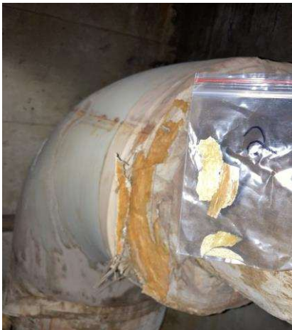
Photo #1 Asbestos: Sample #2. White Pipe End Caulk/Sealant. Same material observed on Pipes G & F throughout.
