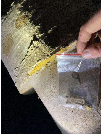
Photo #7 Asbestos: Sample #9 – White Pipe End Caulk/Sealant Section #3 Pipe F.
