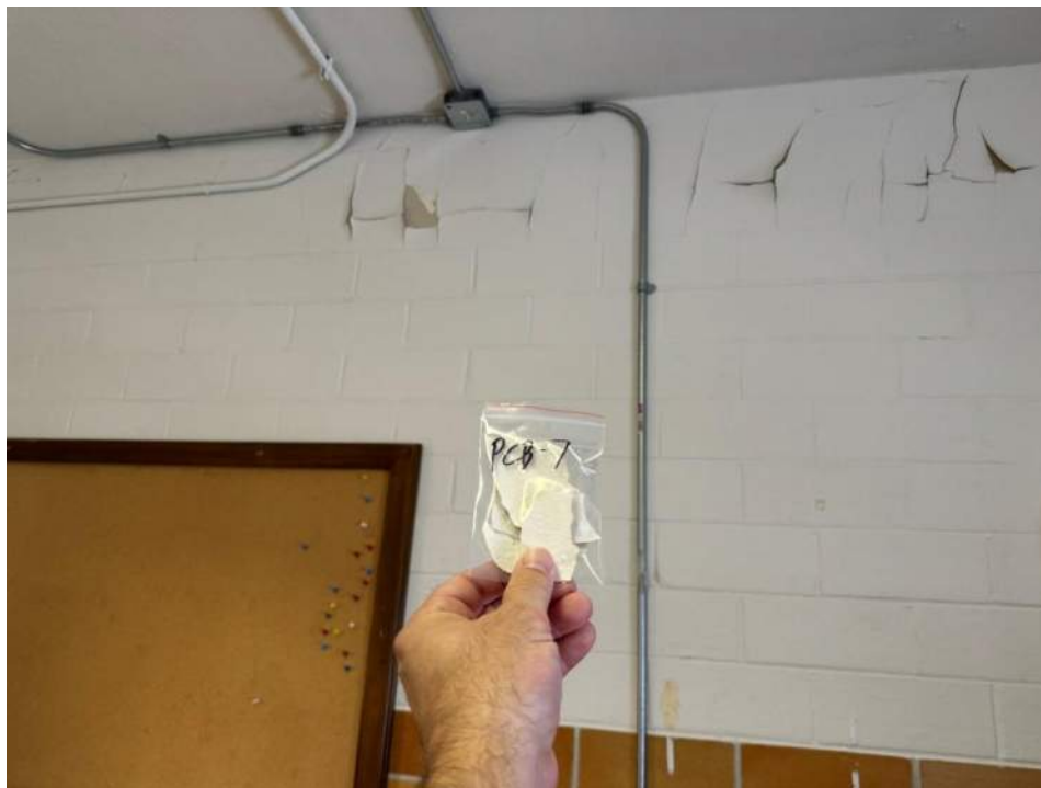
View of the White Lead Containing Paint. (PCB-7, 0.046% Pb)
