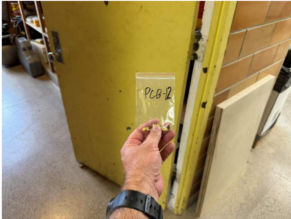
View of the Yellow Lead Containing Paint. (PCB-12, 0.29% Pb)
