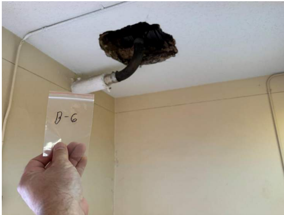
View of the Asbestos Containing White Pipe Insulation. (B-6, 45% Chrysotile)
