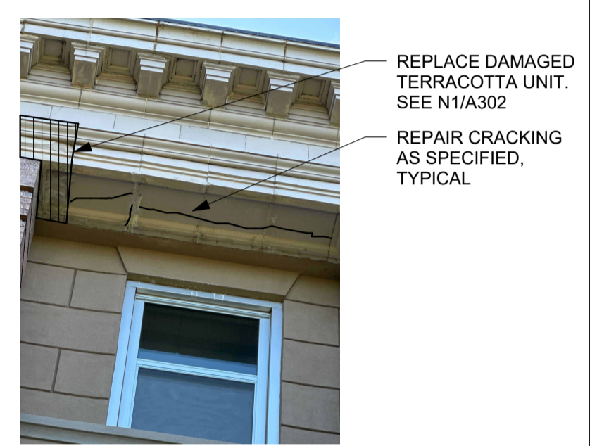
M23 PHOTO - LIMESTONE CRACKING 3 1/8" = 1'-0"
