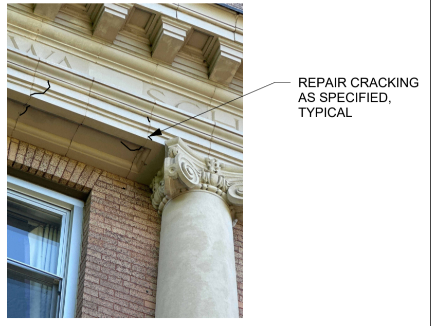
J23 PHOTO - LIMESTONE SOFFIT CRACKING 2 1/8" = 1'-0"
