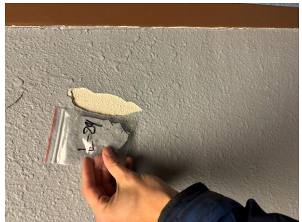
Photo #30 Sample L-29 – Grey Lead-based Paint on Plaster Wall in Larches 2 nd Floor.
