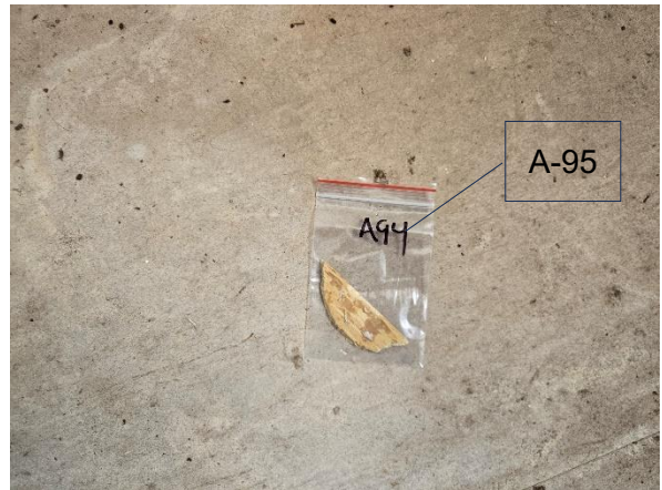
Photo #16 Sample A-95. Hemlock, Asbestos Containing Vinyl Sheet Flooring.
