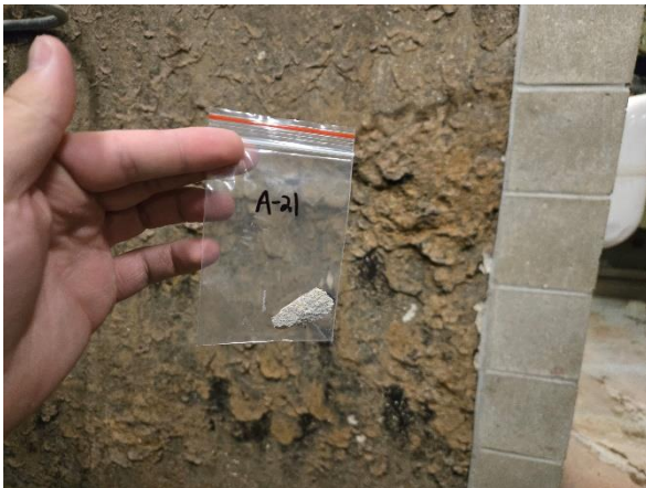
Photo #3 Sample A-21. Chiller, Asbestos Containing Black Tar Vapor Barrier.
