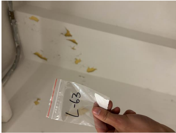
Photo #37 Sample L-63 – White Lead-based Paint on Concrete Wall in Employee Home Basement South Wing.
