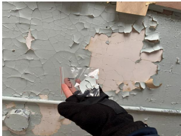
Photo #21 Sample L-4 – Blue Lead-based Paint on Plaster Ceiling in Oak Hall 2 nd Floor East Room.
