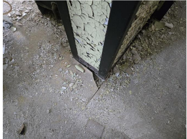
Photo #2 Sample A-8. Oak Hall, Asbestos Containing Vinyl Sheet Flooring and Black Mastic.
