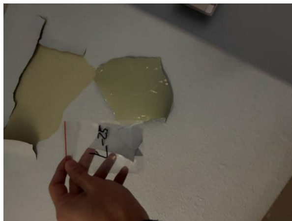
Photo #29 Sample L-25 – Blue Lead-based Paint on Plaster Wall in Larches 1 st Floor.
