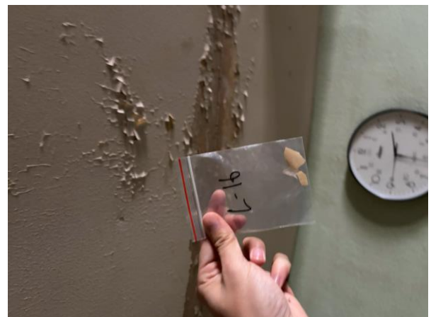
Photo #24 Sample L-16 – White Lead-based Paint on Plaster Wall in Supply Depot on 1 st Floor.
