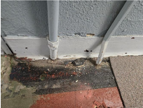
Photo #13 Sample A-71. Employee Home, Asbestos Containing Black Flooring
