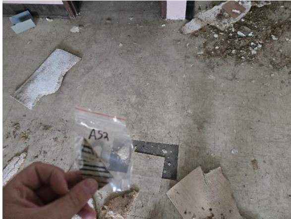
Photo #7 Sample A-52. Maple Lodge, Asbestos Containing 9" x 9" Floor Tile and Black Mastic.
