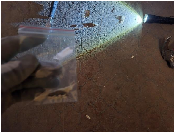
Photo #15 Sample A-72. Employee Home, Asbestos Containing Vinyl Sheet Flooring.
