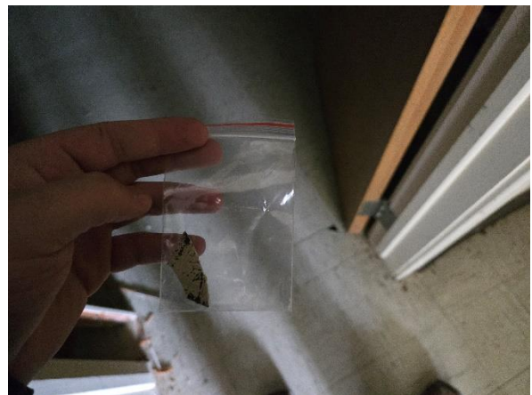
Photo #6 Sample A-59. Maple Lodge, Asbestos Containing 9" x 9" Floor Tile and Black Mastic.
