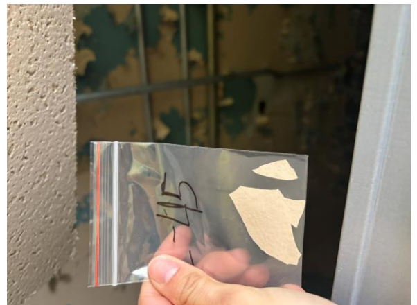
Photo #36 Sample L-45 – Brown Lead-based Paint on Plaster Ceiling in Maple 3 rd Floor.
