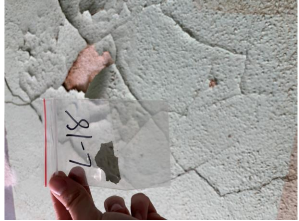
Photo #26 Sample L-18 – Green Lead-based Paint on Plaster Wall in Supply Depot 1 st Floor.
