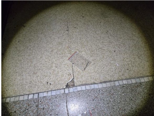
Photo #19 Sample A-102. Hemlock, Asbestos Containing Vinyl Sheet Floor and Black Mastic.
