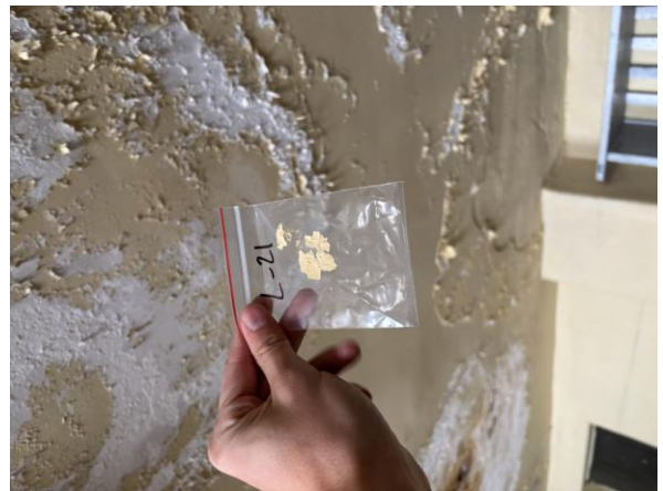
Photo #28 Sample L-21 – Yellow Lead-based Paint on Plaster Wall in Supply Depot 2 nd Floor.
