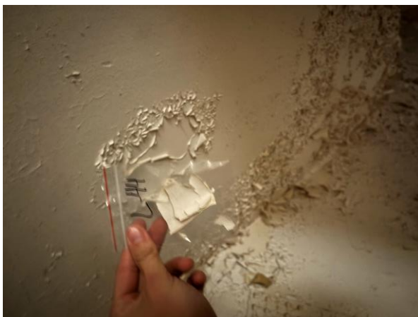
Photo #35 Sample L-44 – White Lead-based Paint on Plaster Wall in Maple 3 rd Floor.
