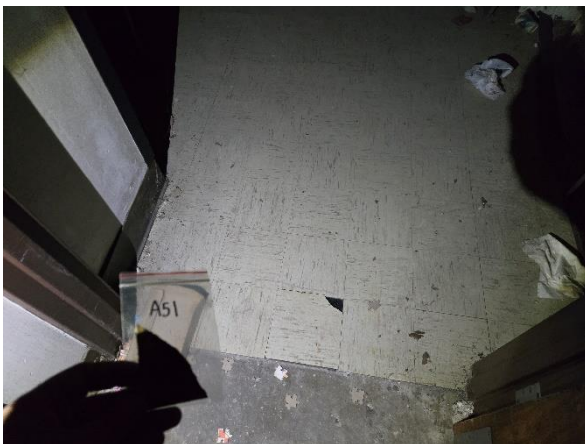
Photo #5 Sample A-51. Maple Lodge, Asbestos Containing 9" x 9" Floor Tile and Black Mastic.
