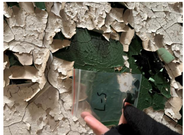
Photo #22 Sample L-5 – Green Lead-based Paint on Plaster Wall in Oak Hall 2 nd Floor North Central Stem Landing.
