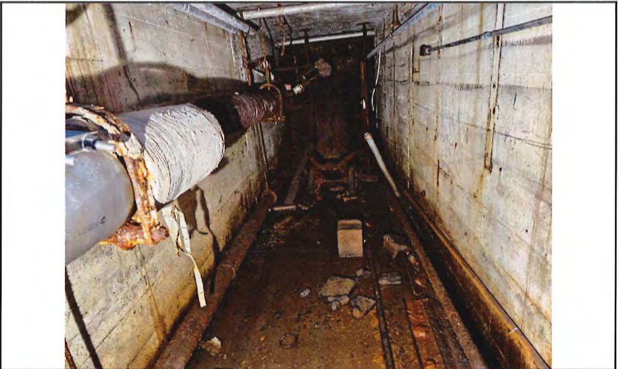
Photo 16: View of general debris and standing water.
