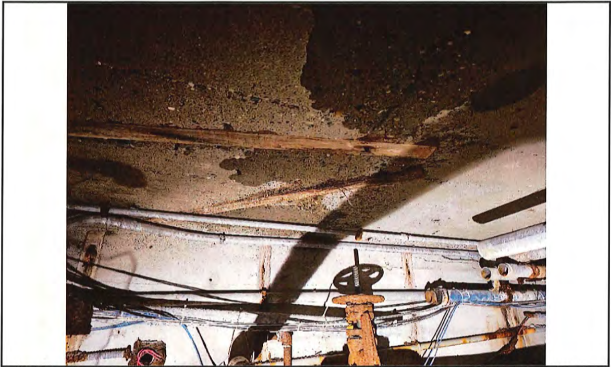
Photo 13: View of apparent moisture intrusion and cracked concrete on the ceiling.
