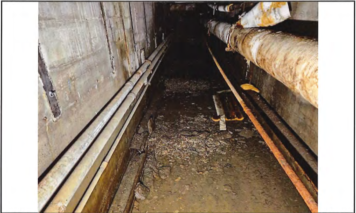
Photo 7: View of fiberglass piping, standing water, and debris from the deteriorating concrete ceiling.
