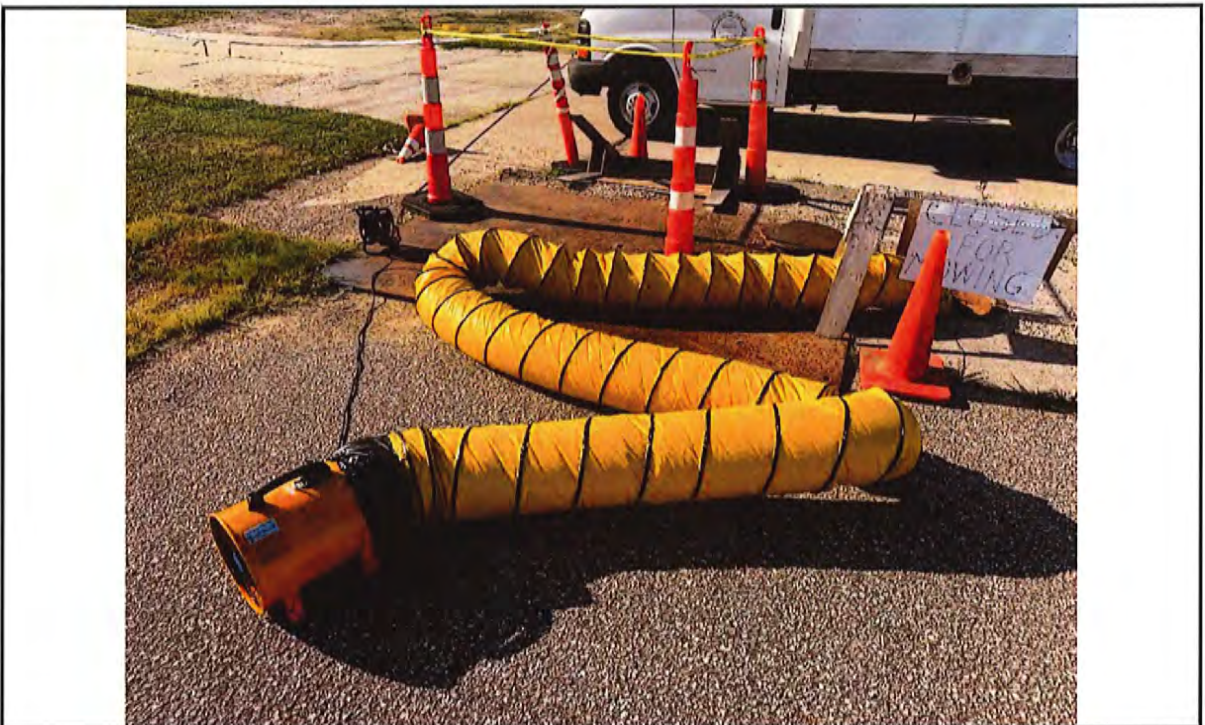
Photo 2: View of air circulation equipment utilized for tunnel.
