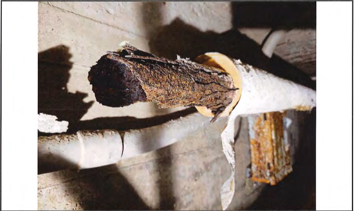
Photo 15: View of a corroded pipe, with non-asbestos containing fiberglass insulation.
