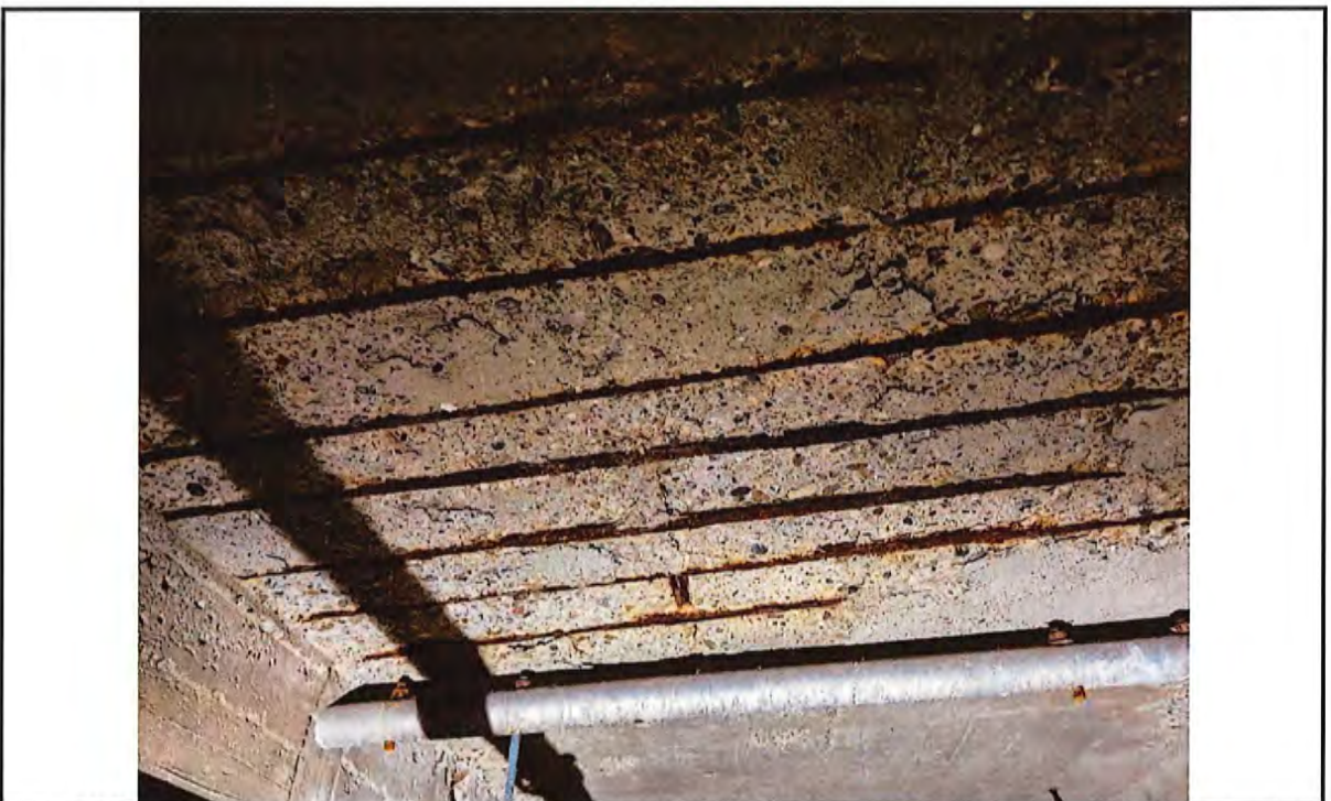
Photo 6: View of spalling concrete and exposed rebar on the tunnel ceiling.
