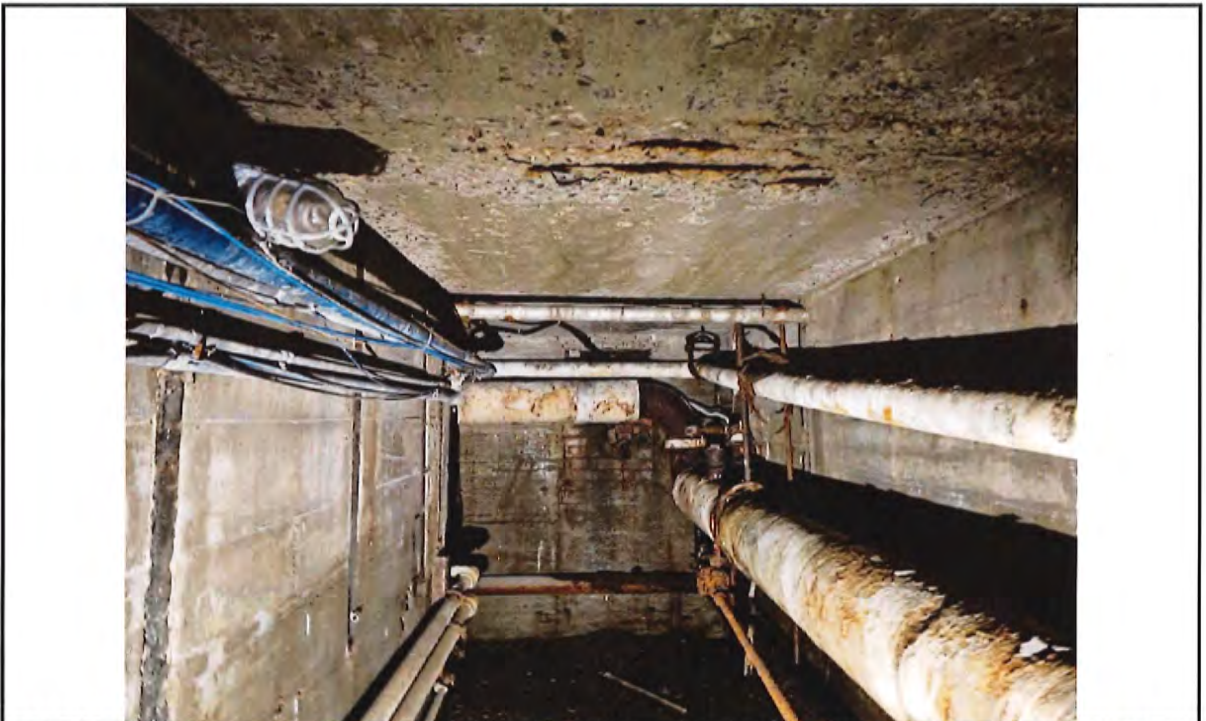
Photo 8: View of fiberglass piping and spalling concrete/exposed rebar on ceiling of utility tunnel.
