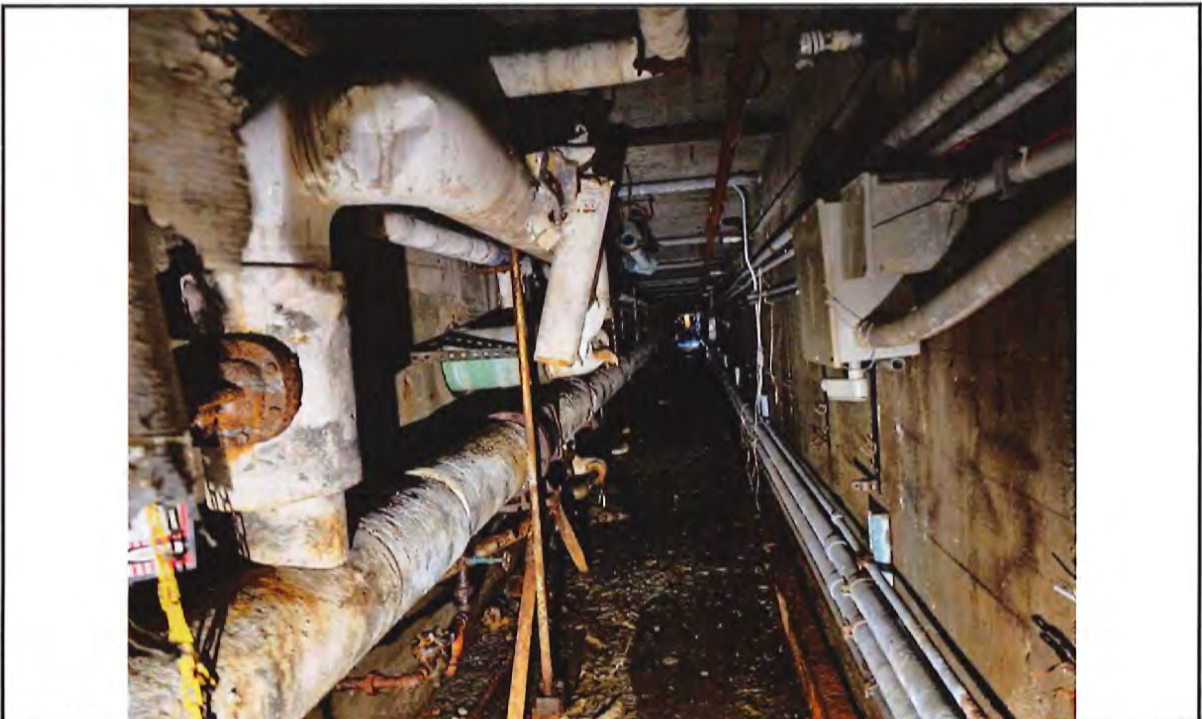
Photo 12: View of degraded non-asbestos containing fiberglass pipe insulation.
