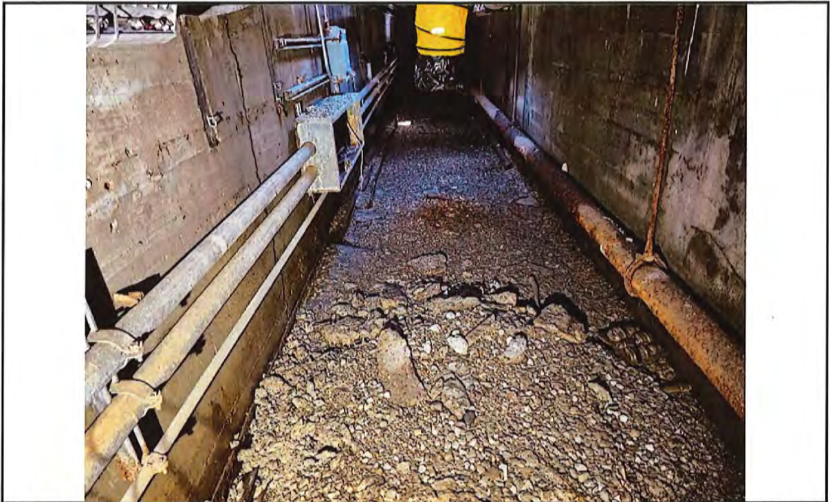
Photo 5: View of concrete debris on the floor of the tunnel from the deteriorating ceiling (as shown in photo 4).
