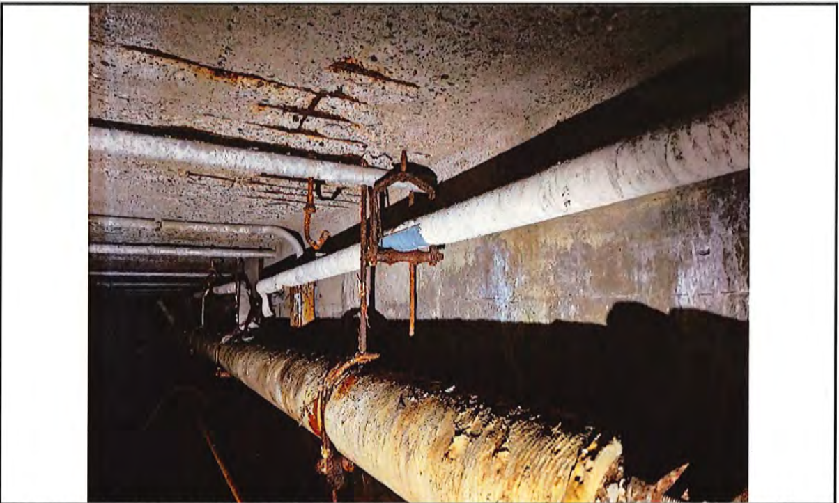
Photo 10: View of piping support brackets, fiberglass wrapped pipes, delaminated concrete and exposed rebar on ceiling.
