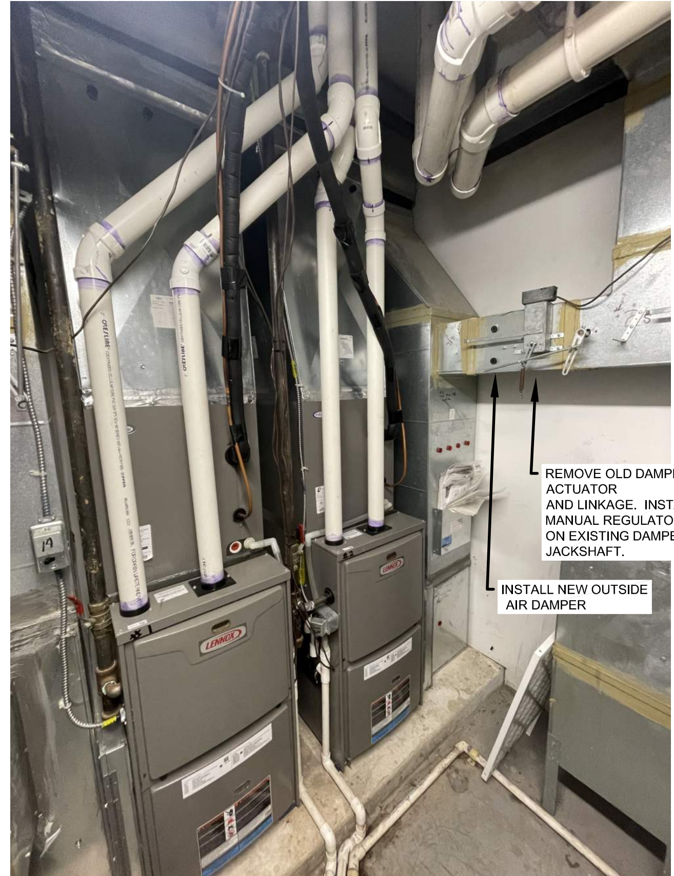
7 FURNACE OUTSIDE AIR PHOTO NO SCALE
