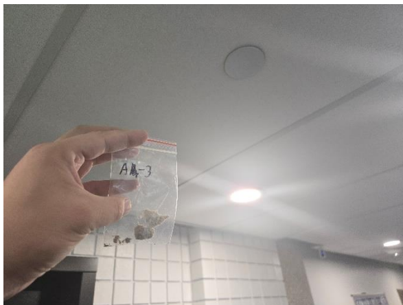
Photo #5 Non-ACM sample A-3. 2'X4' ceiling tile found in the hallway.
