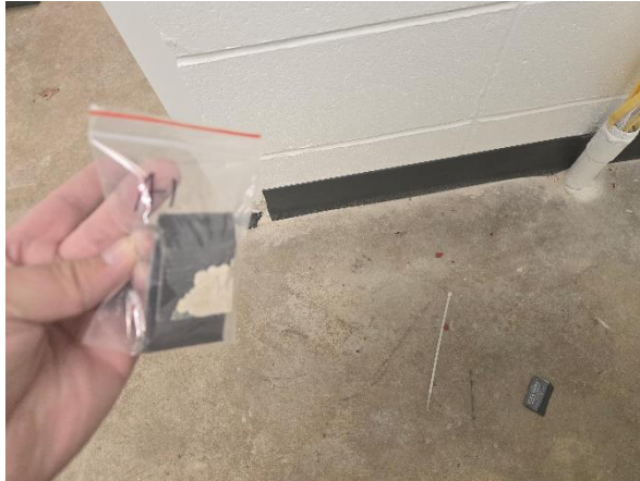
Photo #1 Non-ACM sample A-1. Base cove and adhesive found in the Mechanical Room.
