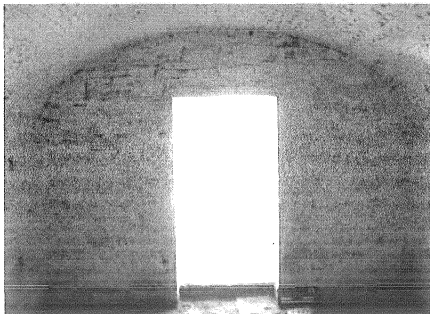
Figure 11. Powder Magazine interior photographs, 2006 (from Whittaker 2006d:75). Upper: facing east. Lower: facing west.
