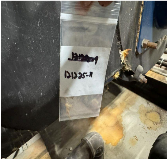
121225-11: Gasket material from front of boiler number 3 negative for asbestos.
