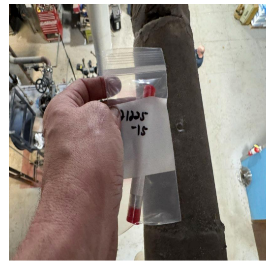
121225-15: TSI from white pipe directly above boiler number 3 positive for asbestos. (Believe new boiler will tie into this pipe).
