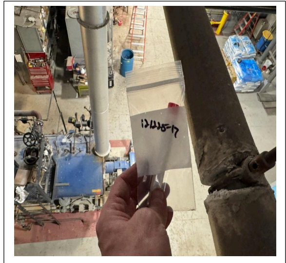
121225-17: TSI from white pipe directly above boiler number 3 positive for asbestos. (Believe new boiler will tie into this pipe).
