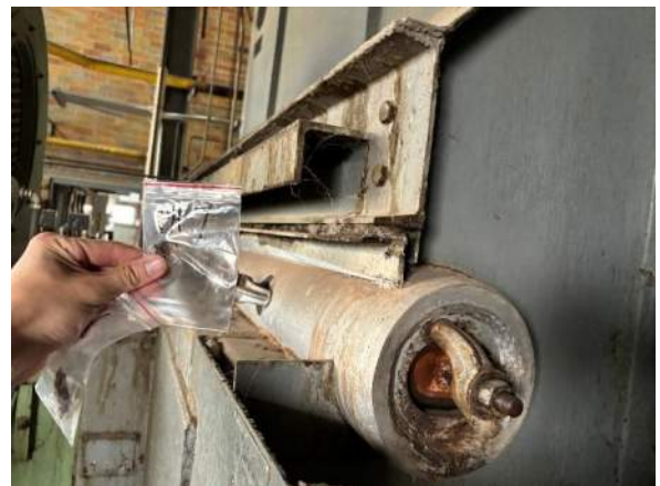
Photo #6 Sample PH-7. Asbestos containing boiler gasket on boilers #3 and #4.
