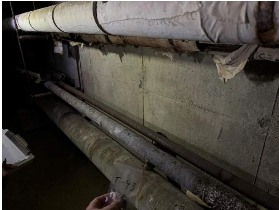
View of the Asbestos Containing Low Pressure Pipe in Birches Branch. (T-43, 26% Amosite & 10% Chrysotile)
