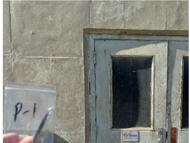
Photo #2 Sample P-1. Asbestos containing caulk around exterior doors.
