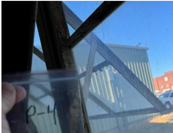
Photo #3 Sample P-4. Asbestos containing window glazing.
