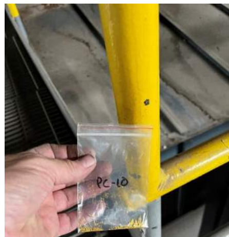
Photo #18 Sample PC-10. Yellow lead-based paint on handrail associated with boiler #2.
