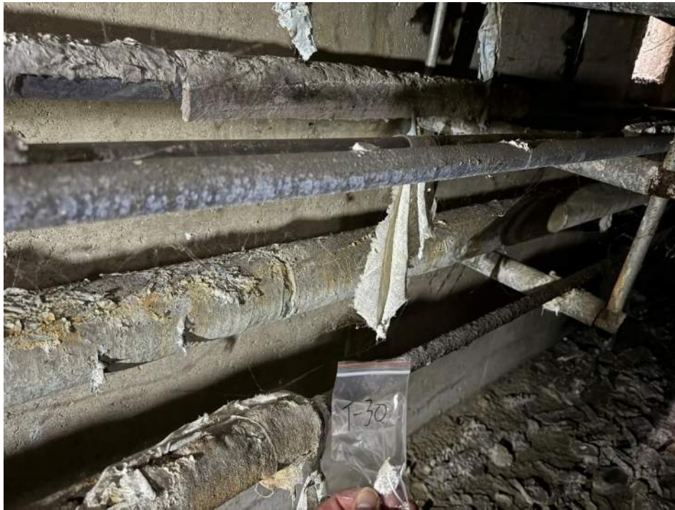
View of the Asbestos Containing 1” Pipe on Bottom Shelf in Maple Branch. (T-30, 33% Amosite & 20% Chrysotile)
