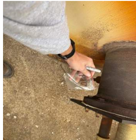
Photo #10 Sample PH-17. Asbestos containing rope gasket on fuel oil storage tank #3.
