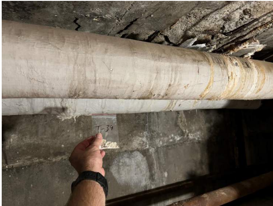
View of the Asbestos Containing Pipe Insulation. (T-39, 55% Chrysotile)
