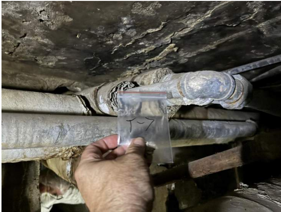
View of the Asbestos Containing TSI Airocell. (T-7, 17, 20, 32, 34, 35, 41, & 42, 40% - 80% Chrysotile)
