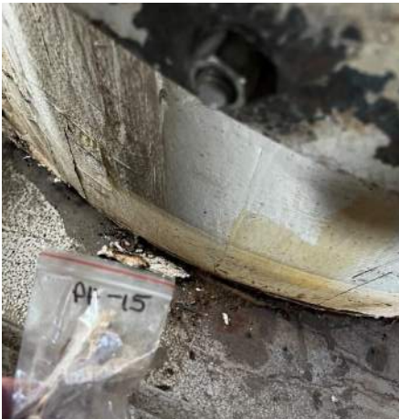
Photo #9 Sample PH-15. Asbestos containing white caulking on insulation located on the 2 nd floor mezzanine steam tank.
