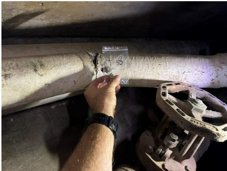
View of the Asbestos Containing Hot Water Pipe Elbow in Oak Hall Branch. (T-50, 65% Chrysotile)
