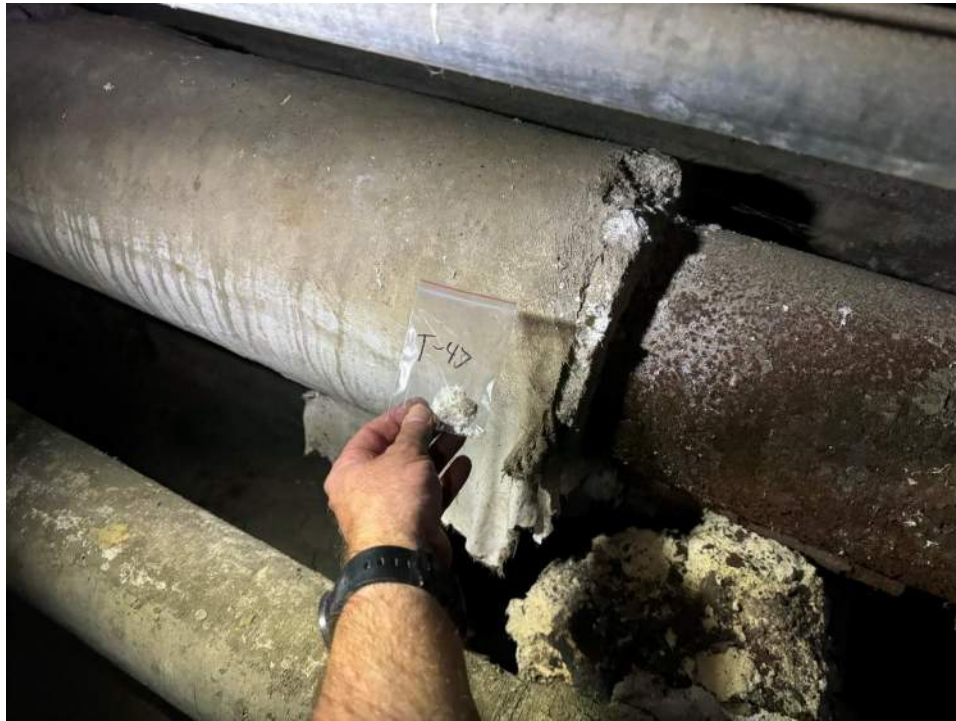
View of the Asbestos Containing Low Pressure Pipe in Oak Hall. (T-47 & 48, 25% Chrysotile, & 25% Chrysotile and 10 % Crocidolite)
