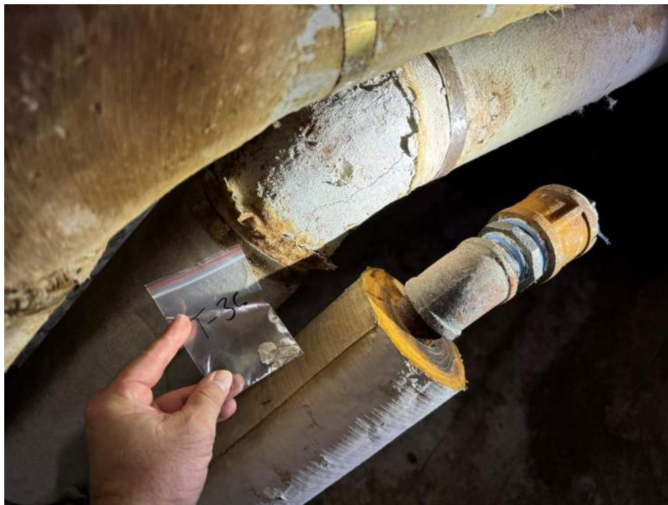
View of the Asbestos Containing Steam Pipe Elbow in Medical Branch. (T-36, 65% Chrysotile)
