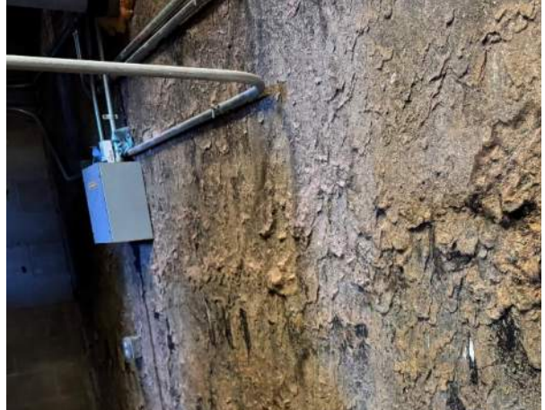
Photo #2 Sampe C-2. Asbestos containing black tar on diving wall.
