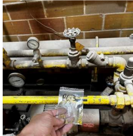
Photo #14 Sample PC-3. Yellow lead-based paint on metal fuel tank #4 piping.
