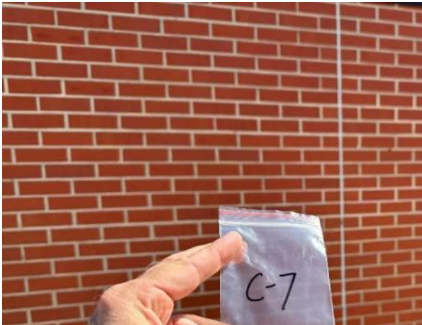
Photo #3 Sample C-7. Asbestos containing light grey expansion joint on exterior west side..
