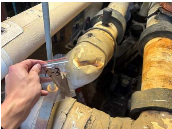
Photo #5 Sample C-3. Asbestos containing dark brown sealant on south side chilled water supply and return.
