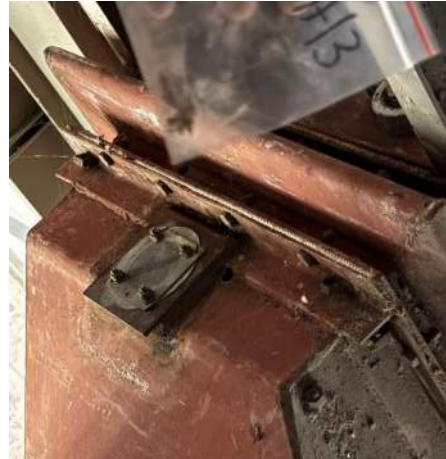
Photo #8 Sample PH-13. Asbestos containing red sealant on coal feeders in boiler rooms #3 and #4.
