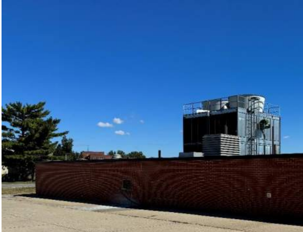
Photo #1 View of the Chiller.
