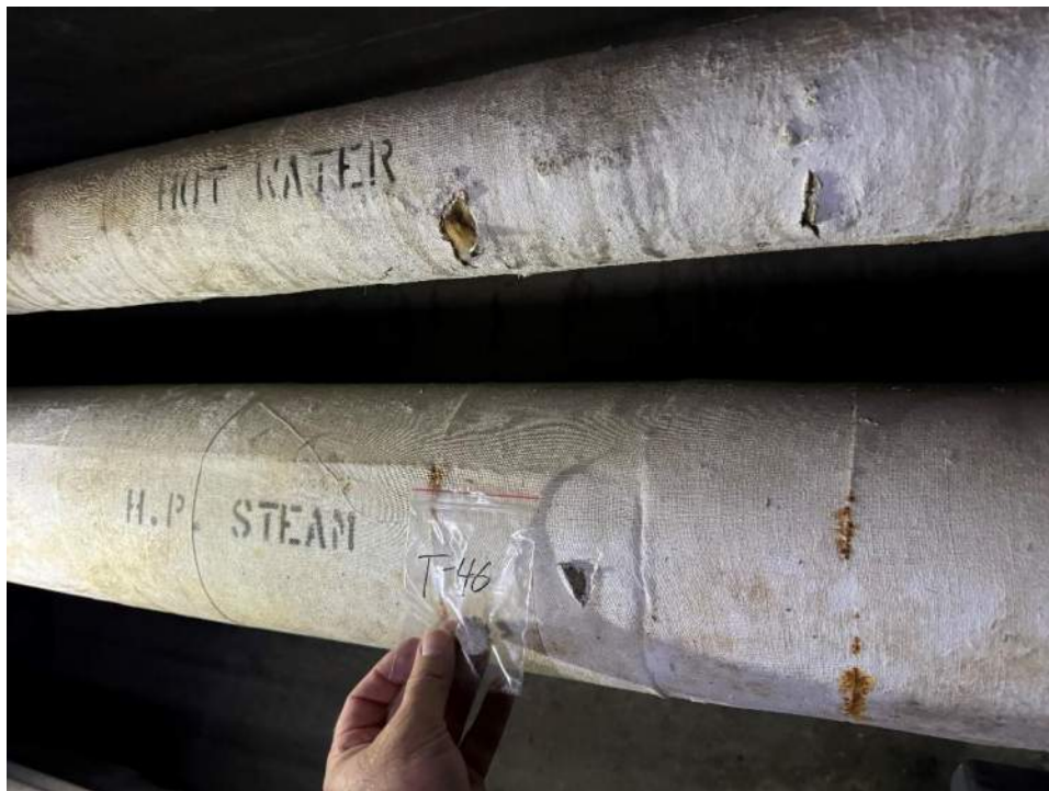
View of the Asbestos Containing High Pressure Pipe in Oak Hall Branch. (T-46 & 49, 30% Amosite & 15% Chrysotile, & 60% Chrysotile)
