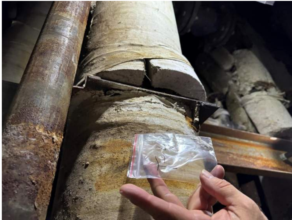
View of the Asbestos Containing High Pressure TSI. (T-4, 70% Chrysotile)
