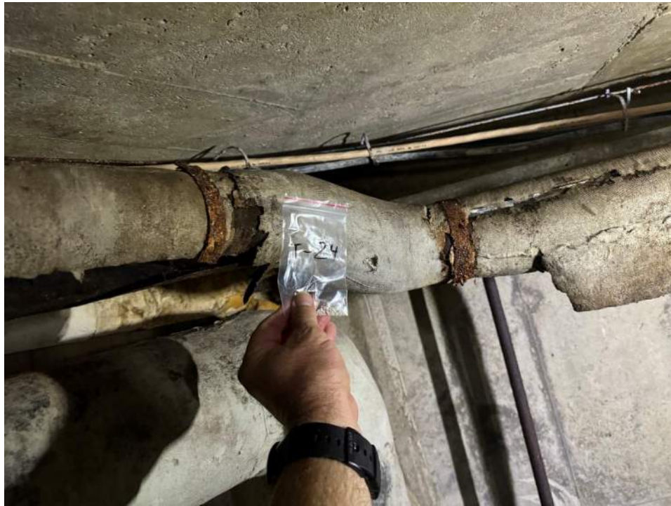
View of the Asbestos Containing 2" Elbow. (T-24, 7% Amosite & 55% Chrysotile)
