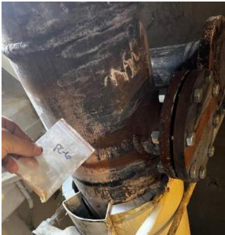
Photo #15 Sample PC-6. Pink lead-based paint on steam piping on future turbine room on ground floor.
