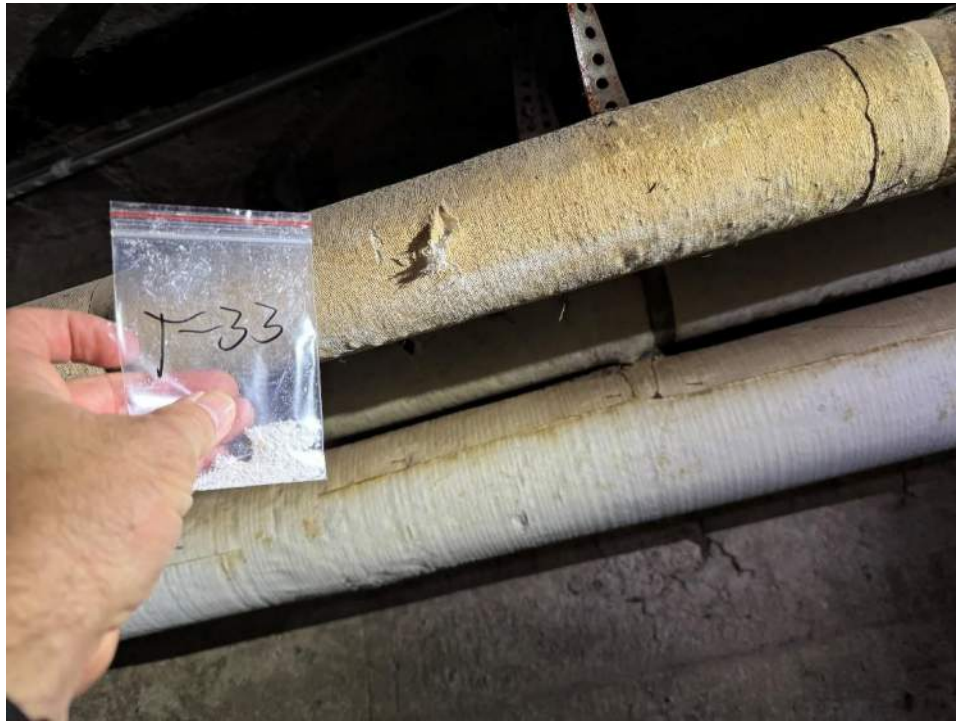
View of the Asbestos Containing 2" Pipe Run in Medical Branch. (T-33, 38% Chrysotile)
