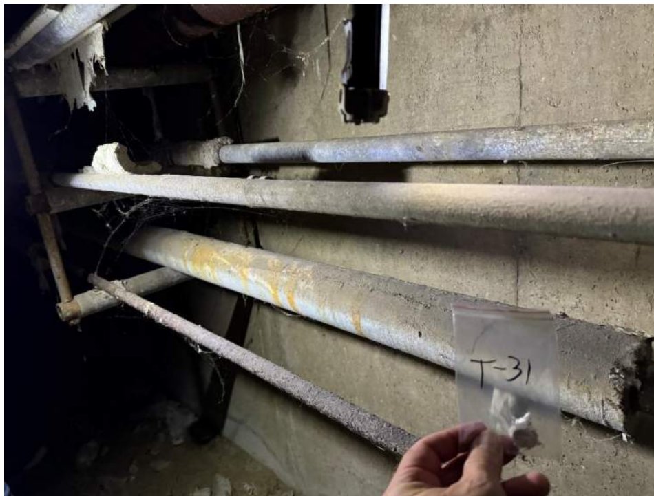
View of the Asbestos Containing 2” Pipe on Bottom Shelf in Maple Branch. (T-31, 33% Amosite & 20% Chrysotile)
