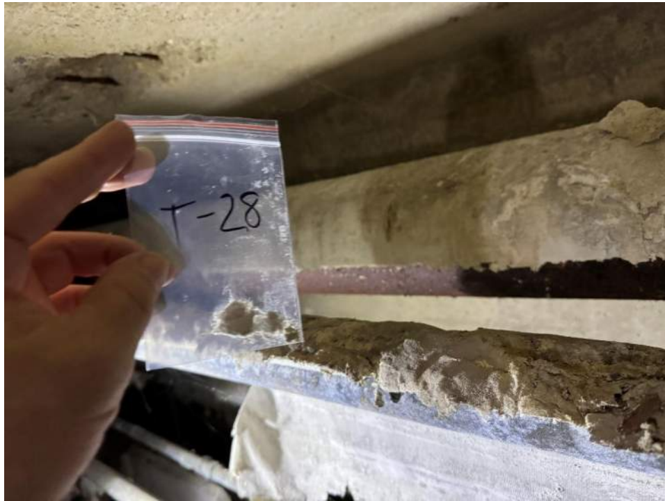
View of the Asbestos Containing High Pressure Pipe in Maple Branch. (T-28, 15% Amosite & 20% Chrysotile)
