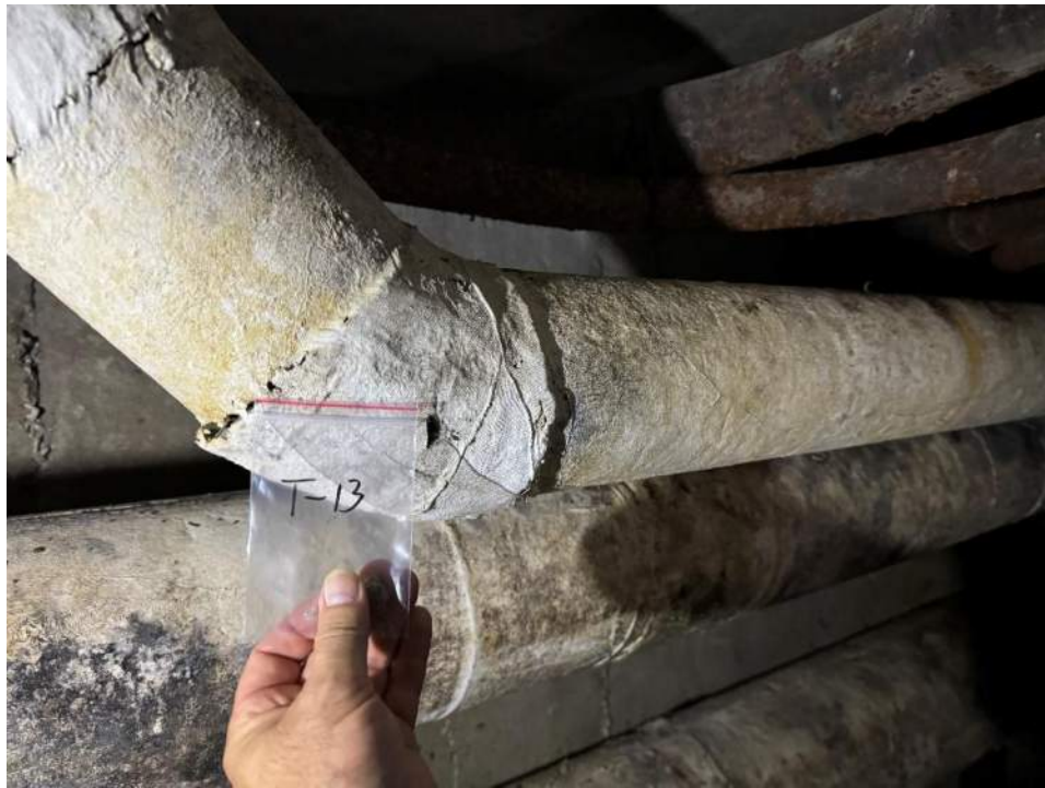
View of the Asbestos Containing Hot Water Elbows. (T-13, 14, 15, & 19, 60% - 65% Chrysotile)
