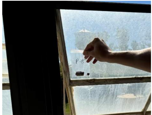
Photo #4 Sample P-8. Asbestos containing window glazing.
