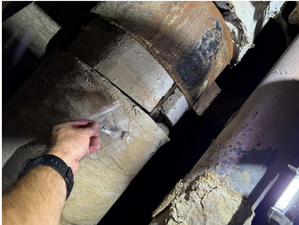
View of the Asbestos Containing Low Pressure Pipe. (T-1, 2, & 3, 40% - 65% Chrysotile)
