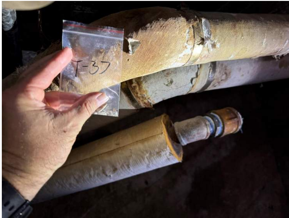
View of the Asbestos Containing Middle Pipe Elbow in Medical Branch. (T-37, 12% Chrysotile)
