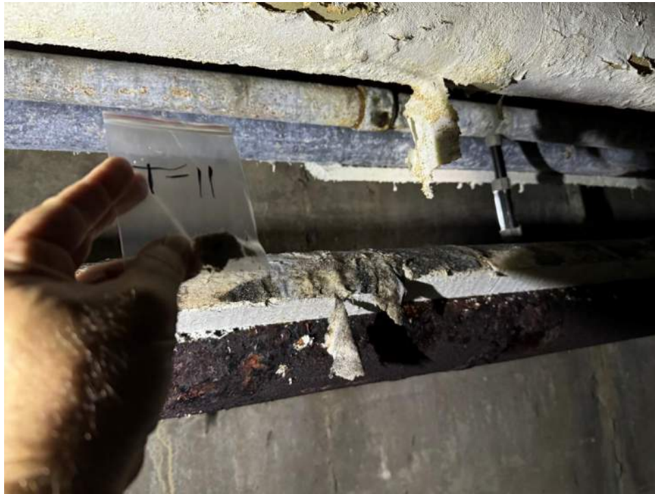
View of the Asbestos Containing Pipe (above Hot Water at Orchard and Cedar Intersection). (T-11, 40% Chrysotile)
