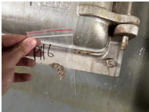
Photo #5 Sample PH-6. Asbestos containing boiler door gasket on boilers #3 and #4
