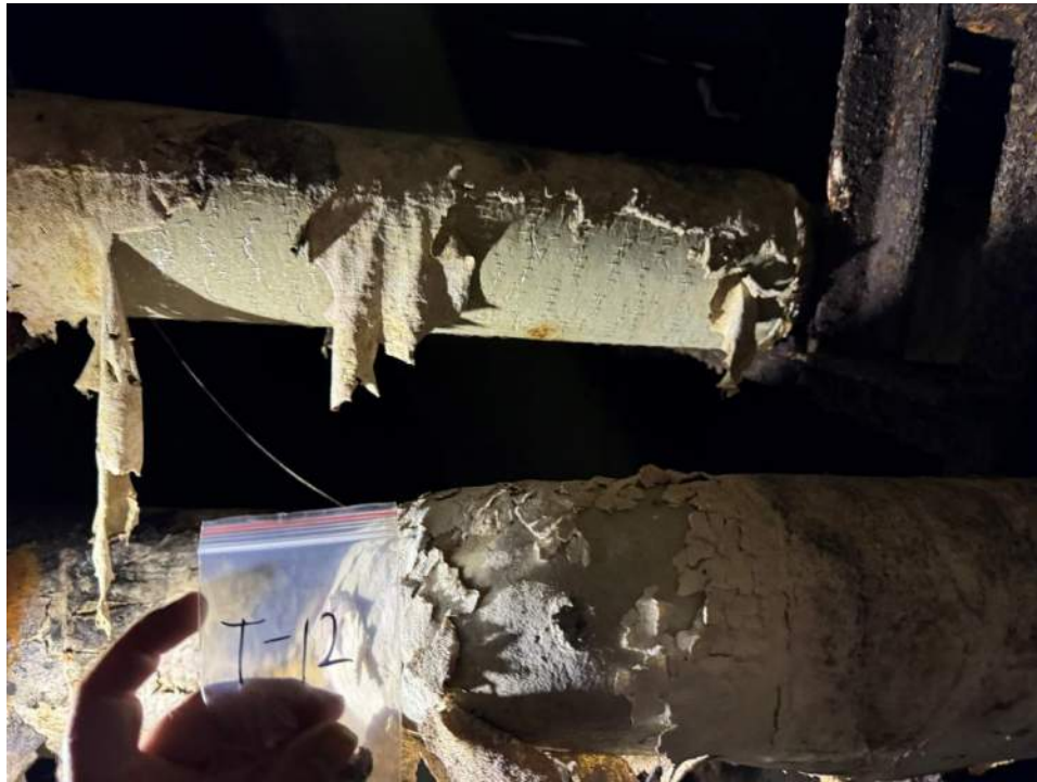
View of the Asbestos Containing High Pressure Elbow. (T-12 & 18, 65% & 70% Chrysotile)
