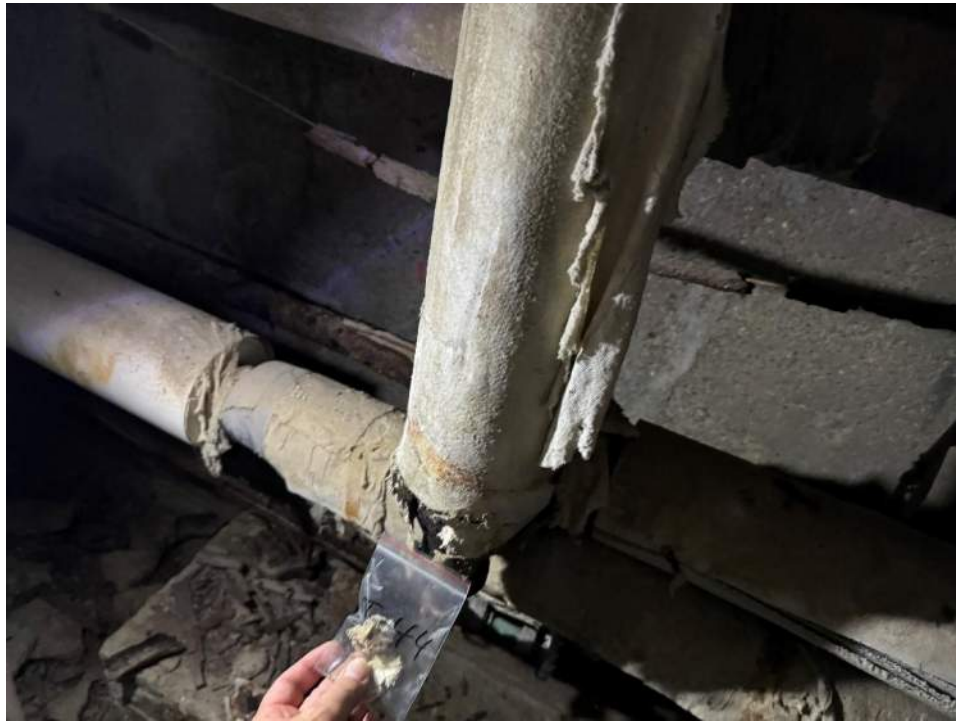
View of the Asbestos Containing High Pressure Pipe Elbow. (T-44, 60% Chrysotile)
