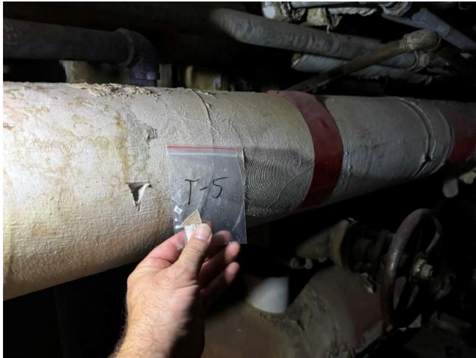
View of the Asbestos Containing High Pressure Pipe. (T-5, & 6, 22% - 28% Amosite & 7% - 10% Chrysotile)
