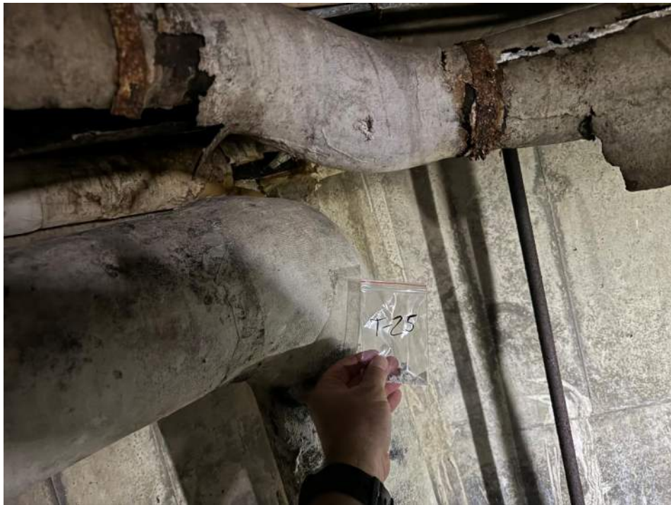
View of the Asbestos Containing 4" Elbow. (T-25, 60% Chrysotile)
