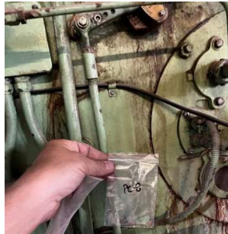
Photo #16 Sample PC-8. Green lead-based paint on metal burn chamber of boiler #1.
