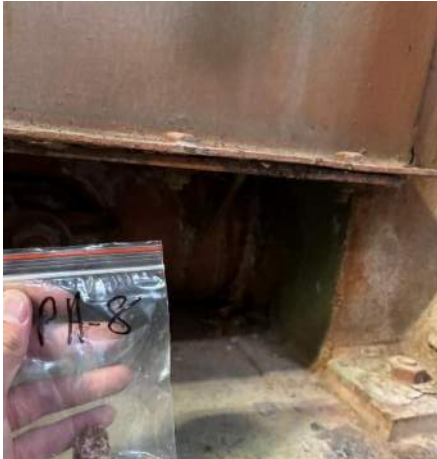
Photo #7 Sample PH-8. Asbestos containing grey boiler sealant on boilers #3 and #4.
