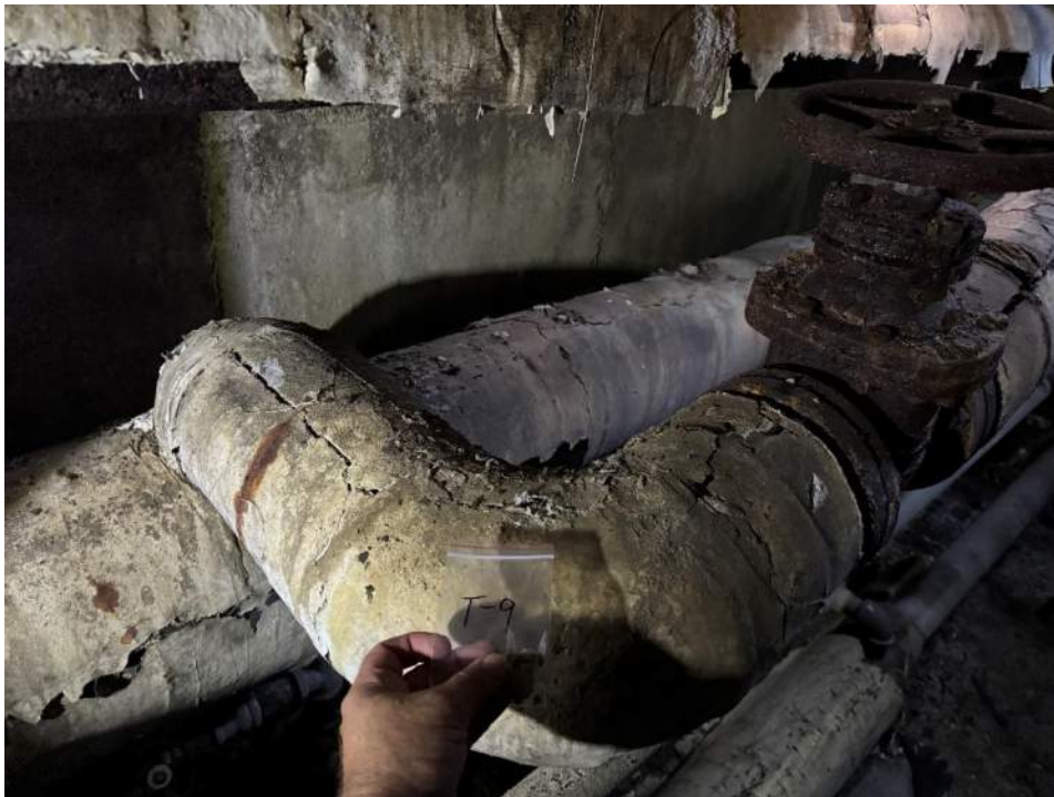
View of the Asbestos Containing High Pressure TSI Elbow. (T-8, 9, & 10, 60% - 70% Chrysotile)
