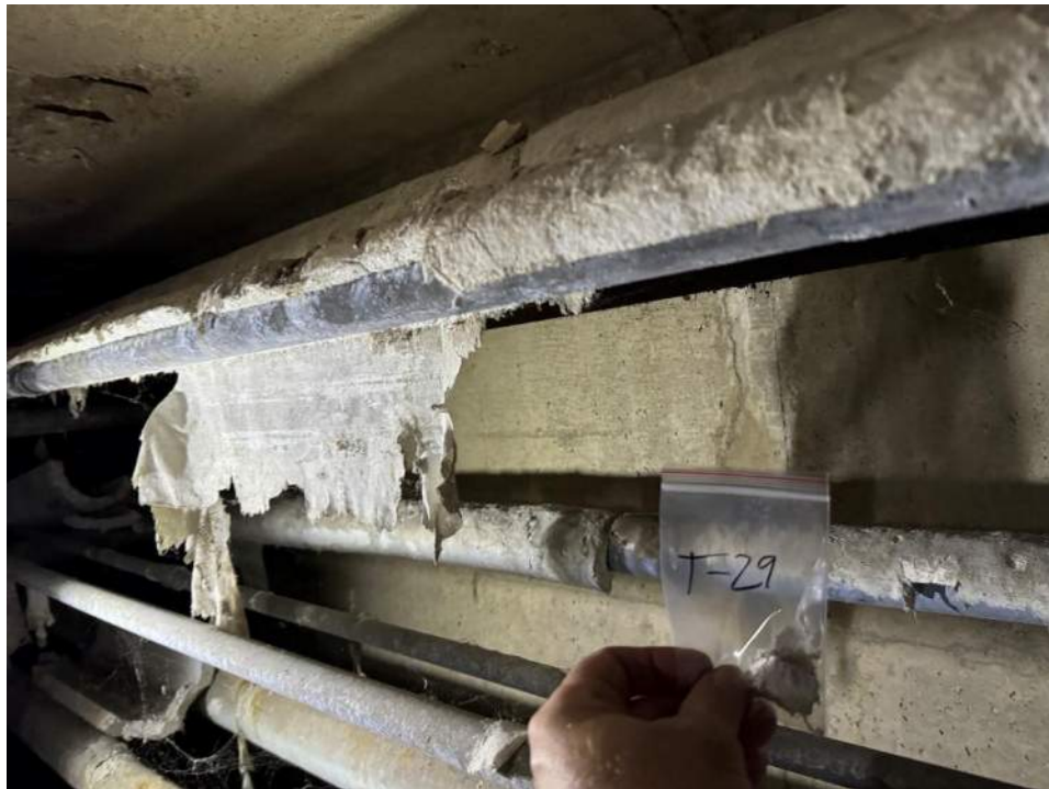
View of the Asbestos Containing 2" Pipe on Middle Shelf in Maple Branch. (T-29, 30% Amosite & 20% Chrysotile)
