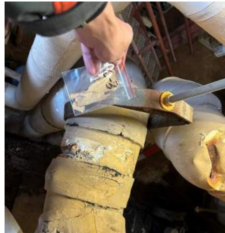
Photo #4 Sample C-3. Asbestos containing dark brown sealant on south side chilled water supply and return.
