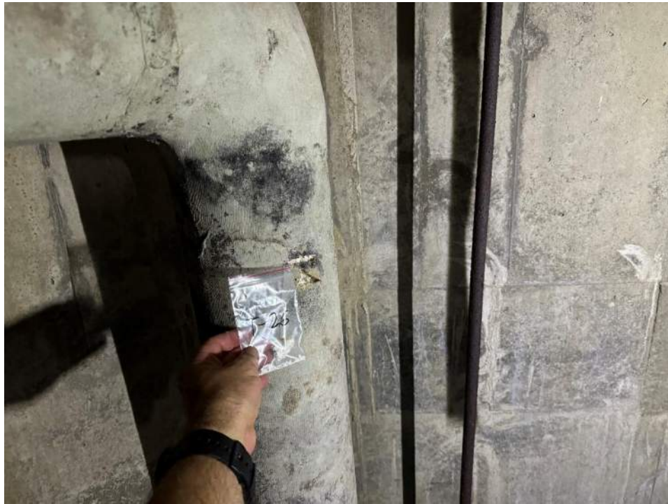
View of the Asbestos Containing 4" Pipe Run in E Home Branch. (T-26, 22% Amosite & 7% Chrysotile)
