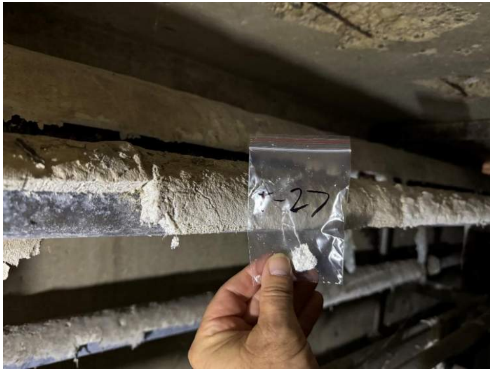
View of the Asbestos Containing 2" Pipe Run in Maple Branch. (T-27, 10% Amosite & 17% Chrysotile)
