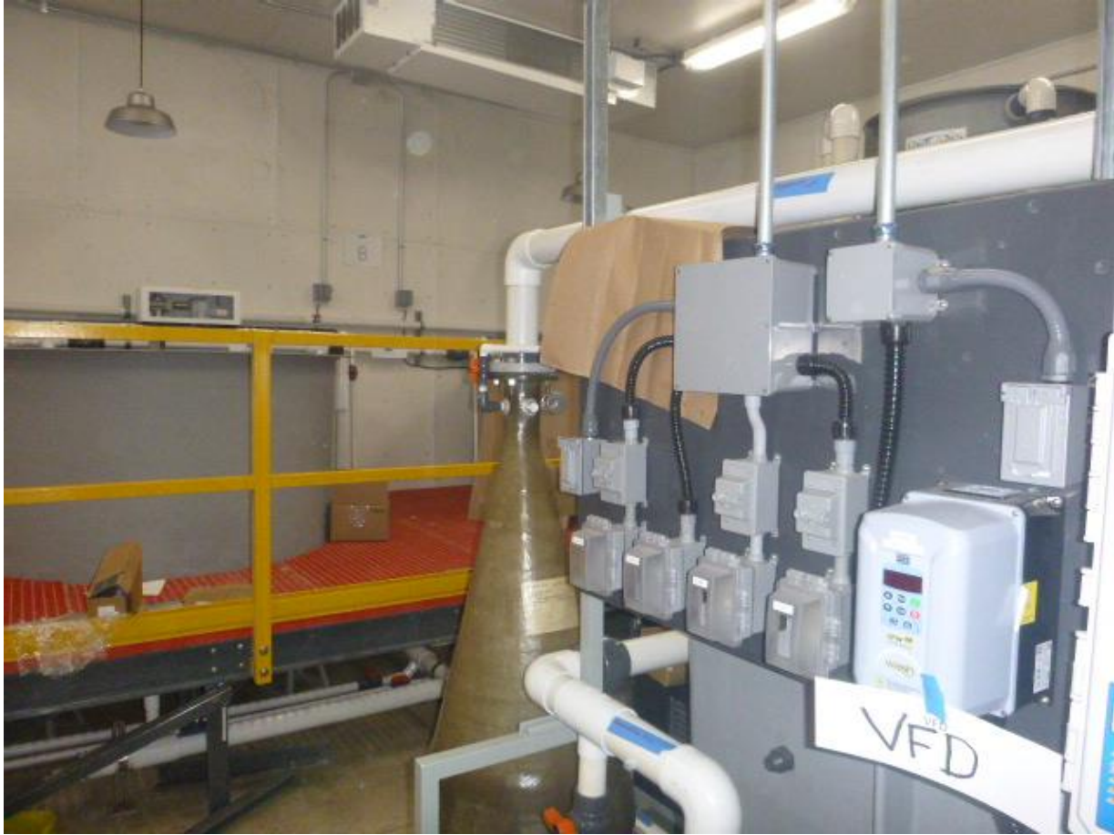
Photo 4: VFD location in relation to Panel B.
