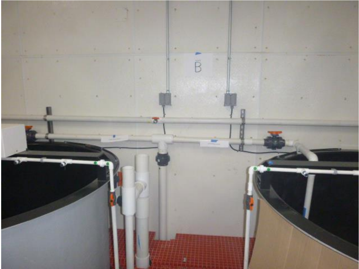
Photo 3: Panel B and 2" pipe flow meter mounting locations.
