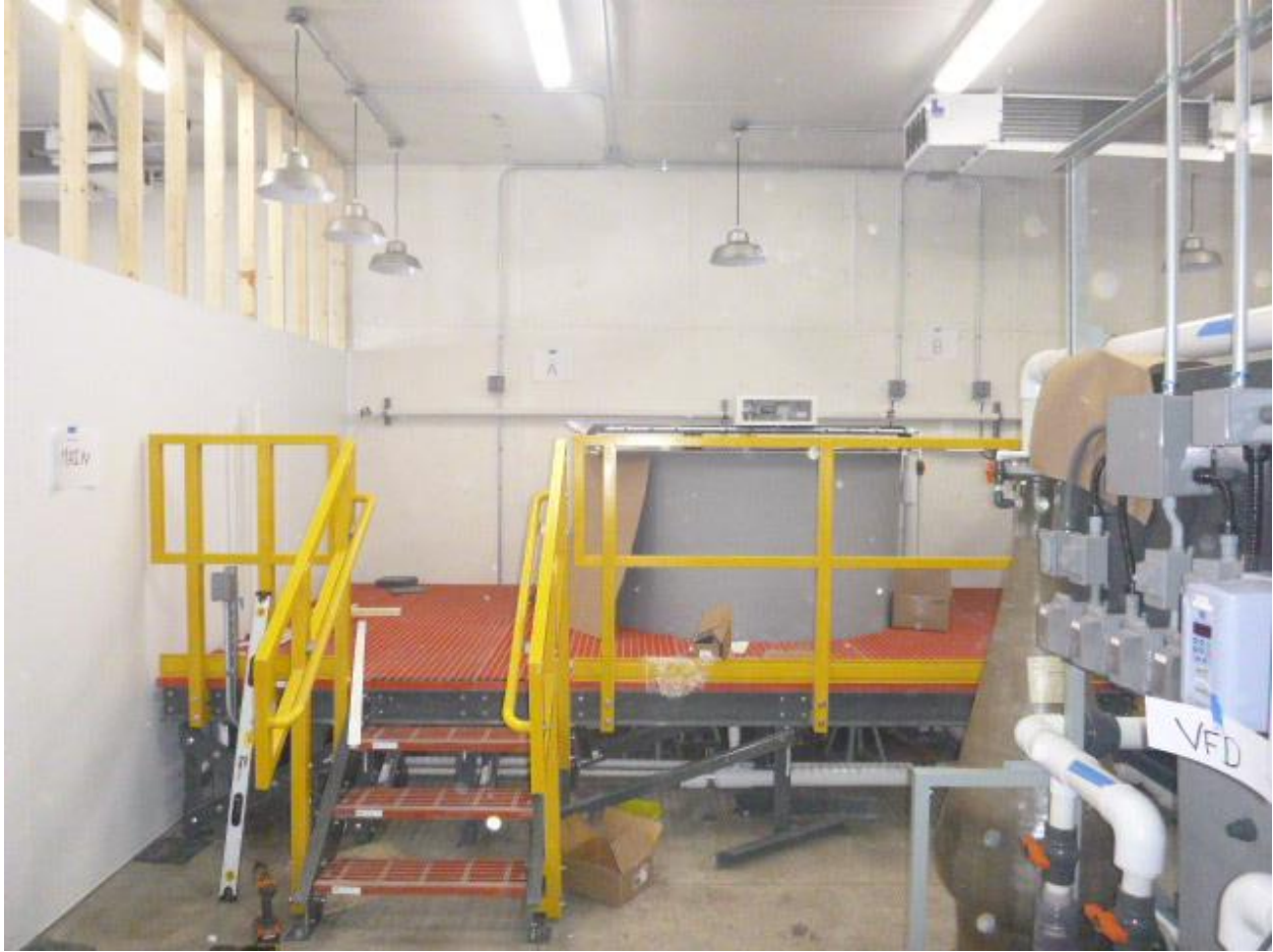
Photo 1: Overview of panel and VFD locations.
