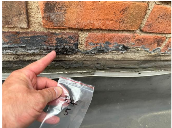
Photo #4 Asbestos containing black tar / sealant on SW wall of roof.
