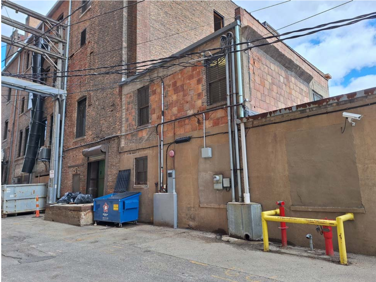
ALLEY - POWER LINES & SPRINKLER PIPES
