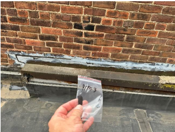
Photo #3 Asbestos containing black tar / sealant on south wall of roof.
