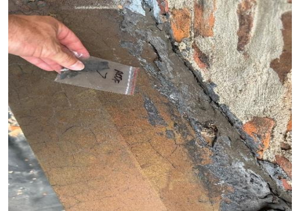
Photo #6 Asbestos containing black tar / sealant on NW wall of roof.
