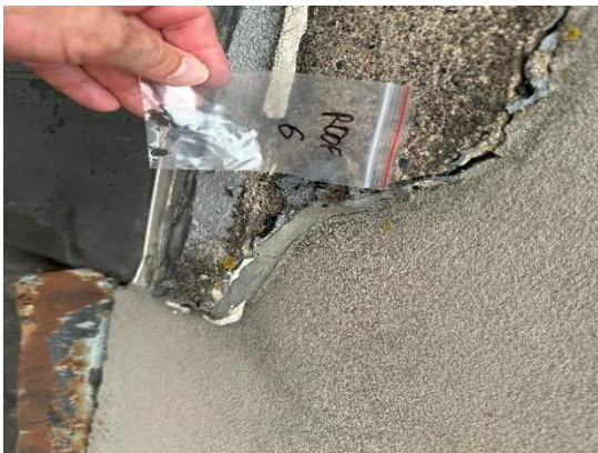
Photo #5 Asbestos containing black tar / sealant on SE wall of roof.
