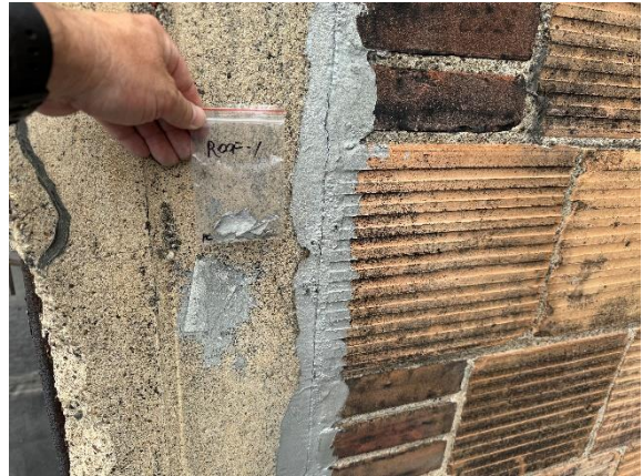
Photo #2 Asbestos containing white caulk on SE corner of roof.
