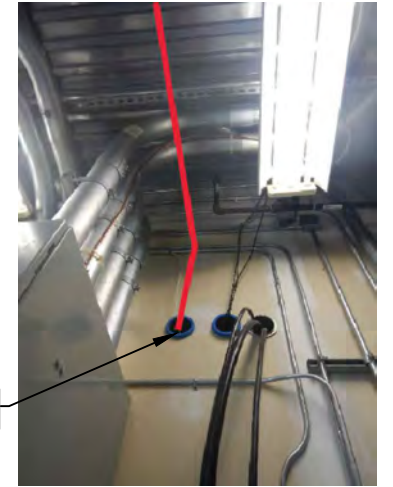
ELECTRICAL ROOM - LOOKING WEST
