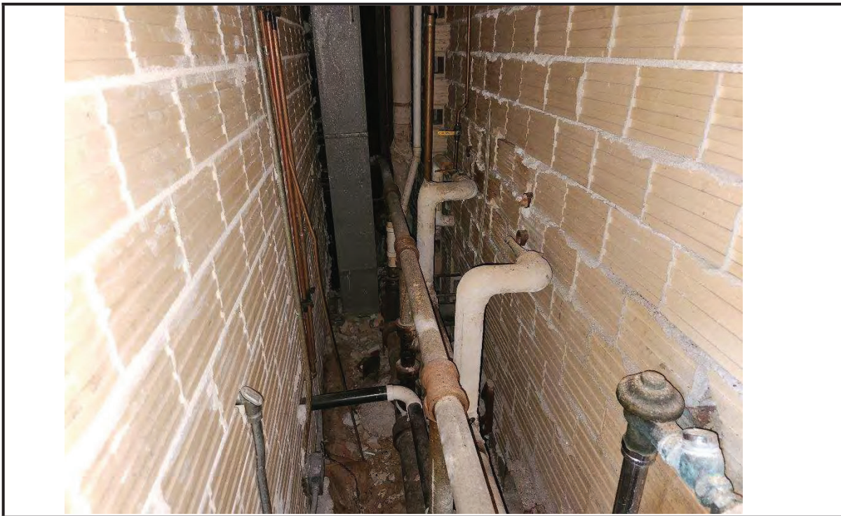
Photo 2: View of mudded joint fittings in a pipe chase in Basement Area B.
