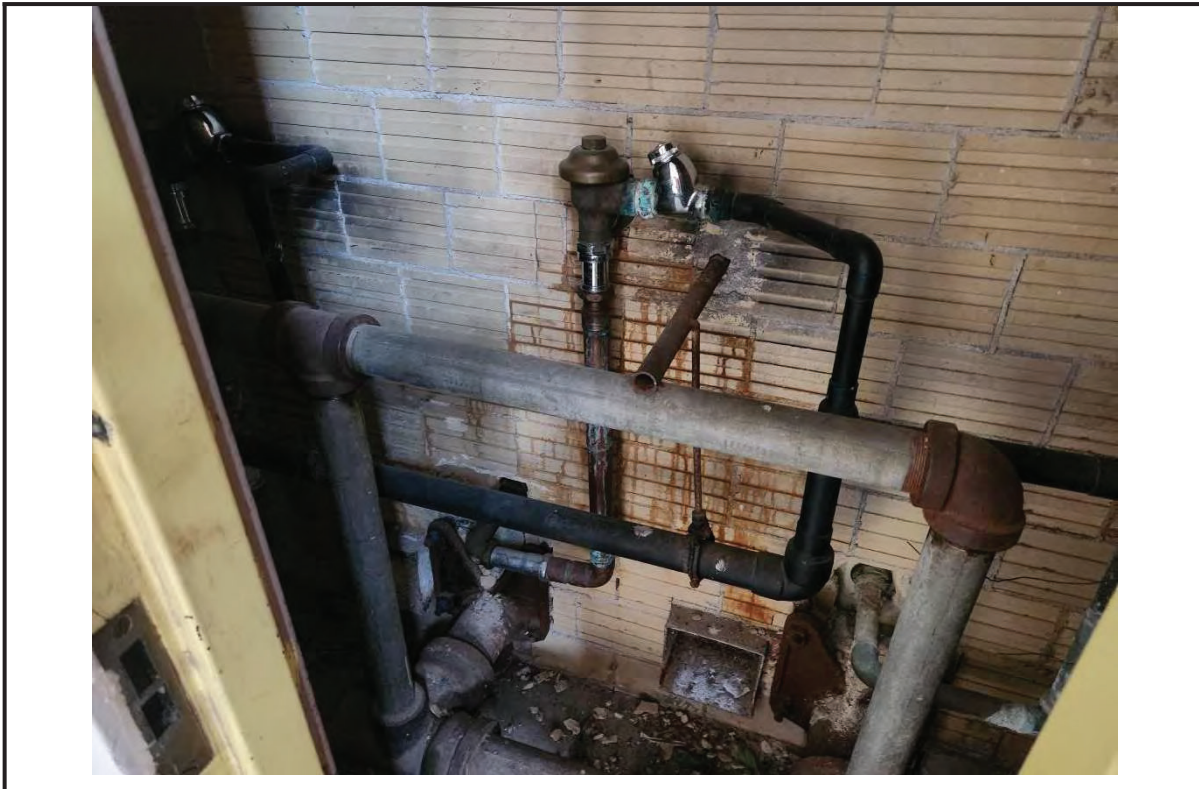
Photo 5: View of a typical plumbing closet (no pipe insulation present).
