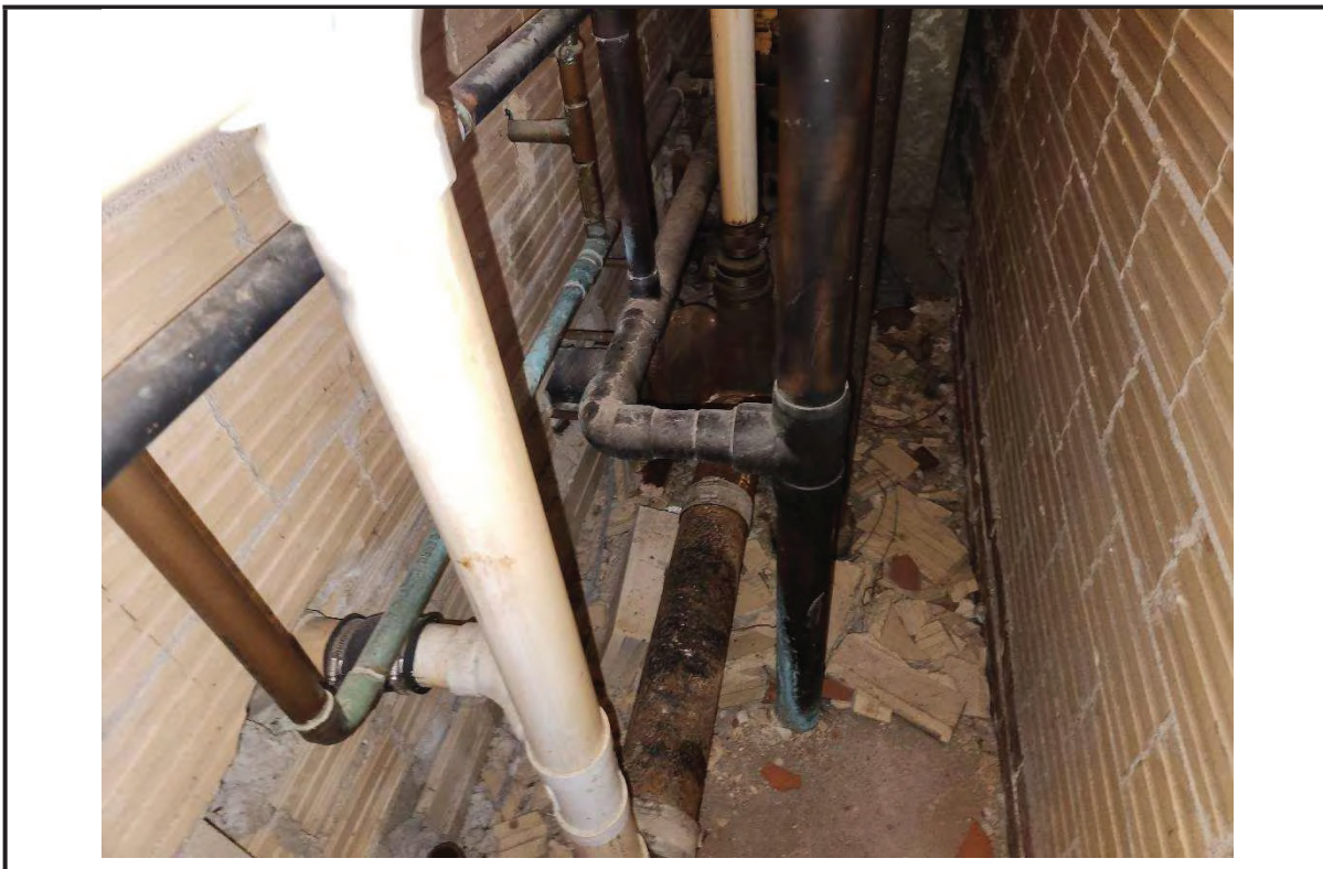
Photo 16: View of a typical pipe chase closet with cast iron, copper, and PVC piping (no ACM present).
