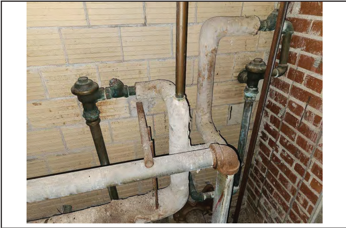
Photo 9: View of pipe insulation and muddled fittings in a pipe chase.
