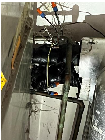
Photo #5 Assumed asbestos containing Black Tar Pipe Wrap – at AHU in Stair Landings of House A & B
