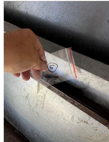
Photo #4 Sample #6 – Black Sealant at Metal Pad of AHU – House A Stair Landing
