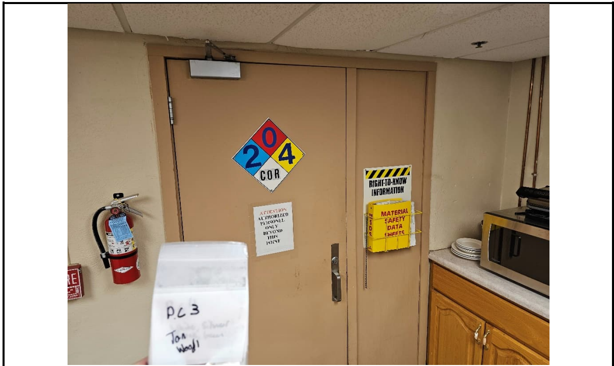
Photo 7: PC 3: lead-containing tan paint on a door and associated components.
