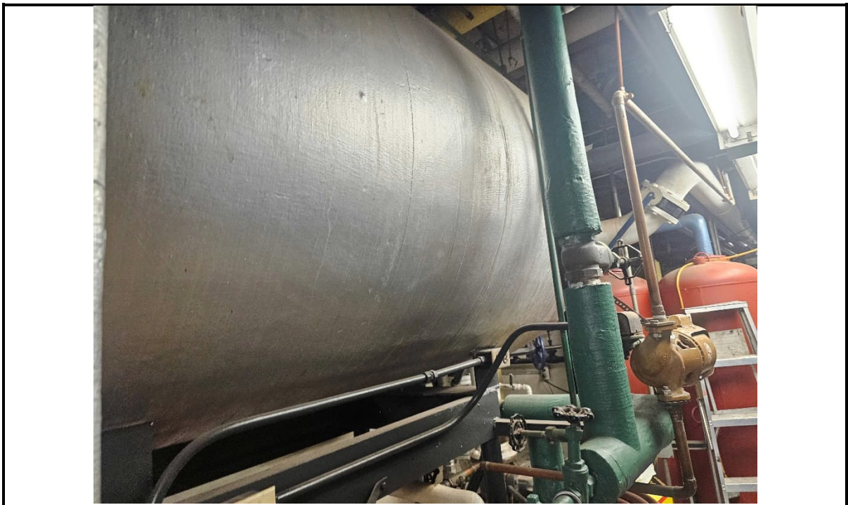
Photo 6: View of the ACM mud associated with the hot water heater tank.
