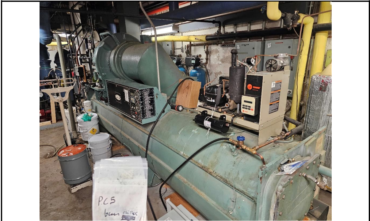
Photo 9: PC 5: lead-containing green paint on the chiller.
