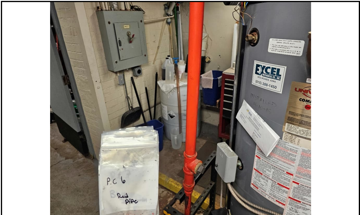
Photo 10: PC 6: lead-containing red paint on a pipe.
