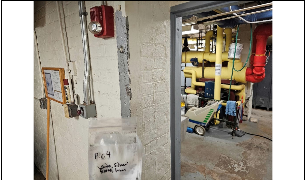
Photo 8: PC 4: lead-containing white and silver paint on walls and frames in the basement.
