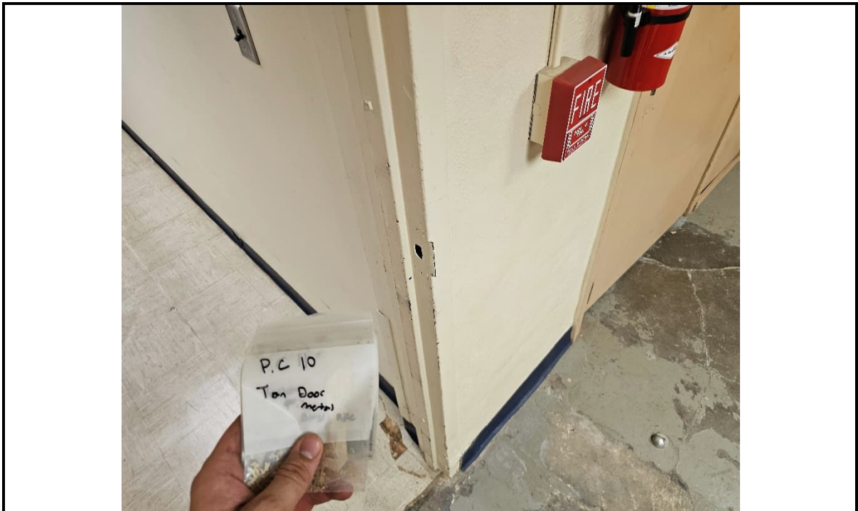
Photo 12: PC 10: lead-containing paint on a tan door.
