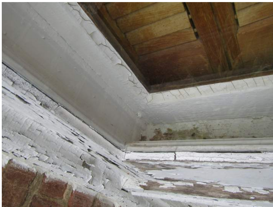
LOWER WINDOW GLAZING AND CHIPPING PAINT
