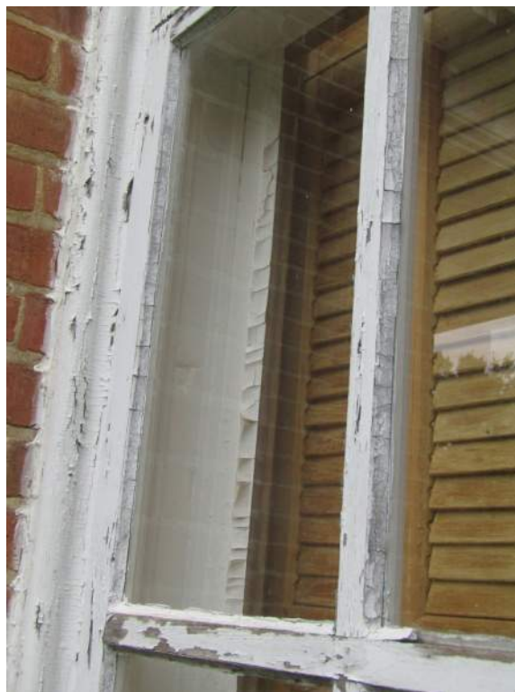
UPPER WINDOW GLAZING AND CHIPPING PAINT
