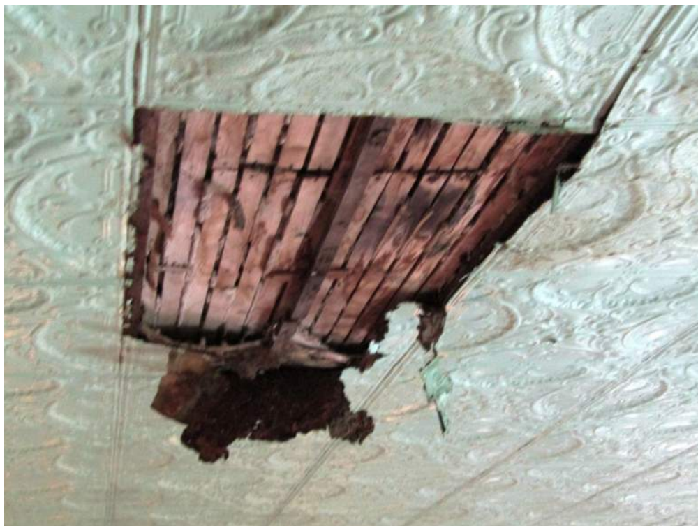
MISSING CEILING TILE INSIDE CHURCH
