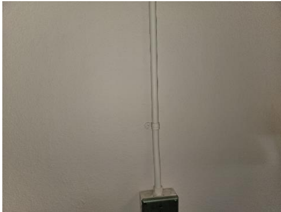
View of white paint on plaster wall in N stairway. (17.9 mg/cm 2 )
