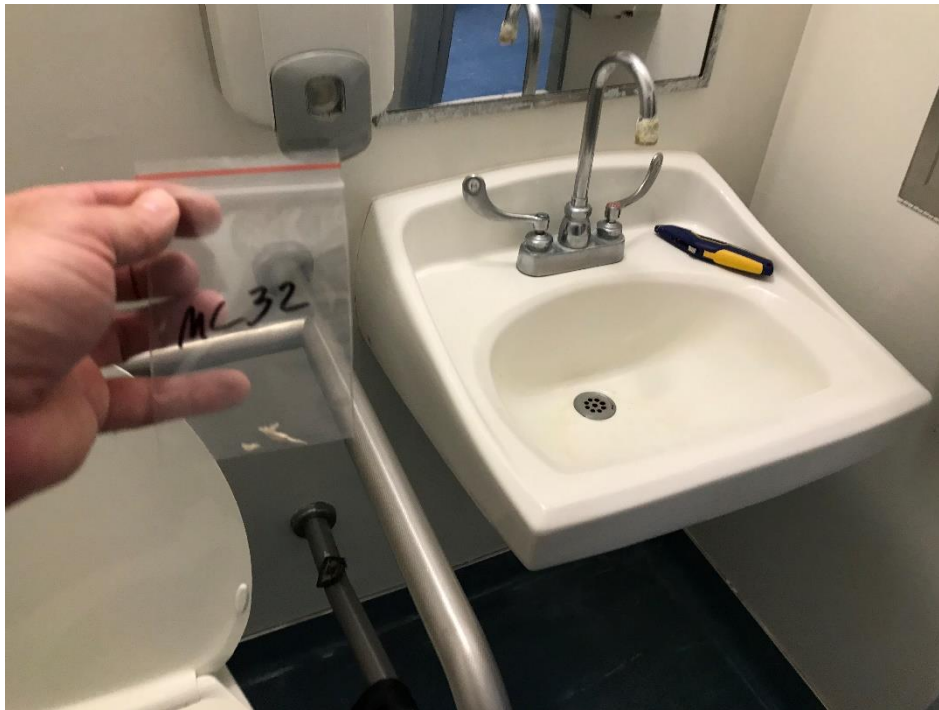
View of the Asbestos Containing White Caulk. (South Wing, MC 32, <1% Chrysotile)
