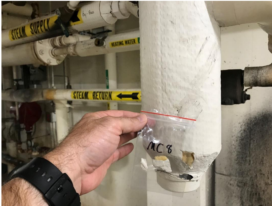
View of the Asbestos Containing TSI Run (Mastic/Sealant). (South Wing, MC 8, 4% Chrysotile)
