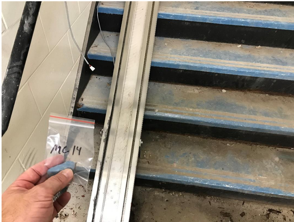
View of the Asbestos Containing Blue Vinyl Flooring on Stairs. (South Wing, MC 14, 3% Chrysotile)
