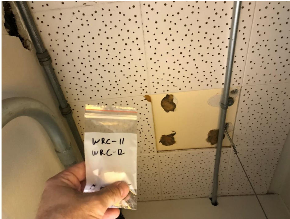
View of Brown Ceiling Pucks on 1 st Floor (WRC-12, 3% Chrysotile)
