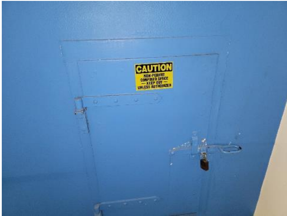
View of blue paint on metal attic access door. (1.0 mg/cm 2 )
