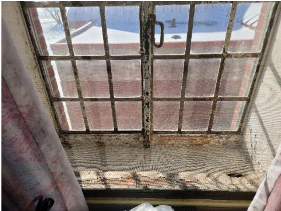
View of white paint on window frame and trough. (2.0 and 5.9 mg/cm 2 )
