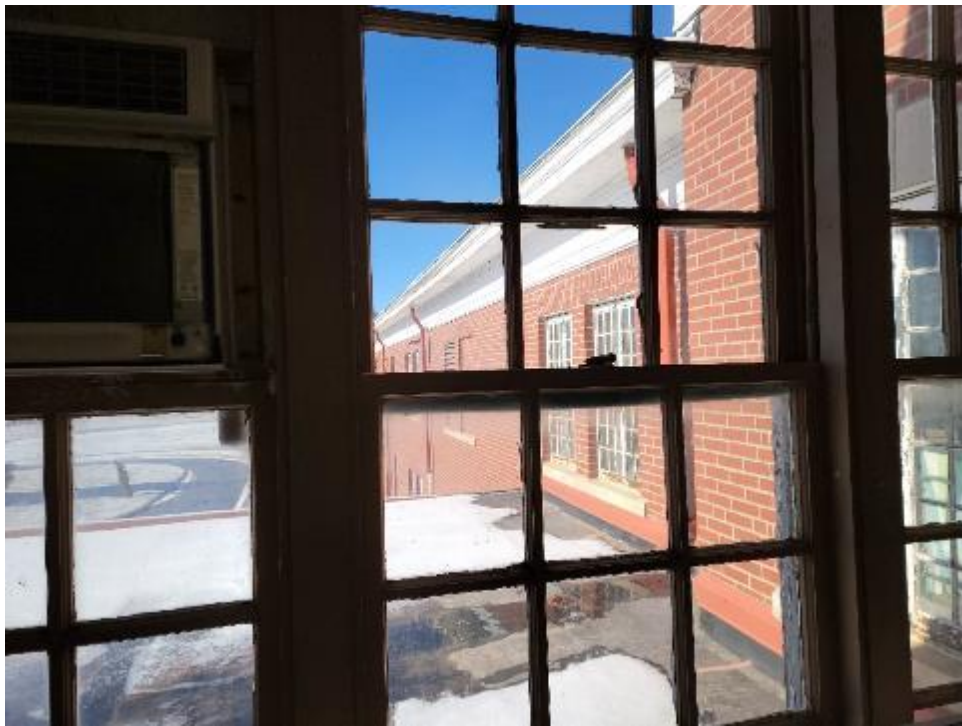
View of very light tan paint on the window frames (1.9 mg/cm 2 )
