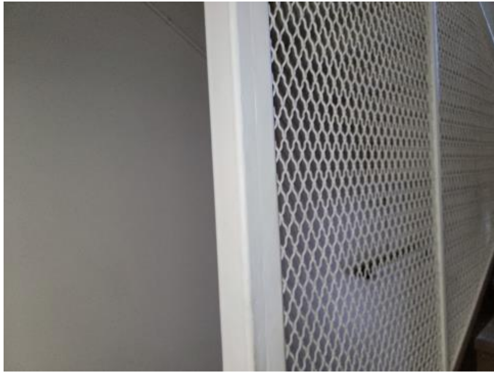
View of white paint on stair post and cage. (9.6 mg/cm 2 )
