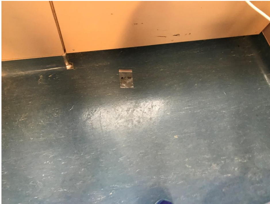
View of the Asbestos Containing Blue Vinyl Flooring. (South Wing, MC 30, 2% Chrysotile)
