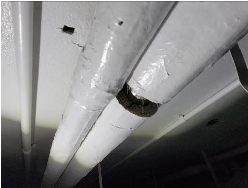
View of TSI Aerocell (40-65% Chrysotile)
