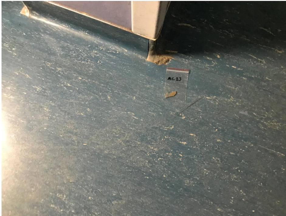
View of the Asbestos Containing Blue Vinyl Flooring. (South Wing, MC 23, 3% Chrysotile)
