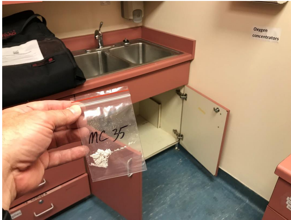
View of the Asbestos Containing White Sink Insulation. (South Wing, MC 35, 8% Chrysotile)
