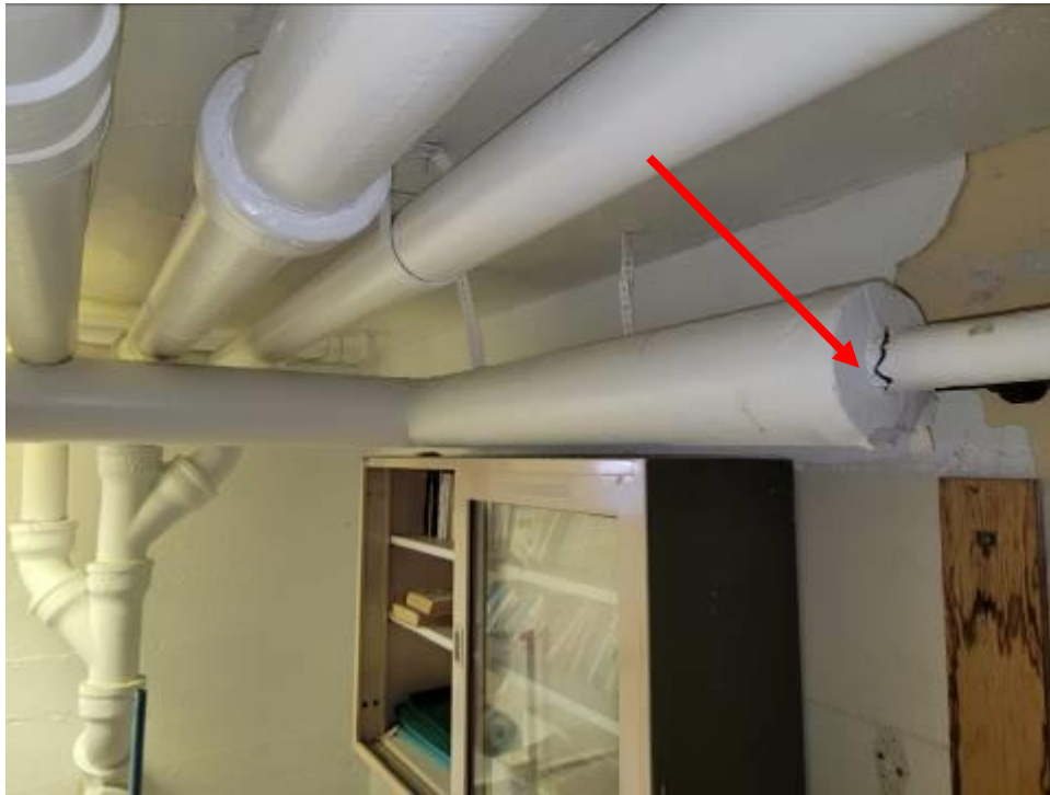
View of TSI 2" Pipe (10-20% Amosite 5% Chrysotile)
