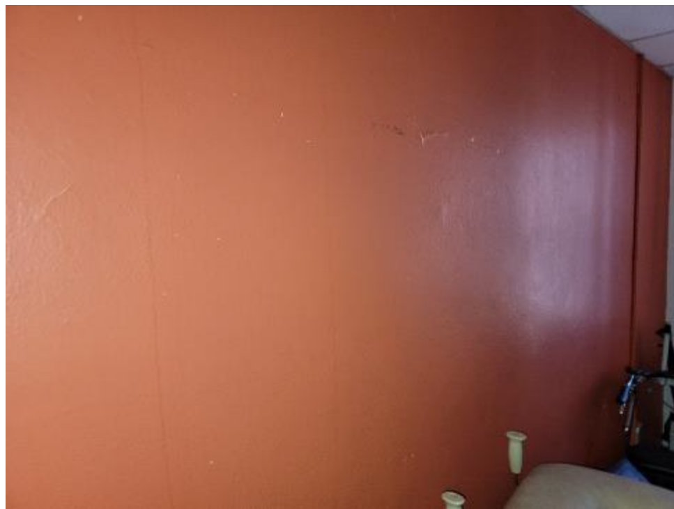
View of pink over orange paint on the plaster walls. (17.3 mg/cm 2 )
