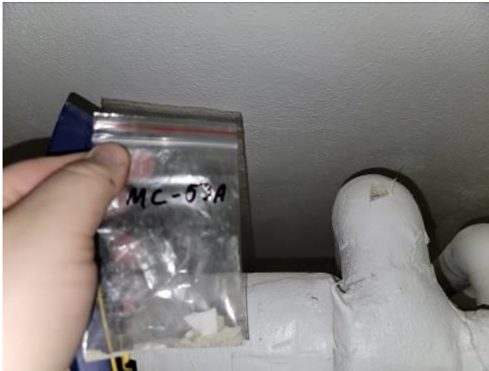
View of TSI 1" Elbow (2% Chrysotile)
