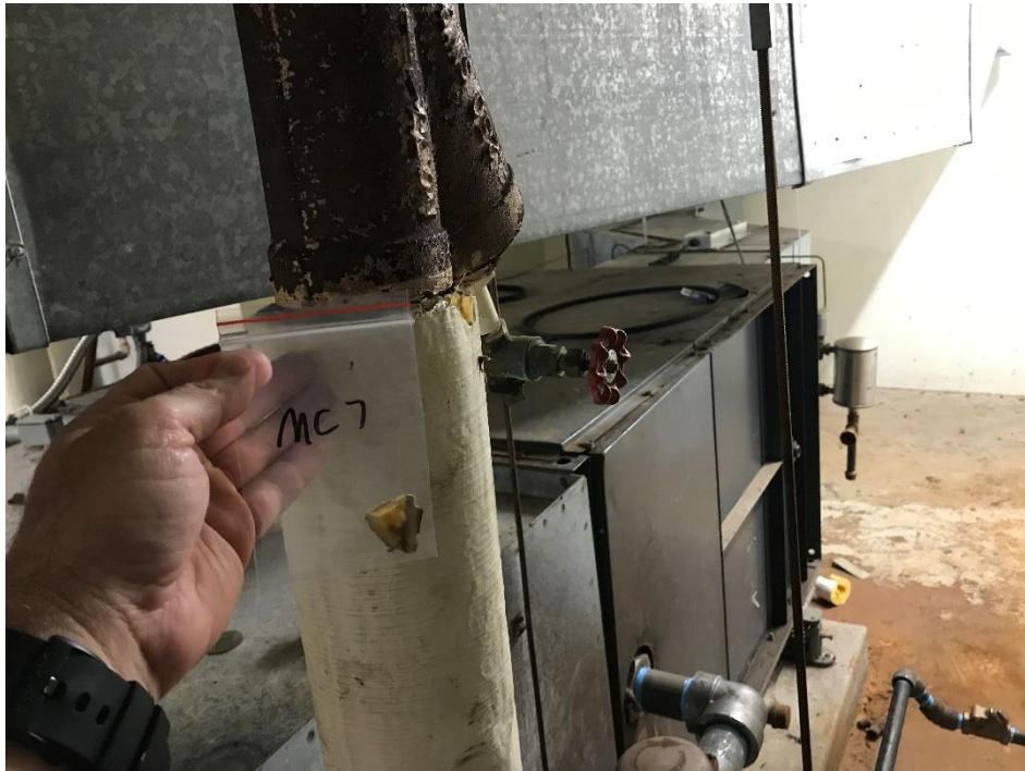
View of the Asbestos Containing TSI Run (Mastic/Sealant). (South Wing, MC 7, 4% Chrysotile)
