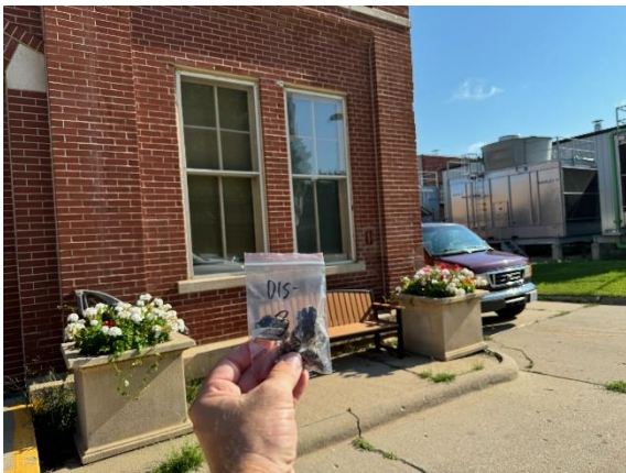
Photo #3 Another photo of window caulking. (DIS-3, 20-35% Chrysotile)
