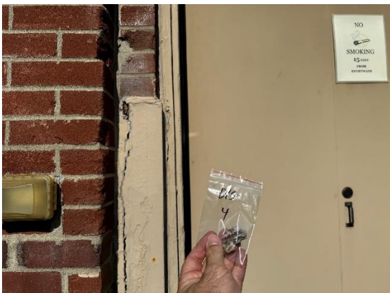
Photo #5 Another photo of doorframe caulking. (DIS-4, 15% Chrysotile)
