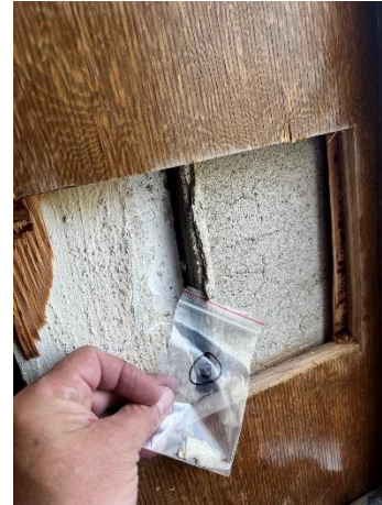
Photo #2 Sample #3 – Old white sealant. At NW window in Room ED3-18.
