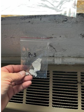
Photo #7 Paint Sample PC-3 – Wall under window Room ED3-14.
