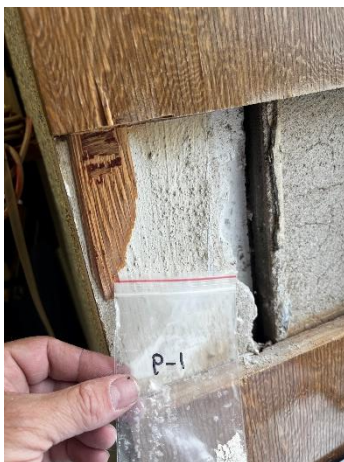
Photo #5 Paint Sample PC-1 – Cream paint on old plaster wall at NW window in Room ED3-18.
