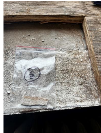
Photo #4 Sample #6. Plaster on window sill. Room ED3-18.
