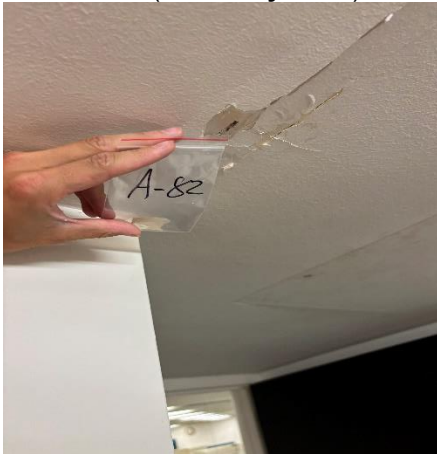
Photo # 3 A-82 Room 1111 Ceiling, 1 st Floor, White Drywall Tape ( 3% Chrysotile ).
