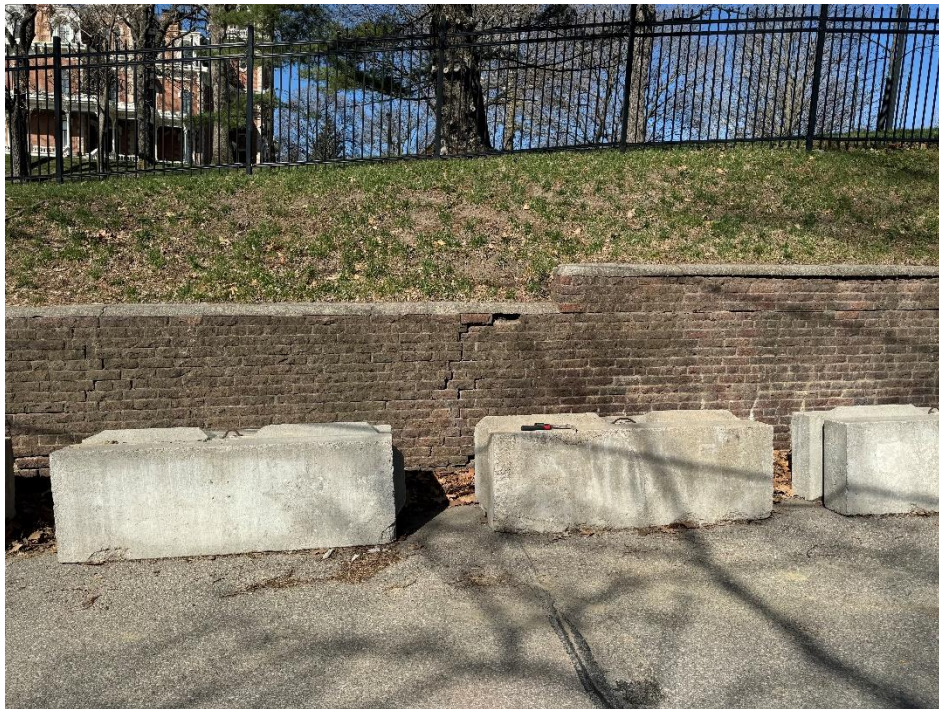
View of the retaining wall where most of the damage is, and samples were taken
