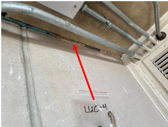
Photo #3 View of Brittle Asbestos Containing Caulk above Loading Dock Doors.
