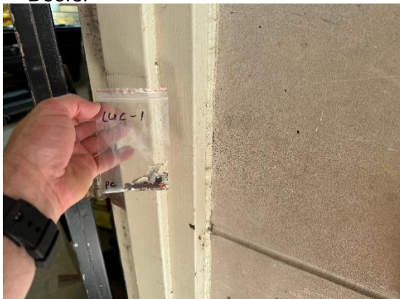
Photo #5 View of Off-white LBP on Loading Dock Doorframe.
