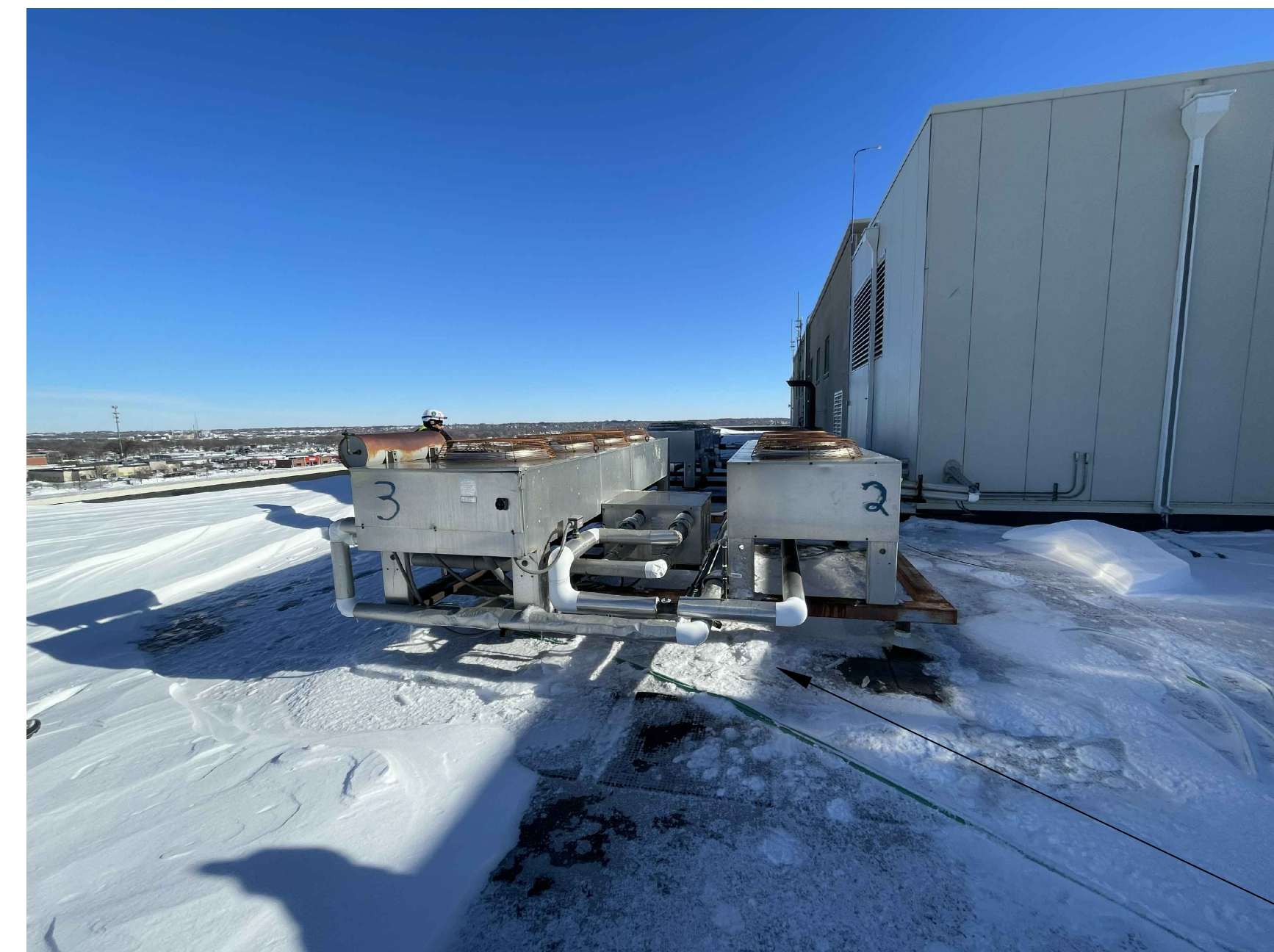
3 PICTURE OF EXISTING DRYCOOLERS
