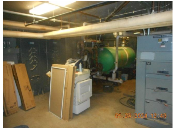
Photo #2 Asbestos Containing Tank Insulation – Wing 61 – Mech Room 108
