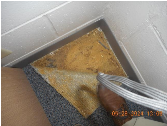
Photo #3 Asbestos containing mastic remnants under carpet – Wing 61 – Room 215.
