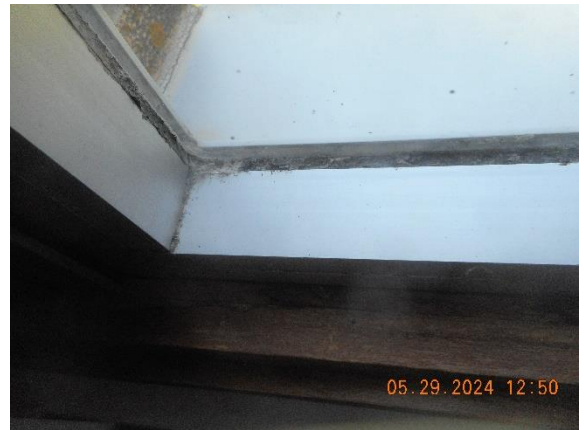
Photo #4 Asbestos window glazing on inoperable windows in Wing 71.
