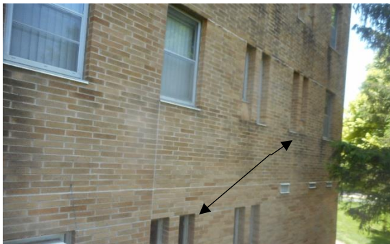
Photo #5 Overview of inoperable windows on Wing 71.
