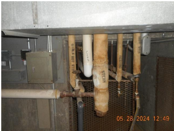
Photo #1 Asbestos pipe fittings – Wing 61 – Mech Room 108
