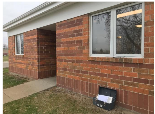
Photo #4 View of the Exterior of the Windows, Typical for all Windows on all Wings except the Dining Hall.
