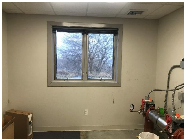
Photo #3 View of the Window in Conference Wing, West Most Room, Typical for Conference and Staff Wings.
