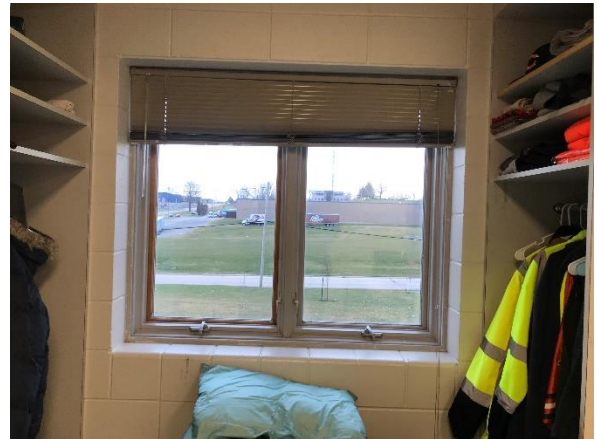
Photo #2 View of the Window A7, Typical for Windows in Wings A - D.
