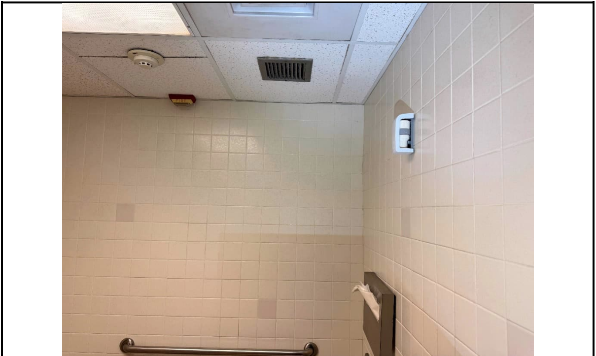
Photo 16: View of fluorescent lighting and associated light ballasts, emergency strobe lighting, a smoke alarm, and a motion sensor.
