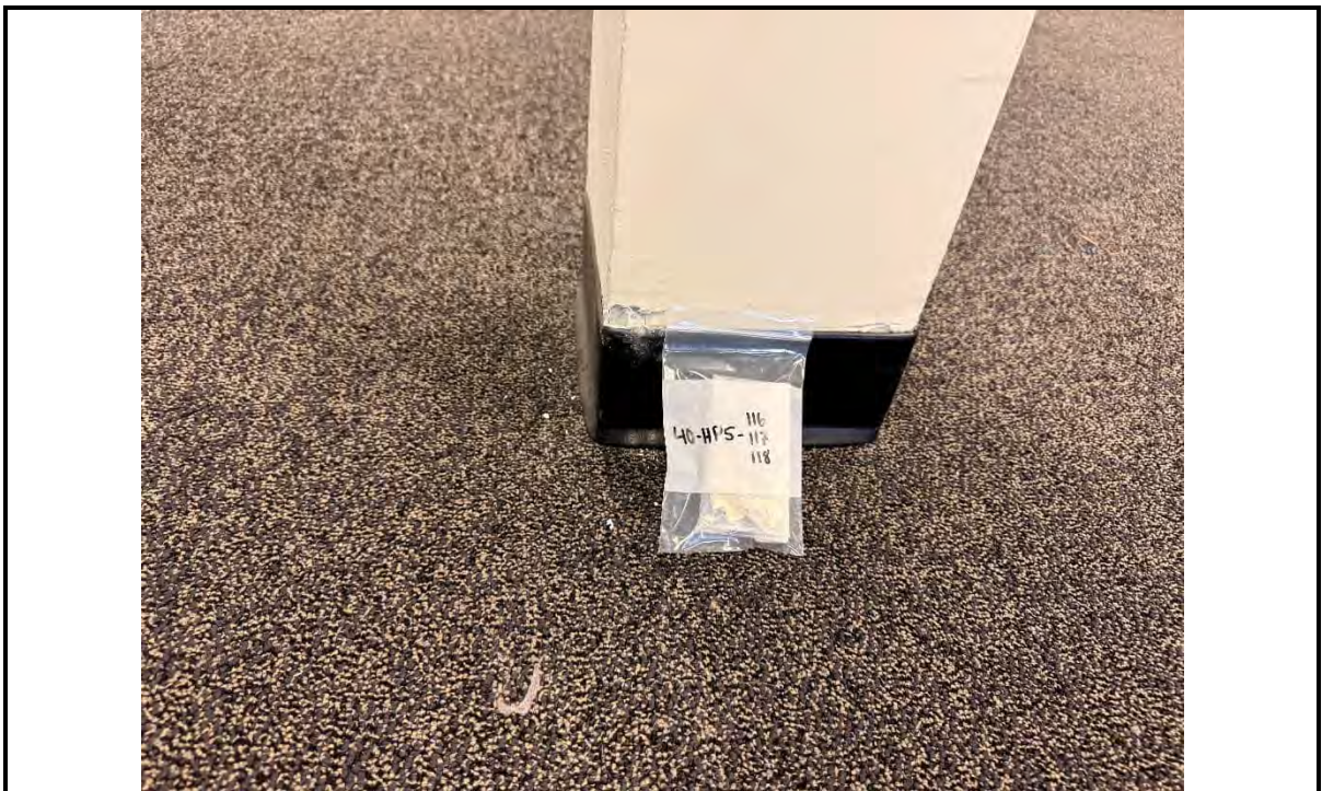
Photo 6: HA 40: Asbestos-containing surfacing material on support beam located in main open office area.
