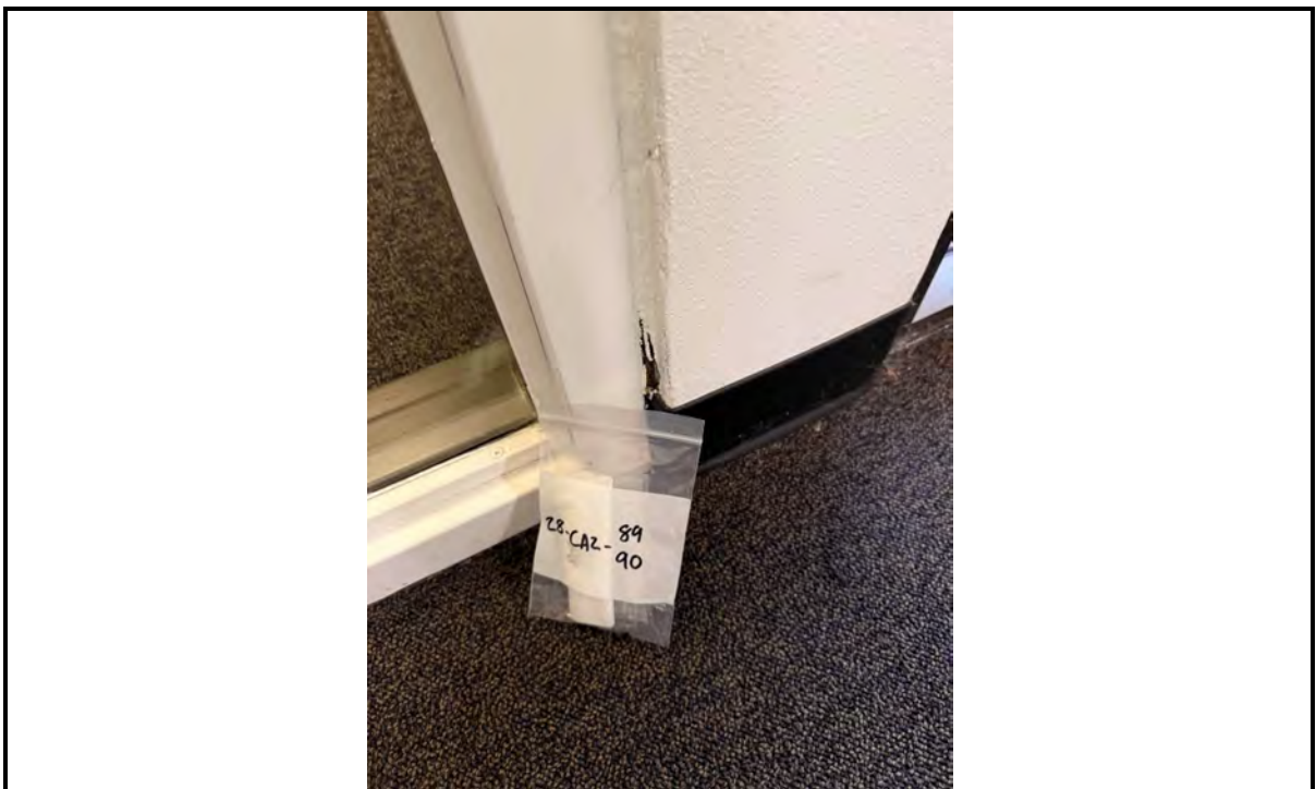
Photo 4: HA 12: Asbestos-containing grey caulk on southwest main entry door.
