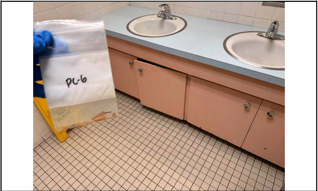
Photo 9: PC-6: Lead-containing pink paint located on cabinetry in women's restroom.
