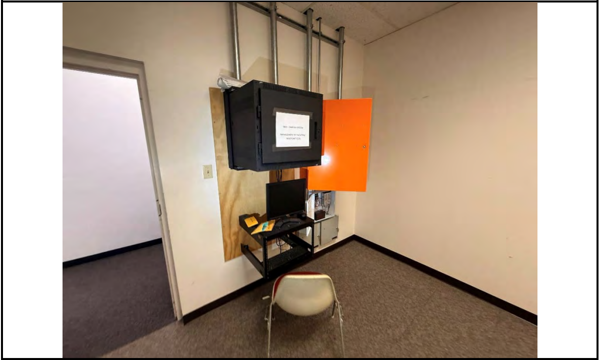
Photo 11: View of computer/server equipment present on site.
