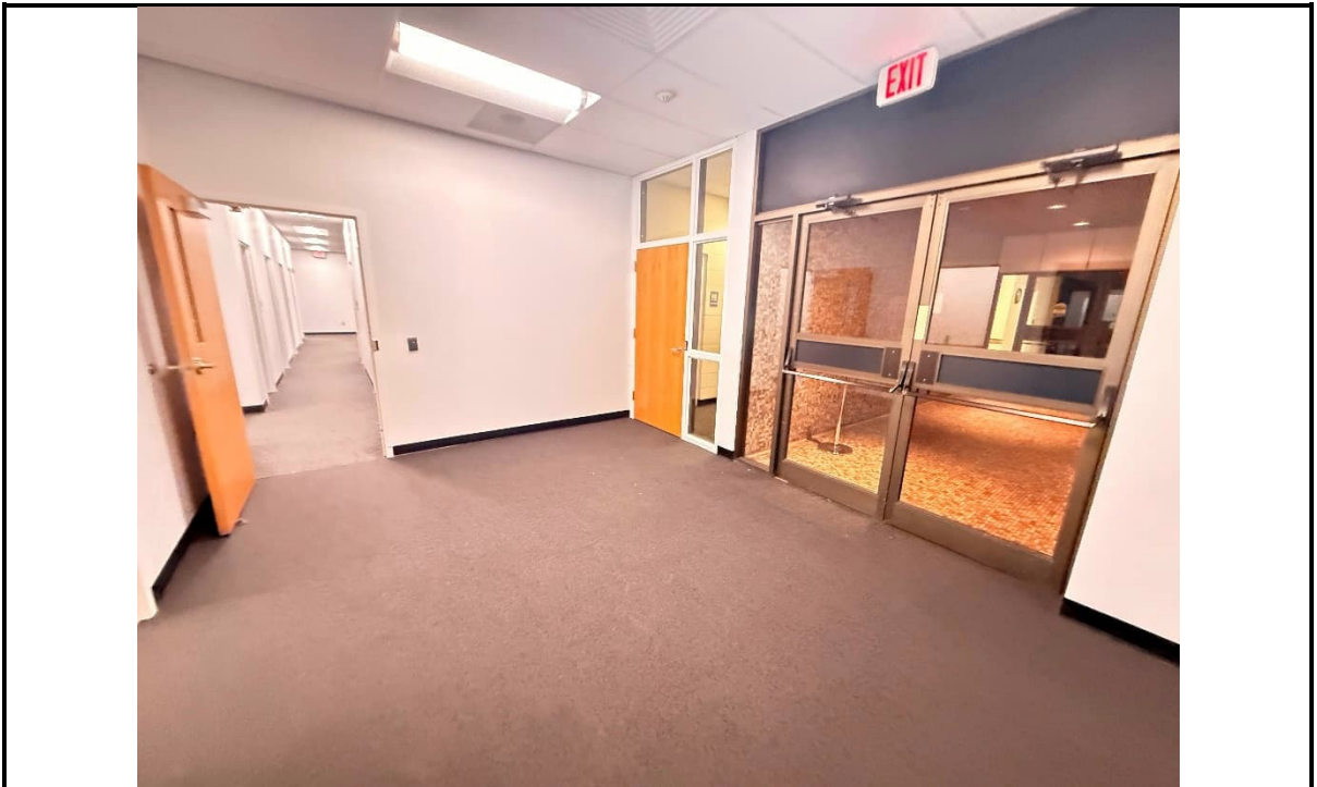
Photo 12: View of emergency exit signage, emergency strobe lighting, fluorescent lighting, associated light ballasts, and automatic door closers present on site.
