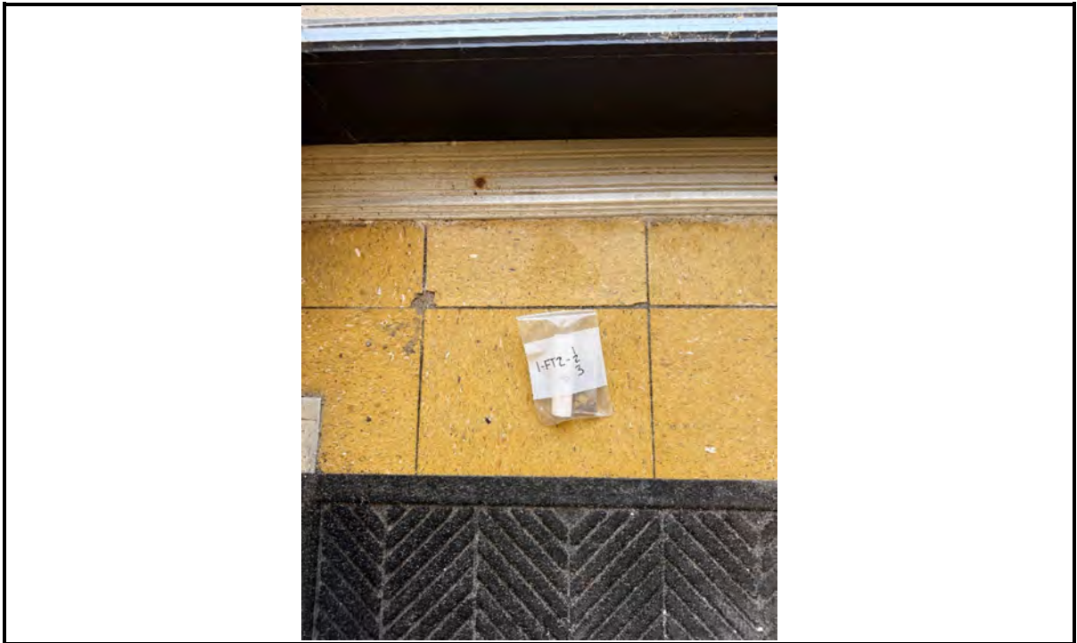
Photo 1: HA 01: Asbestos-containing brown 12"x12" floor tile and associated black mastic located in the entrance hallway at Door #1.
