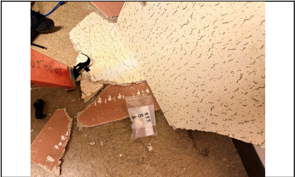
Photo 5: HA 38: Asbestos-containing ceiling tiles in Room #4.
