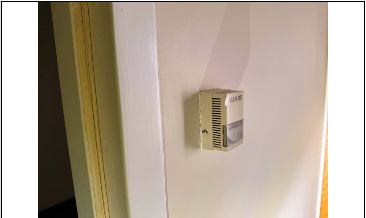
Photo 10: View showing a mercury switch thermostat on site.
