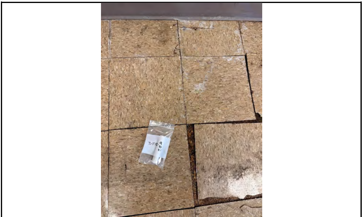
Photo 2: HA 03: Asbestos-containing black mastic under tiles in the breakroom, community area, and Room #4.
