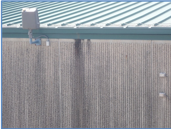
Photo 54: Staining on the concrete wall panel correlate to seams in the gutter system. Gutters are only located around portions of the Pods, not the entire perimeter as recommended for moisture management.
