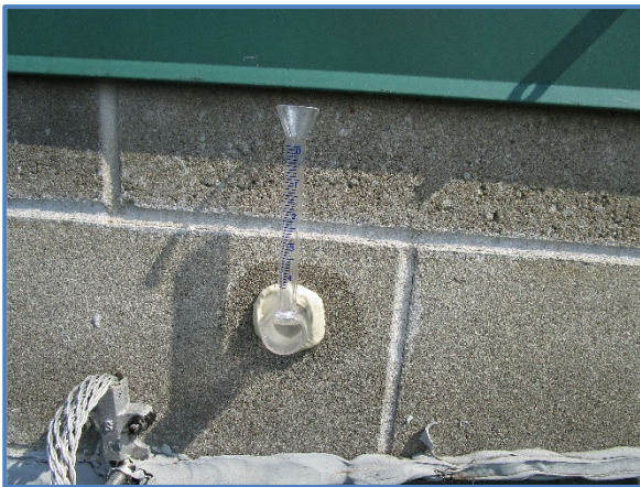
Photo 33: For the evaluation of CMU blocks, the original water level was 2.5ml and the final level after 20-minutes should lose no more than 0.5ml. The tube located on the CMU block wall, the tube completely emptied into the CMU in less than one minute, indicating the block is quite porous and absorbs water during rain events.
