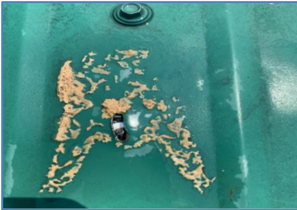
Photo 63: Hole in the metal roof panel where the lightning protection damaged the roof.
