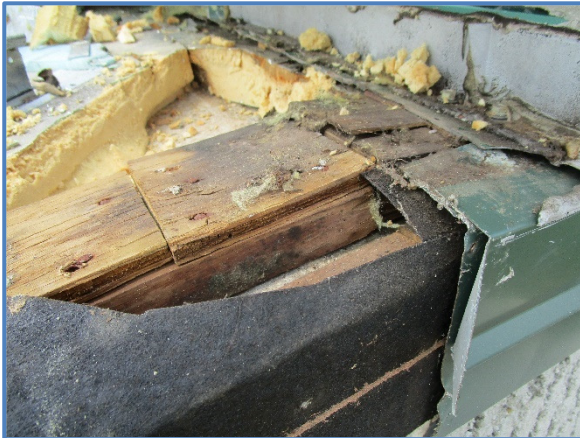
Photo 45: Removal of the metal drip edge revealed there are two separate sections of metal drip edge installed over a small section of membrane flashing. This does not match the detail from the construction drawings provided.
