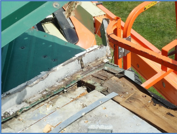
Photo 40: Removing the metal drip edge exposed the wood blocking that exhibits water stains and other signs of moisture intrusion. At the time of this inspection the wood blocking was not wet.
