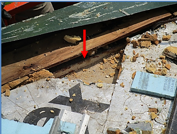
Photo 41: A section of the rigid insulation board was removed to allow for inspection of the concrete deck. There was no fully adhered vapor barrier installed underneath the rigid insulation board, as is common practice with concrete roof decks. The rusted metal structural angle (Red Arrow) is also visible from the Cells below.
