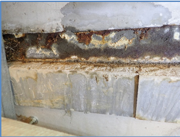
Photo 24: Deterioration is occurring at the metal structural plate holding up the concrete roof deck and concrete wall panel indicating prolonged exposure to bulk water infiltration.
