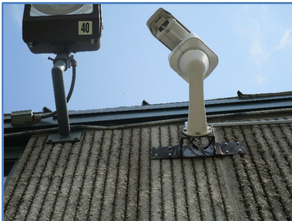
Photo 53: The metal roof panels do not extend over the metal drip edge allowing for water to roll back under the roof panels.
