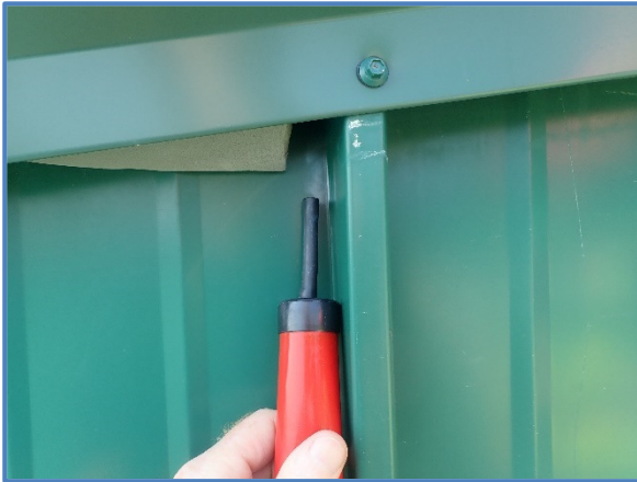
Photo 31: Along the area that was re-roofed in 2017 synthetic smoke demonstrated that outdoor air leakage into the building was occurring at this location.
