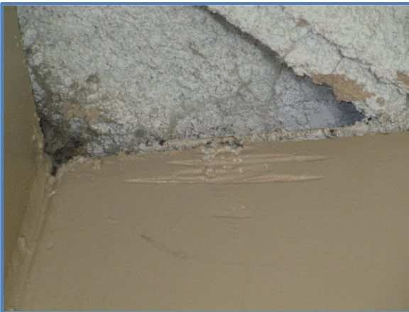
Photo 6: Cobwebs at the exterior wall to roof transition on the 2 nd Floor demonstrates air leakage at this location. Synthetic smoke and infrared imaging confirm the story told by the spiders. The exterior wall to roof deck transition is unsealed in multiple areas; synthetic smoke clearly illustrates these areas as air leakage sites. Depending on the temperature difference between indoors and outdoors, airflow direction (and other factors) infrared imaging will not always show air leakage.
