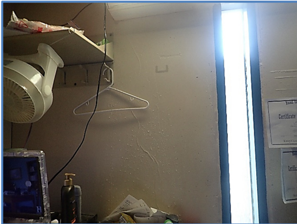
Photo 65: Water was observed running down the wall during the nozzle test at the hole from the lightening protection.
