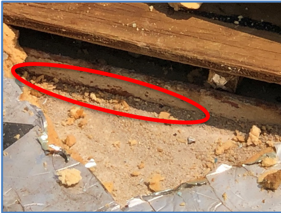
Photo 42: Close up view of the metal structural angle holding the concrete roof deck in place. A small crack is observed between the metal and concrete (Red Circle).
