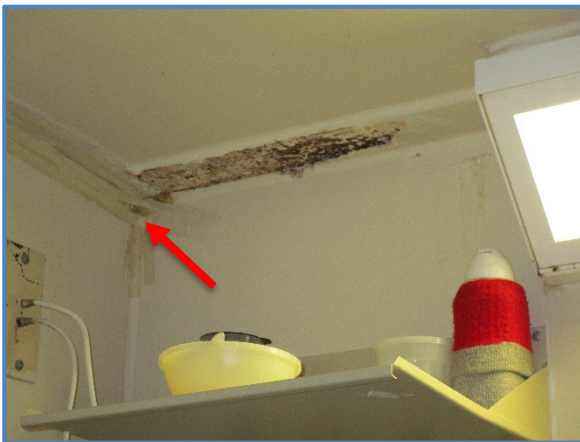
Photo 8: The metal structural angles to hold the concrete deck to the precast concrete panel located throughout the building are rusting; likely due to the bulk water entering from the roof assembly.
