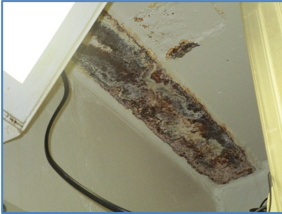
Photo 11: Rust on the structural angle supporting the concrete roof deck is observed throughout Pod-C. This is likely from prolonged bulk water intrusion from the concrete wall panel and concrete roof deck.
