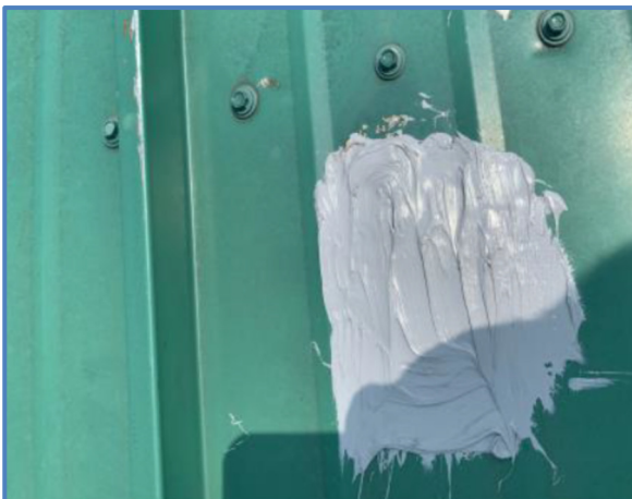
Photo 64: Temporary repair was completed by Tremco while onsite to prevent further bulk water intrusion at this location.
