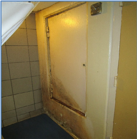
Photo 12: On the first floor the access panel for the plumbing/mechanical chase is located in a shower stall. Having an access panel located in a shower stall promotes the moisture pathway into the chase.
