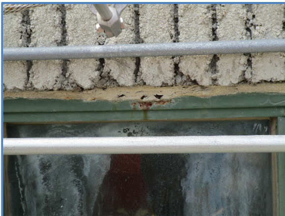
Photo 47: The caulk joint around the window assembly has deteriorated resulting in damage to the metal window frame and the glazing.
