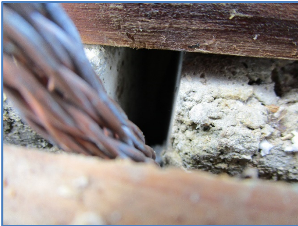
Photo 44: A closer inspection of the sealant joint in the concrete wall panel system revealed that the seam is open behind the wood blocking. This opening in the sealant joint allows bulk water to enter the concrete wall panel and enter the conditioned space.
