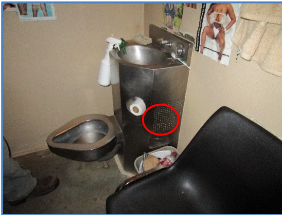
Photo 2: Metal toilet and sink combination in each cell has an opening into the plumbing chase that serves as the return plenum. Excess return airflow creates a significant negative pressure in the Pods.
