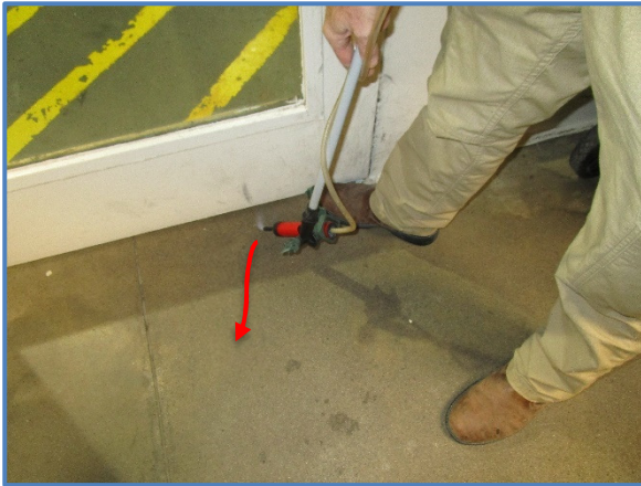
Photo 19: Synthetic smoke demonstrates the negative pressure between the Unit 1 of Pod-C. Standing in the hall area outside Unit 1, smoke directed at the Pod-C Unit 1 door is rushing back towards the hall.
