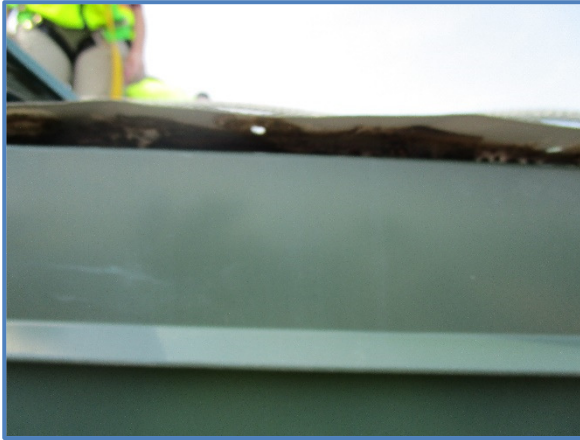
Photo 37: The standing metal seam roof panels are not continuously sealed to the metal drip edge. Some locations are missing screws. These defects will allow water to roll under the standing seam roof; wind driven rain will enter the assembly in even greater amounts.
