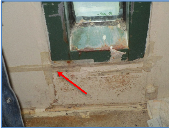
Photo 10: Tape (Red Arrow) has been installed in an attempt to prevent bulk water intrusion. Signs of bulk water intrusion were observed throughout Pod-C.
