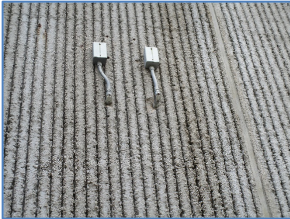
Photo 51: Multiple penetrations through the precast wall panel are unsealed. Water can run in through this penetration or be sucked in due to the negative pressure on the other side of the wall.
