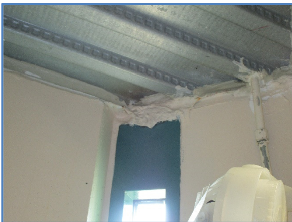
Photo 18: Exterior wall to roof deck transition has been repaired with caulk but the sealant is not continuous and will continue to fail until the bulk water intrusion from the roof is repaired.
