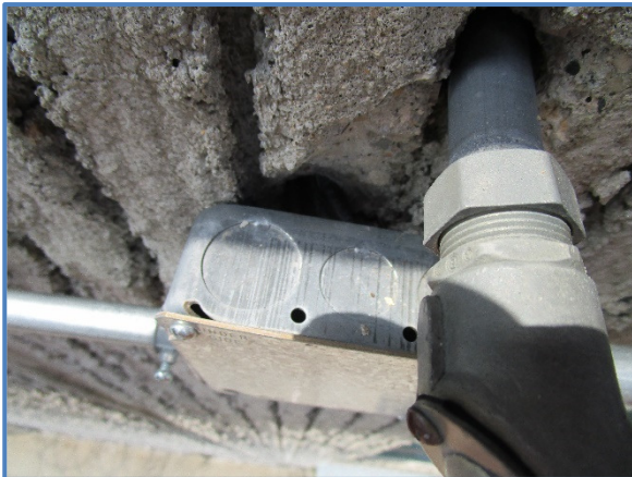
Photo 50: Multiple penetrations through the precast wall panel are unsealed. Water can run in through this penetration or be sucked in due to the negative pressure on the other side of the wall.
