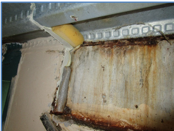
Photo 15: Removing the light fixture revealed that the metal deck is completely unsealed at the top of the concrete wall panel transition to the wall. Rust is occurring on the light fixture and on the structural metal angle.
