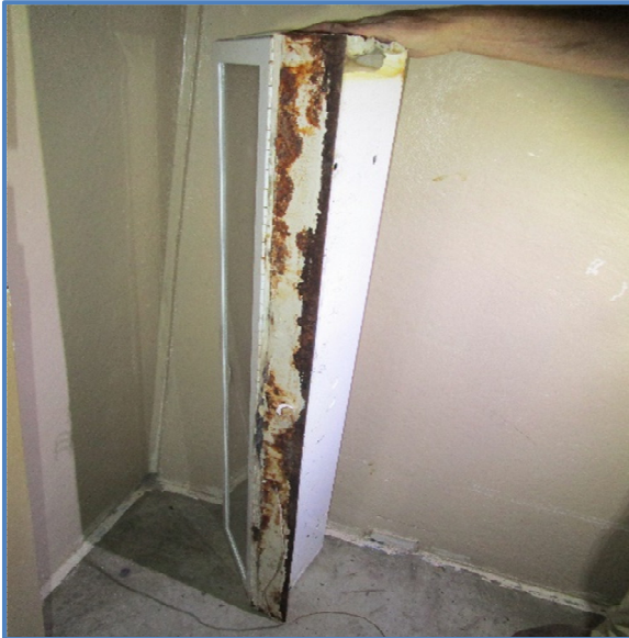
Photo 17: Rust occurring on the light fixture removed from Pod-C cell 16 as the result of air leakage and bulk water intrusion.
