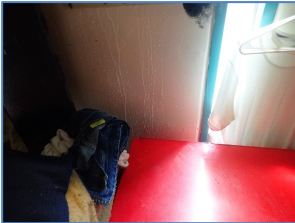
Photo 66: Water was observed running down the wall during the nozzle test at the hole from the lightening protection.
