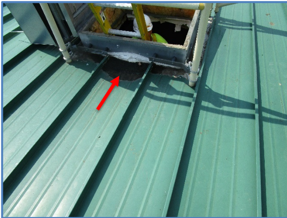
Photo 29: Cricket installed adjacent to the roof hatch appears to be too small and does not properly direct water away from the opening.
