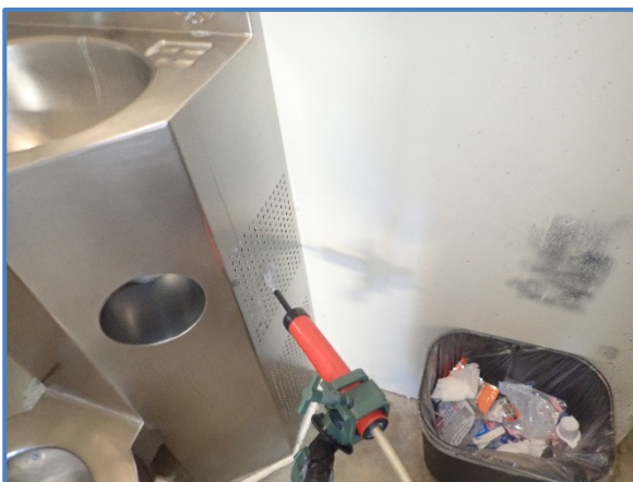
Photo 3: Synthetic smoke demonstrates that the opening in the toilet and sink combination serves as the return air termination for the mechanical system. The return air flows through the plumbing chase which also functions as plenum return which travels up the chase and opens into the Pod common area.
