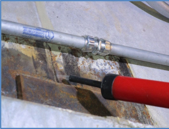
Photo 23: Synthetic smoke illustrates an air leakage pathway under the standing metal seam roof where the concrete roof deck ties into the smooth precast wall panel.
