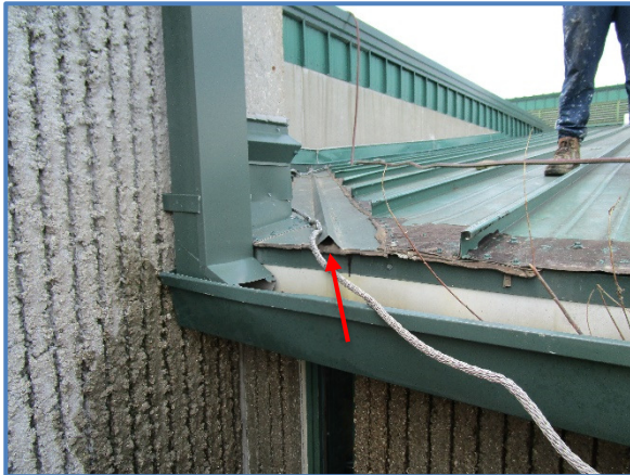
Photo 57: AAMA 501 nozzle was used to test for water penetration at the roof over Pod-C Unit 1 along the south elevation to determine the cause of the bulk water intrusion. Nozzle testing at the valley determined water entry was occurring under the panels (Red Arrow).
