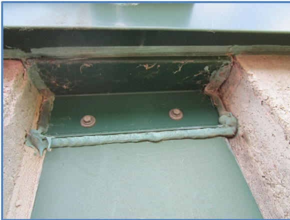
Photo 46: The metal drip edge for the roof assembly was sealed to the precast wall panel from underneath – it is reported that the metal drip edge was replaced after the original construction. A piece of metal drip edge appears to have been installed at a window head. No invasive inspection was conducted above the window assembly to document the construction in this area. The sealant around the perimeter of the metal is not continuous.
