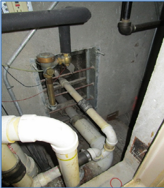
Photo 4: Inside view of the plumbing chase that is used as part of the return air plenum. The plenum is also connected to floors below through the plumbing chase. It is reported that several of the chases have standing water in the bottom of them, presumably from ground water seeping into the building.
