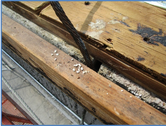
Photo 43: The lightning protection has been installed through the joint in the concrete fractured fin exterior wall panel.
