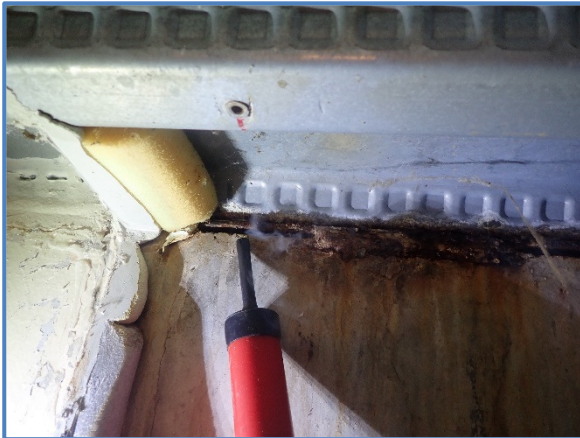
Photo 16: Synthetic smoke demonstrates inward air leakage occurring at the transition between the top of the concrete wall panel and the underside of the roof deck. Air leakage will add to the moisture load on the mechanical system and can cause condensation inside the light fixture.
