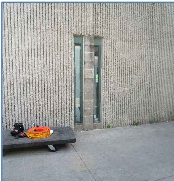
Photo 56: Around the main area of the facility CMU block is observed between the fixed windows. These blocks appear uncoated and likely allow water to penetrate as was demonstrated with the Rilem test for the CMU block at the fire walls.
