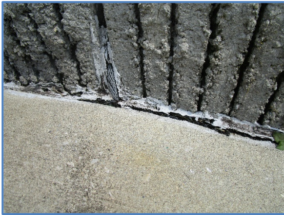
Photo 52: The caulk joints have deteriorated at the seams in the concrete wall panels as well as the joint between the wall and the sidewalk. These deteriorated joints allow for water intrusion.
