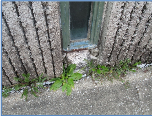
Photo 48: CMU block infill below the window assembly has been damaged. Rust is observed on the window frame.
