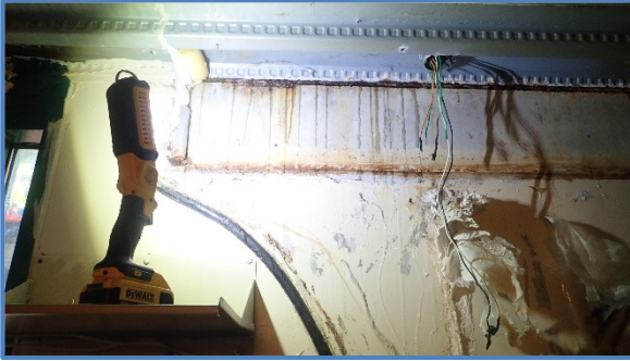
Photo 60: When nozzle testing was conducted around the valley pan, water was observed running down the inside of the precast wall panel in Pod-C-Unit 1, Cell 16. at the unsealed location behind where the light fixture had been removed.
