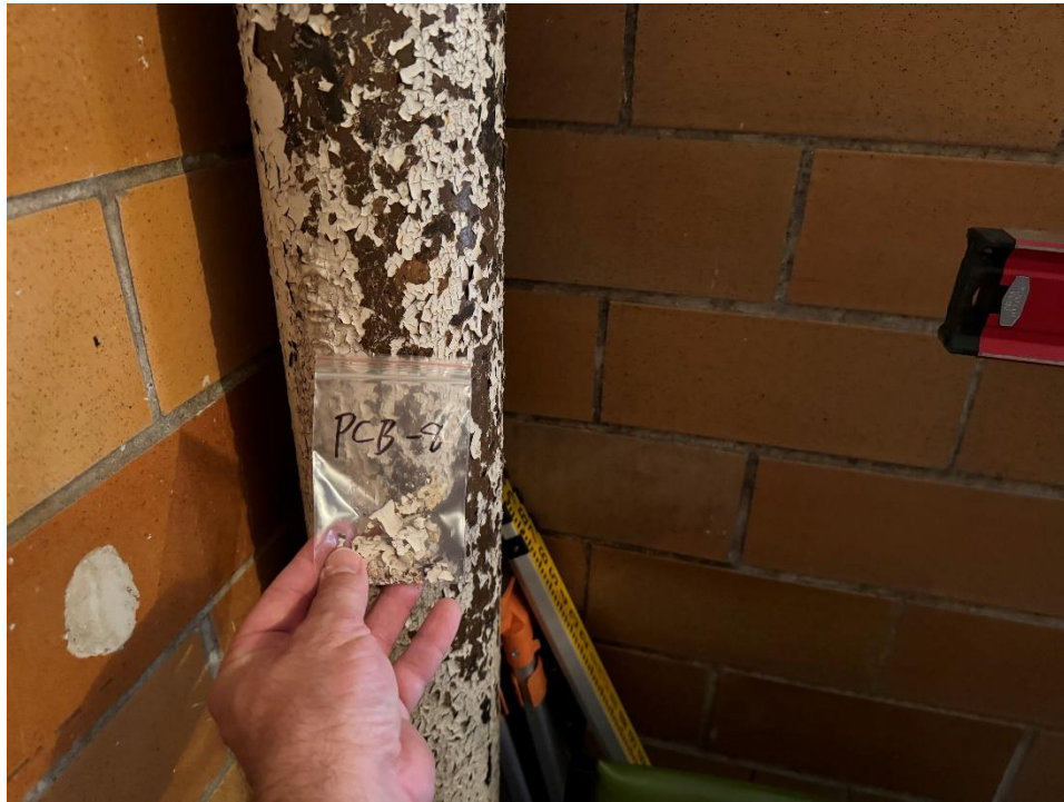
View of the White Lead Containing Paint. (PCB-8, 0.26% Pb)
