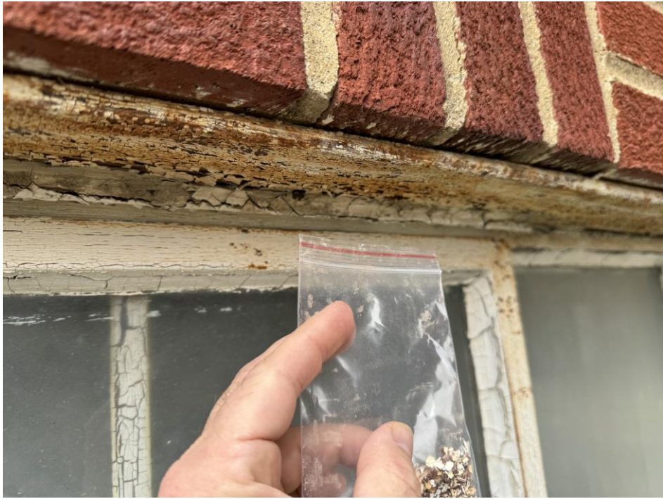
View of the White Lead-based Paint. (PCB-15, 10% Pb)
