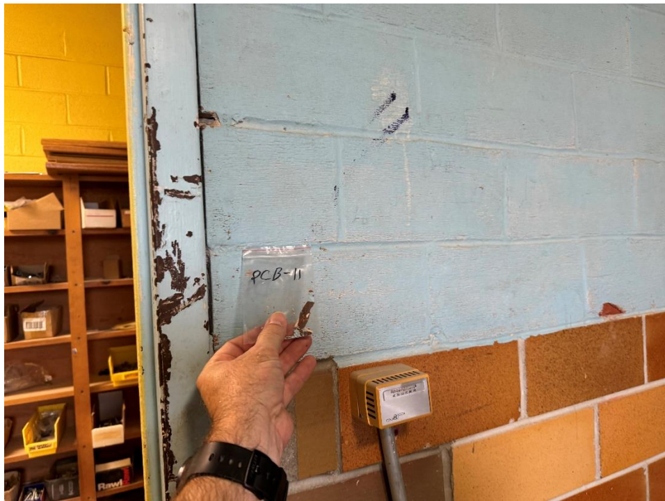
View of the Light Blue Lead Containing Paint. (PCB-11, 0.26% Pb)
