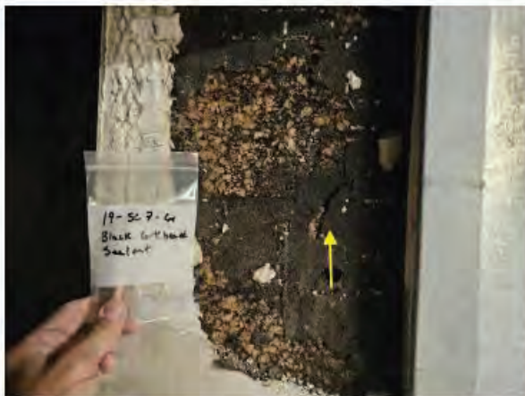
Photo #5 Yellow arrow pointing at asbestos containing black corkboard sealant, HA 19.
