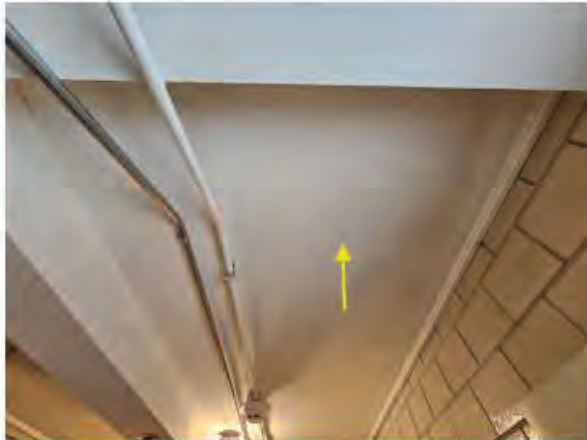
Photo #1 Photo of asbestos containing material (ACM), white plaster, homogenous area (HA) 01.
