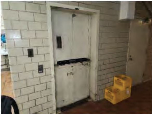
Photo #15 View of lead containing door frame paint.
