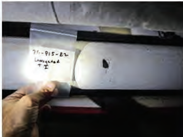
Photo #9 Photo of asbestos containing TSI corrugated paper pipe wrap, HA 26.
