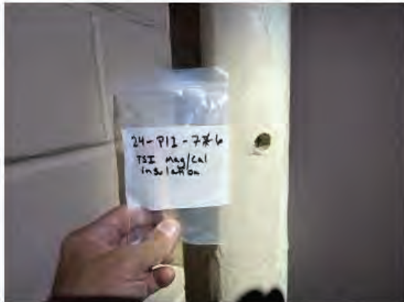
Photo #7 Photo of asbestos containing TSI Mag/Cal pipe insulation, HA 24.
