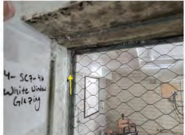
Photo #2 Photo of asbestos containing white window glazing, HA 14.
