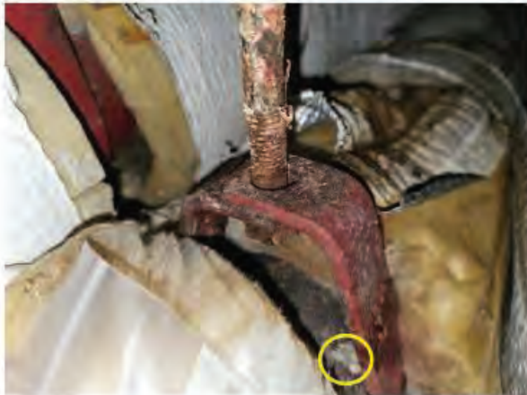
Photo #3 Yellow circle indicating asbestos-containing residual white thermal system insulation (TSI) mudded fitting on fiberglass pipe, HA 17.
