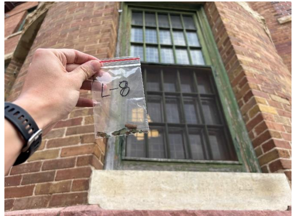
Photo #10 Sample L-8 Green Paint on Windows on South B 1 st Floor Window ( 17% Lead )
