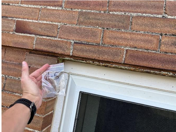
Photo #1 Sample A-5 Clear/Grey Caulk above basement window on north side of the building ( 8% Chrysotile )
