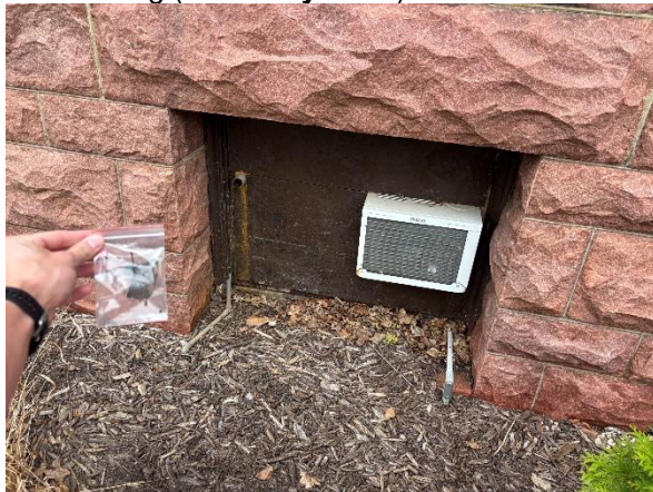
Photo #3 Sample L-1 Brown Paint on Admin Building Basement Windows ( 6.7% Lead )
