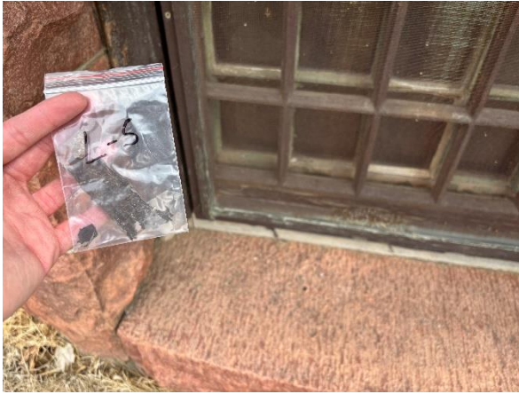
Photo #7 Sample L-5 Brown Pain on North C West Side Basement Window ( 4.5% Lead )
