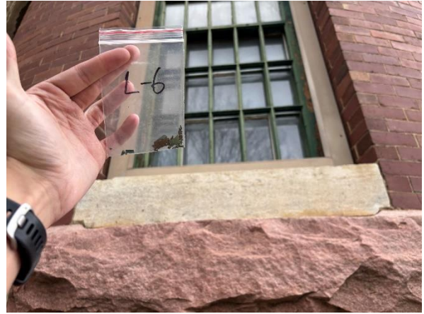
Photo #8 Sample L-6 Green North C on 1 st Floor Window ( 16% Lead )
