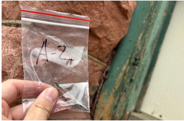
Photo #1 Sample A-2 Red Grout/Stone around 1 st Floor Green Trimmed Windows of Admin Building ( 15% Chrysotile )
