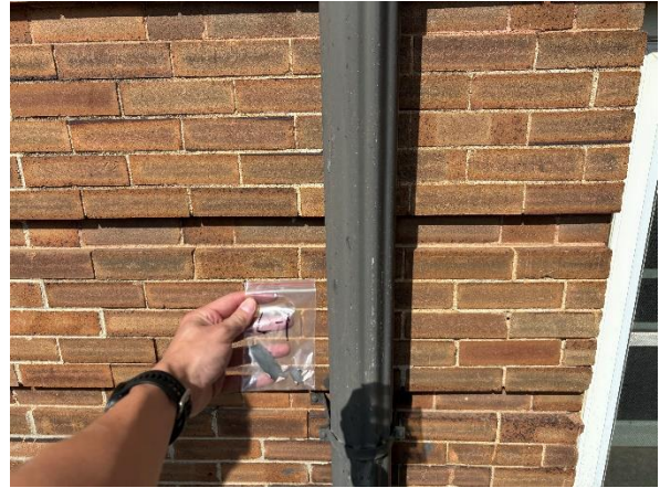
Photo #2 Sample L-1 Black Paint on building downspouts ( 1.3% Lead )
