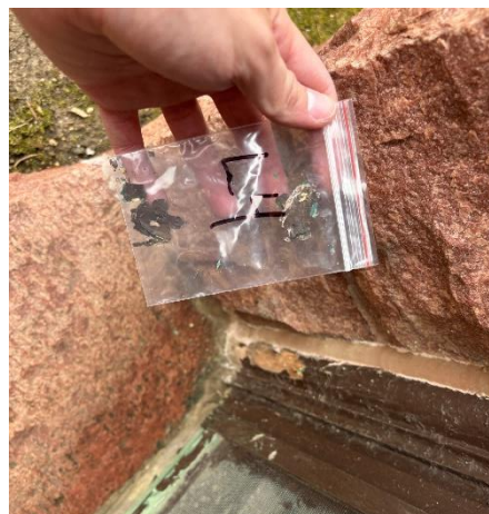
Photo #6 Sample L-4 Brown Paint on North A Central Basement Window ( 9.3% Lead )
