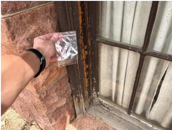
Photo #9 Sample L-7 Brown paint on Rear Center Basement SW Window ( 11% Lead )
