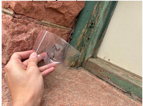
Photo #4 Sample L-2 Green Paint on Admin Building Windows ( 12% Lead )
