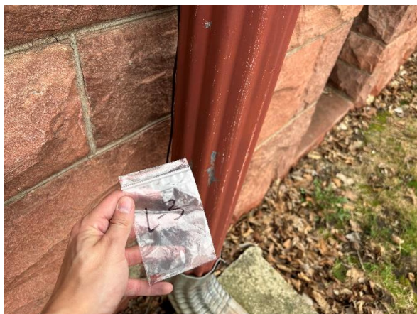
Photo #5 Sample L-3 Admin Building Red Paint on Down Spouts ( 17% Lead )
