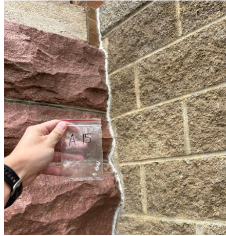
Photo #2 North C 1 st Floor Addition, North Side Exterior (red stone to concrete block) – White Caulk ( 2% Chrysotile )
