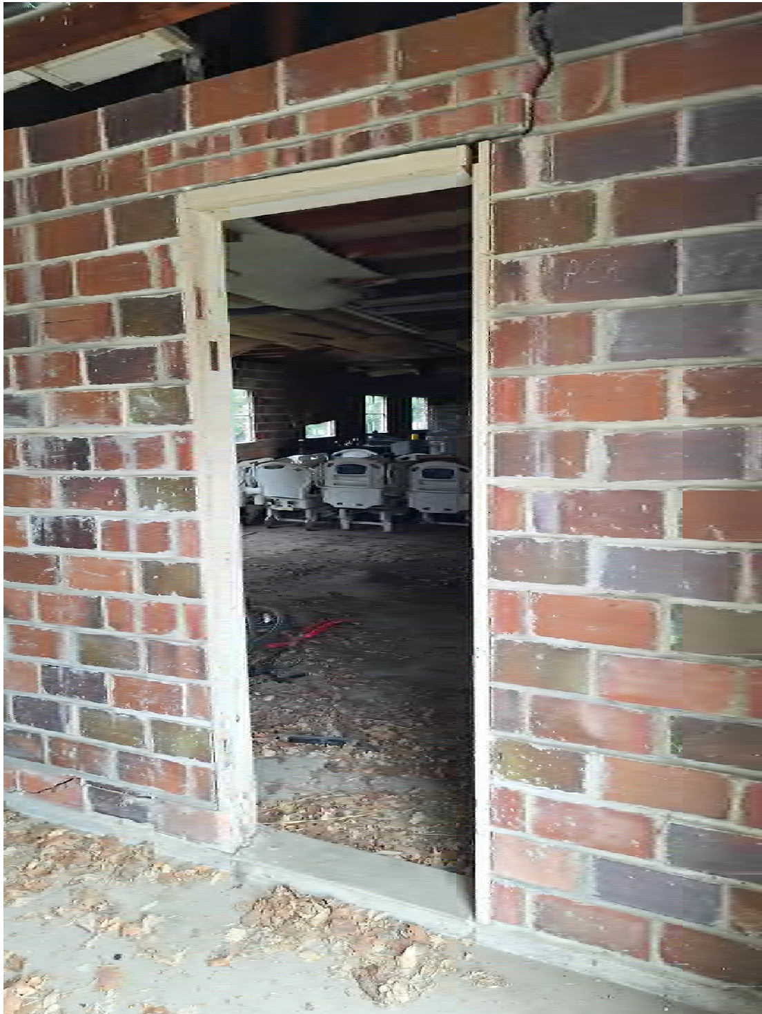
BUILDING INTERIOR - CRACK OVER DOOR IN CENTER TO BE REPAIRED
