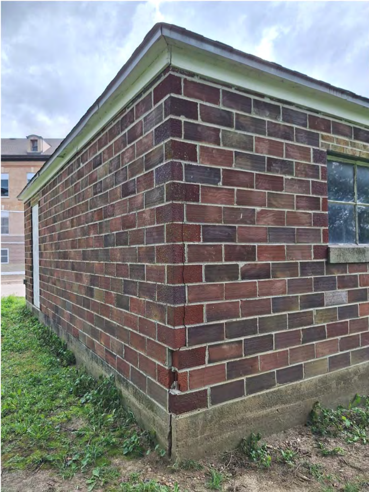
BUILDING EXTERIOR - CRACK ON NORTH WEST CORNER
