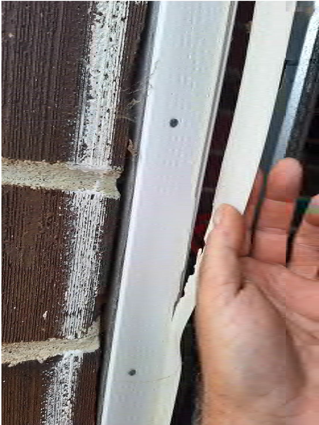
BUILDING EXTERIOR - TYPICAL STOP & WEATHERSTRIP TO BE REPLACED
