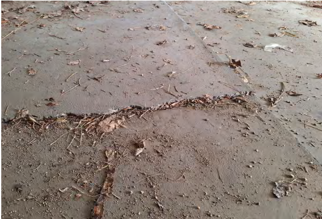
BUILDING INTERIOR - OFFSET FLOOR CRACK TO BE GROUND DOWN FLUSH
