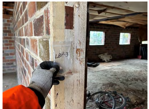
Photo #4 Lead-based paint (white) – CHMHI Fleet Garage interior door frame. (3.7%)
