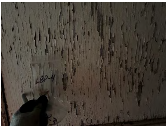
Photo #5 Lead-based paint (white) – CHMHI Fleet Garage interior wood door. (7.3%)
