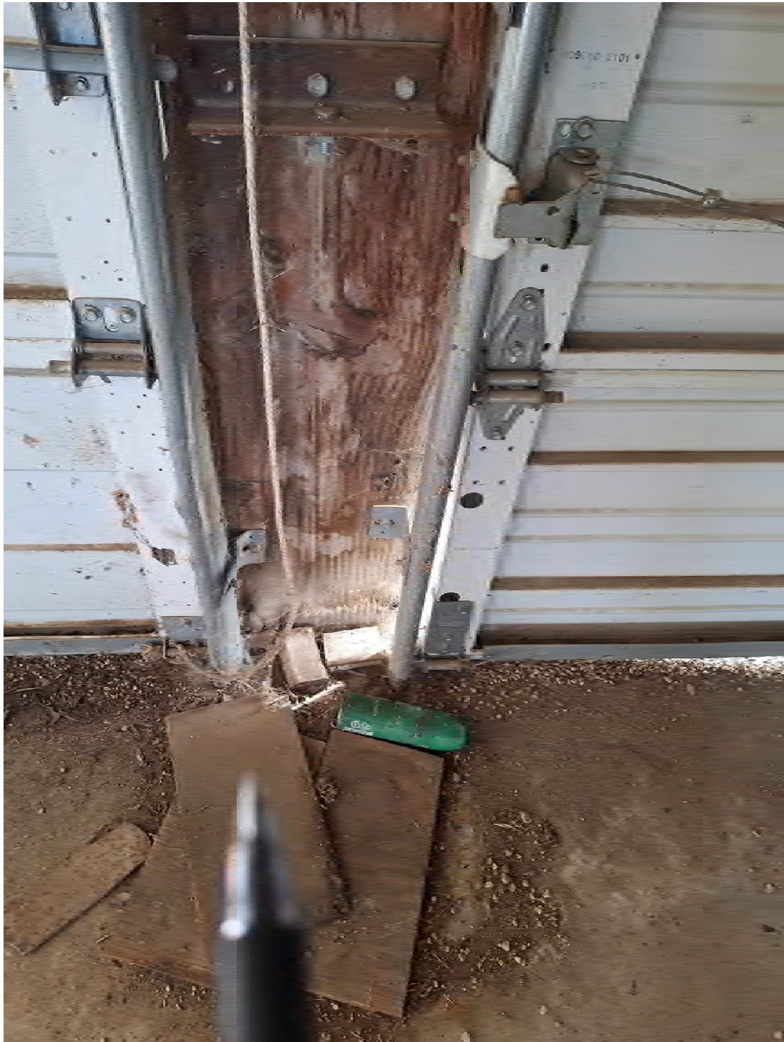
BUILDING INTERIOR - BENT TRACK SECTION TO BE REPLACED
