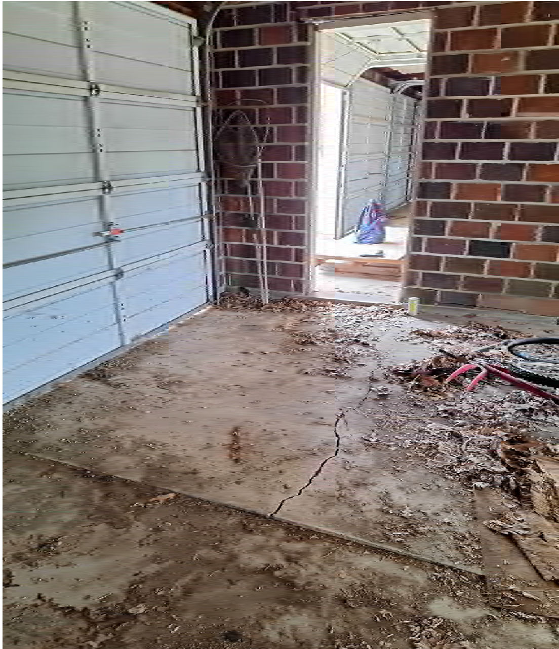
BUILDING INTERIOR - TYPICAL FLOOR CRACK TO BE SEALED
