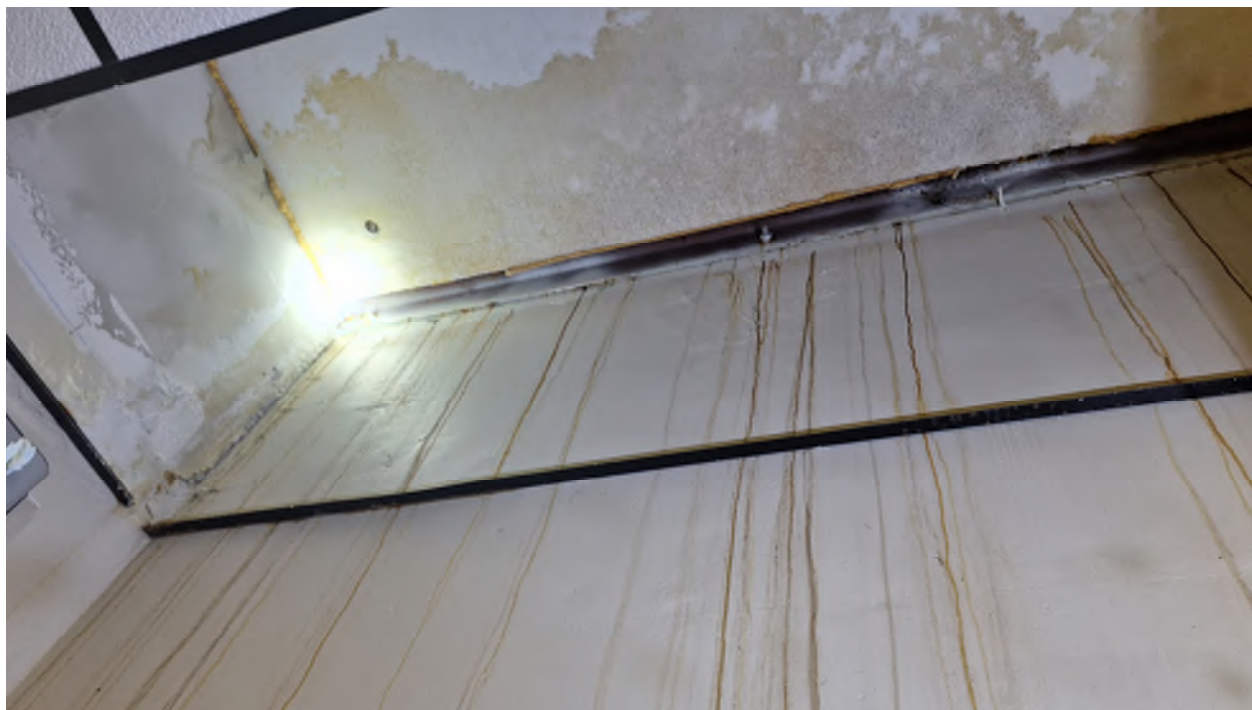
LOFTUS BUILDING - BASEMENT BAND ROOM - LEAKS ABOVE CEILING
