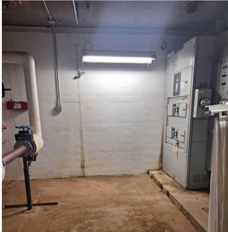
LOFTUS BUILDING - BASEMENT ELECTRICAL RM - ELECTRIC MDP & SUMP PIT #2 LOCATION
