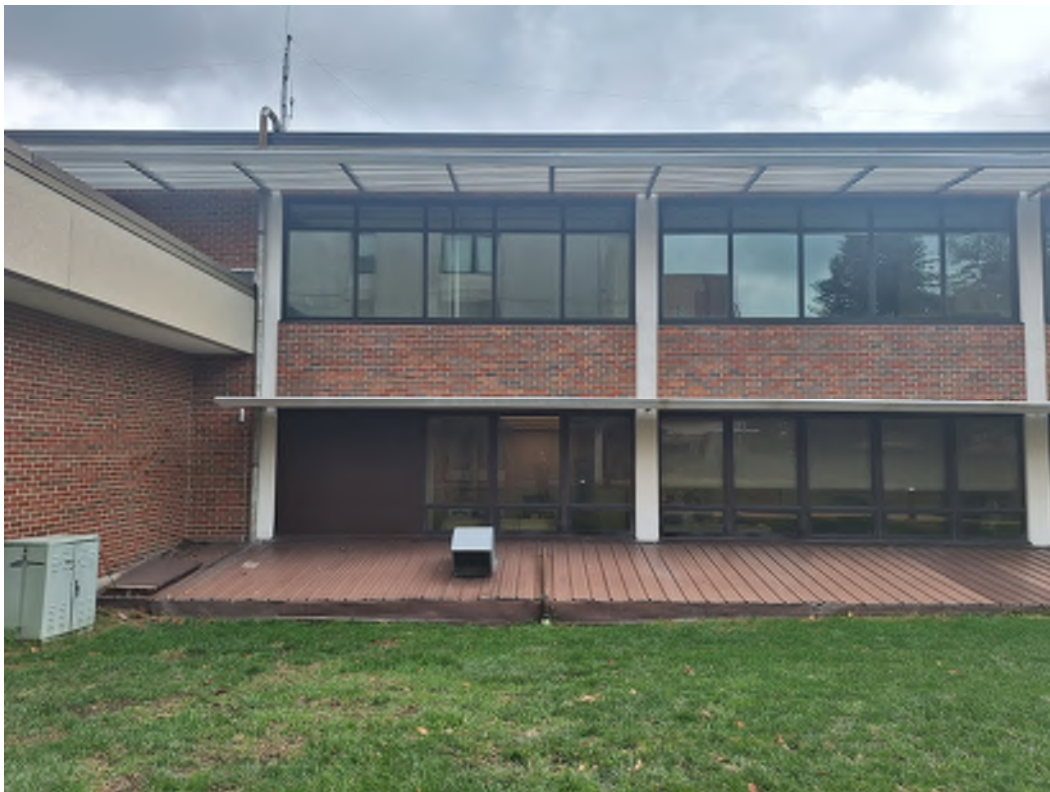
LOFTUS BUILDING - SOUTH WALL - NORTH END OF METAL ROOF AT ROOF HATCH
