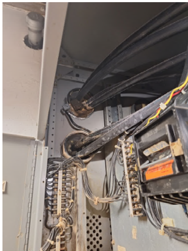
LOFTUS BUILDING - BASEMENT ELECTRIC RM - EXISTING CONDUITS IN MDP
