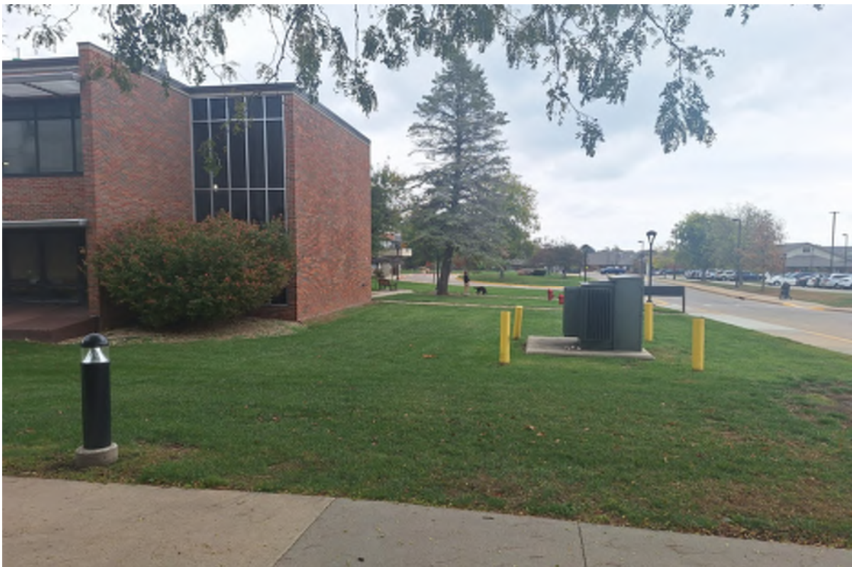
LOFTUS BUILDING - SOUTH WALL - TRANSFORMER AT SOUTH END
