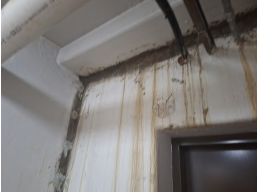
LOFTUS BUILDING - NORTH TUNNEL - INSIDE LEAKS & PATCHING
