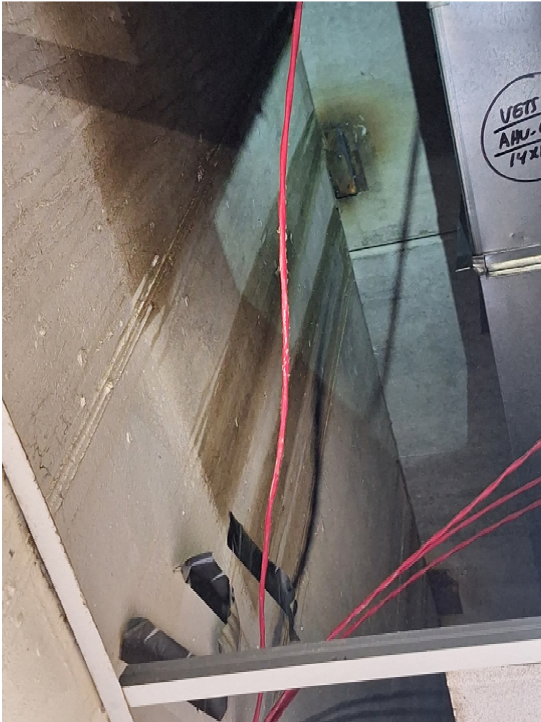
MALLOY BUILDING - NORTH KITCHEN TUNNEL - LEAKS ABOVE CEILING
