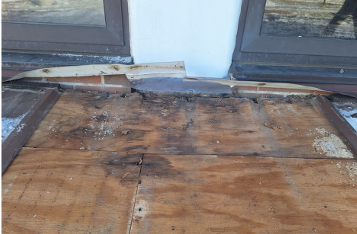
LOFTUS BUILDING - NORTH WALL - METAL ROOF ROTTED PLYWOOD
