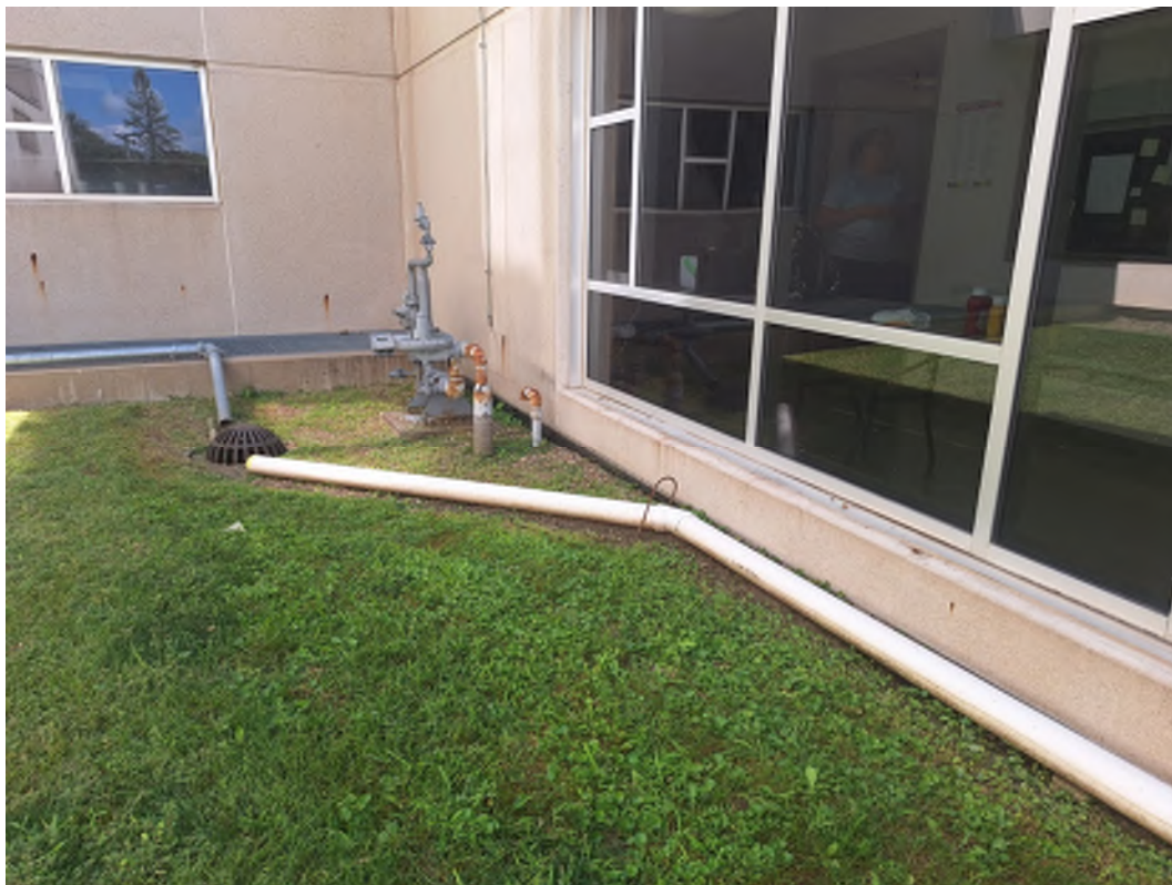
MALLOY BUILDING - NORTH KITCHEN GAS METER & ROOF DRAIN PIPING
