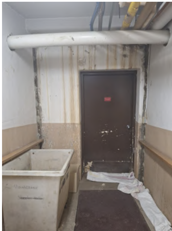
LOFTUS BUILDING - NORTH TUNNEL - INSIDE LEAKS
