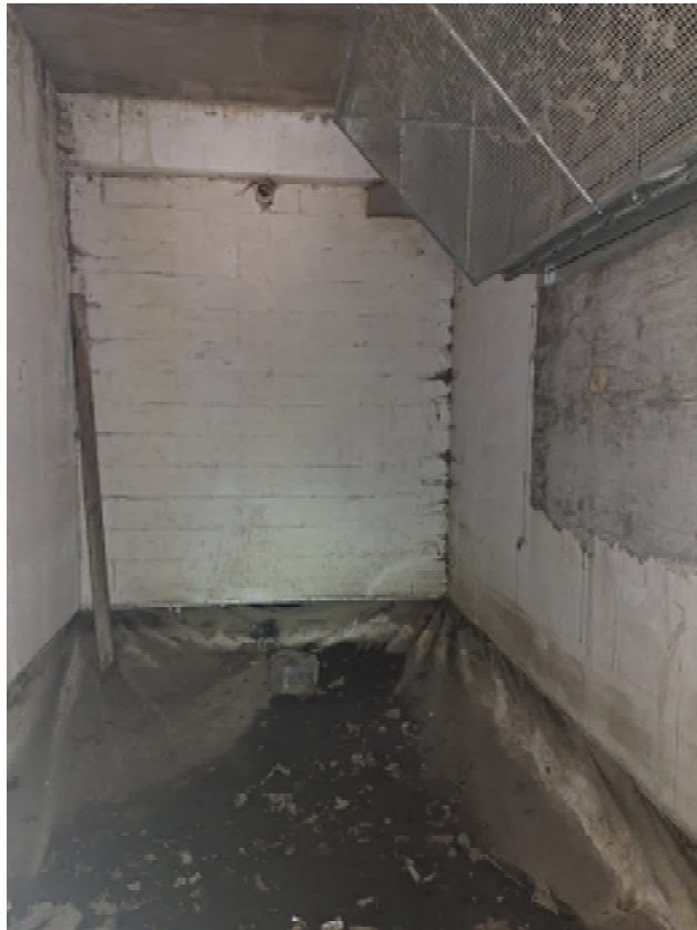
LOFTUS BUILDING - NORTH AIR HANDLING PIT - MEMBRANE PIT
