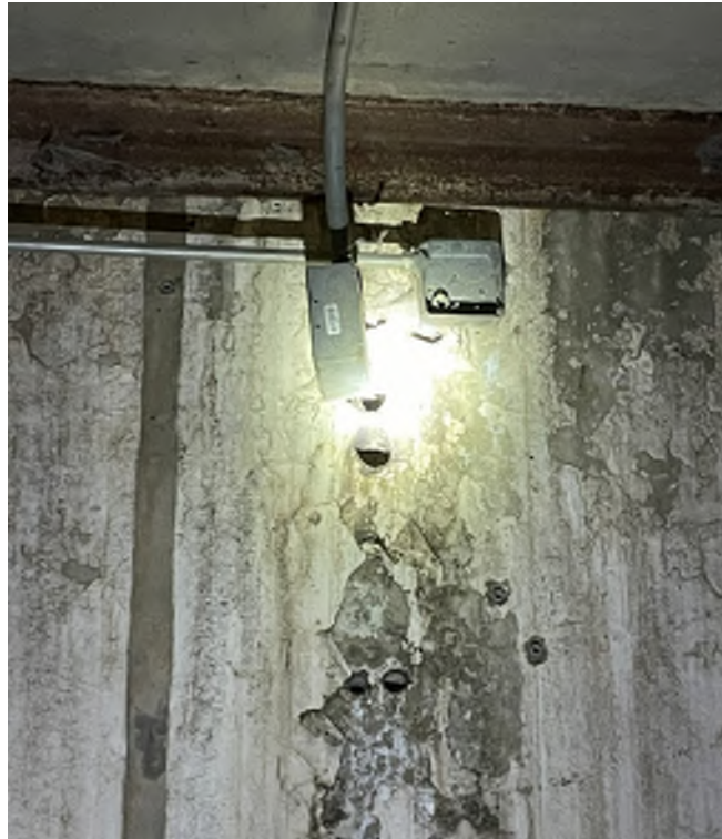
LOFTUS BUILDING - SOUTH AIR HANDLING PIT - PIPE PENETRATIONS TO BE PATCHED
