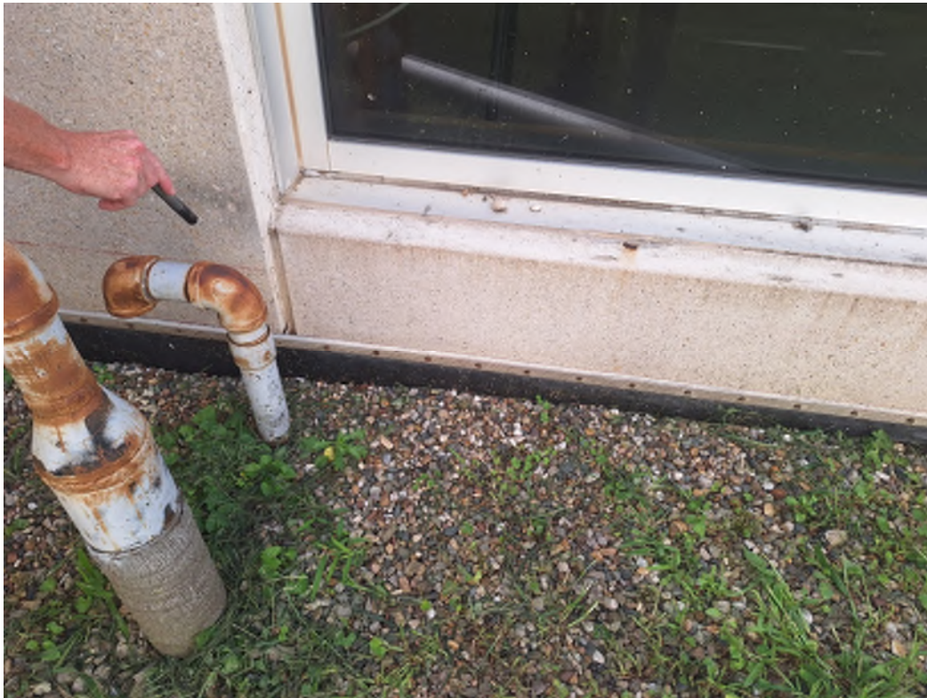
MALLOY BUILDING - NORTH KITCHEN GAS METER, EPDM TERM BAR & PRECAST JOINT
