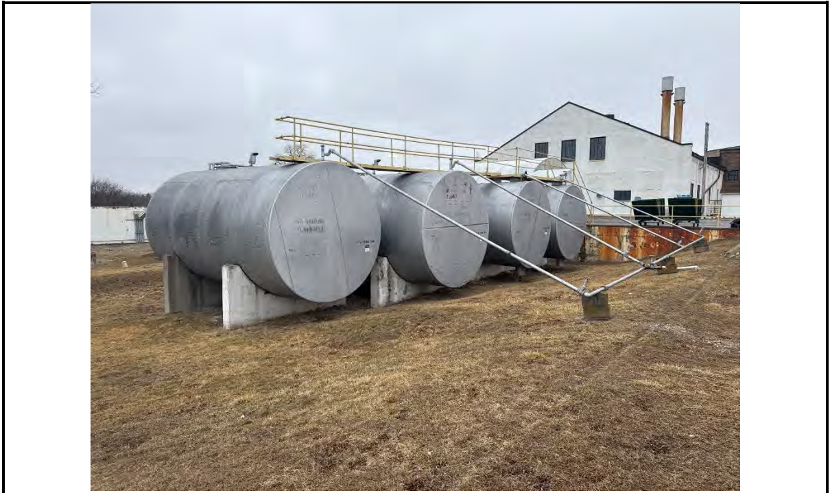
Photo 1: View of diesel tanks, tank paint contains lead above the laboratory reporting limit.
