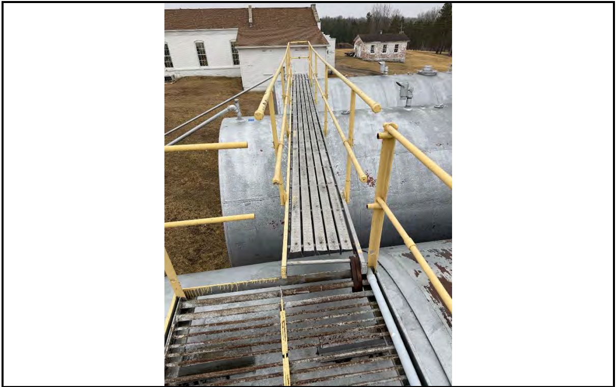
Photo 5: View of walkway above diesel tanks with yellow painted rails containing lead above laboratory reporting limit.
