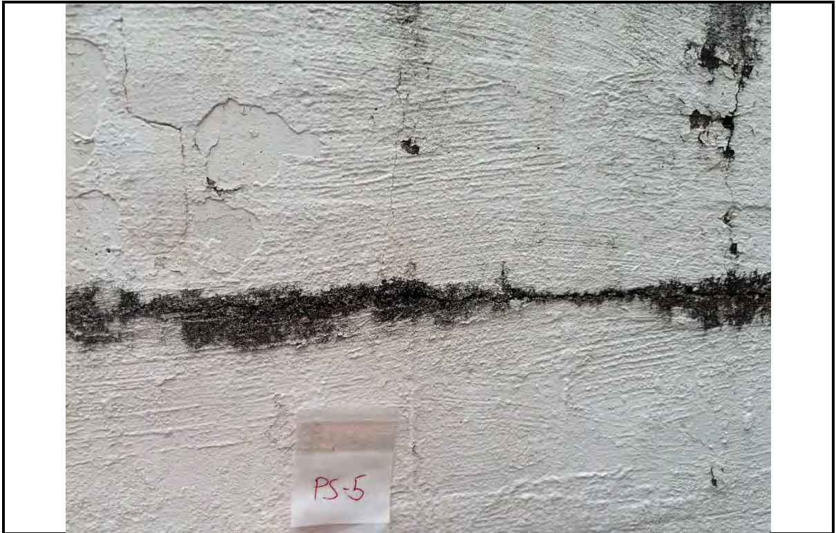
Photo 3: Sample PS-5 location, paint is 1.0% lead by weight. Sample also analyzed for asbestos, no asbestos was detected in the skim coat
