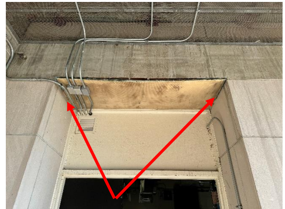
Photo #4 Another Photo of the Asbestos Containing Caulk above Loading Dock Doors.
