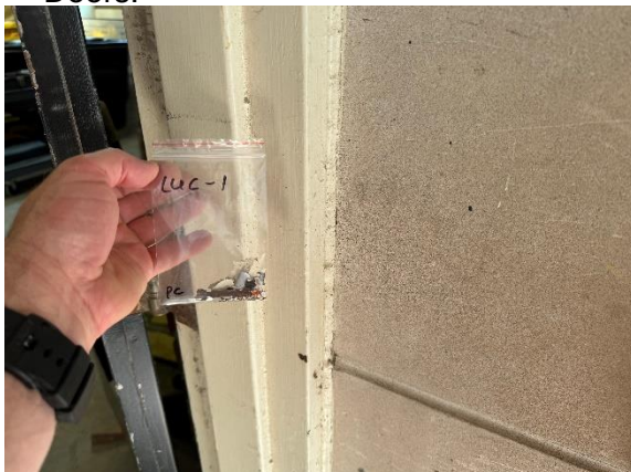
Photo #5 Looking at Off-white LBP on Loading Dock Doorframe.
