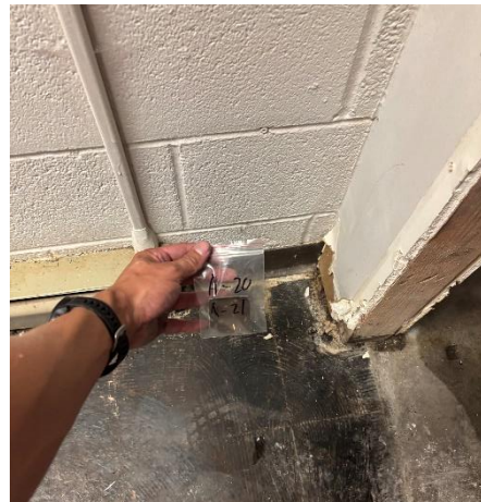
Photo #8 Sample A-21. Asbestos containing drywall mud/joint compound (on back of cover base).
