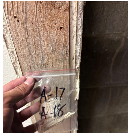
Photo #4 Sample A-18. Asbestos containing drywall mud/joint compound.
