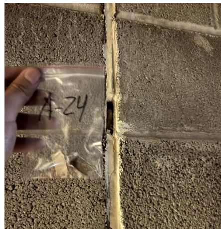
Photo #6 Sample A-24. Asbestos containing expansion joint (lower layer) on the north wall of the 1 st floor.
