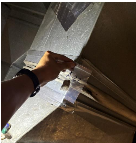
Photo #5 Sample A-22. Asbestos containing HVAC vibration dampener on 1 st floor unit.
