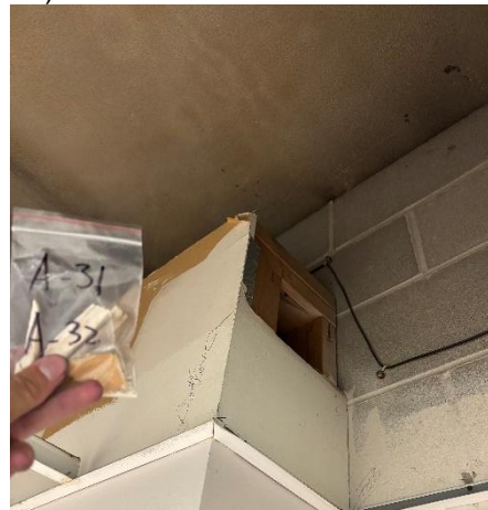
Photo #10 Sample A-32. Asbestos containing drywall mud/joint compound.
