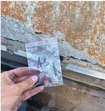
Photo #13 Sample A-5. <1% asbestos containing grey caulking on large stack on roof.
