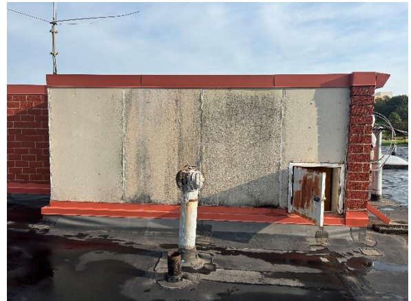
Photo #2 Sample A-7. Asbestos containing transite panels on roof access in the southwest corner of the roof.
