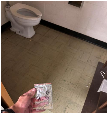
Photo #9 Samples A-38, A-39. Asbestos containing 9" x 9" pink floor tile and black mastic.
