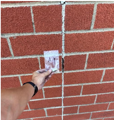
Photo #3 Sample A-9. Asbestos containing grey expansion joint on the exterior north wall.
