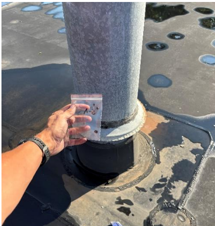
Photo #1 Sample A-2. Asbestos containing grey caulking on central vent stack on roof.
