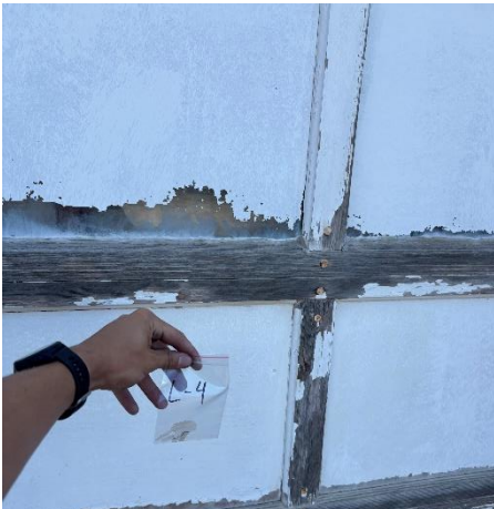
Photo #15 Sample L-4. Lead-based paint (white), on northwest garage door.
