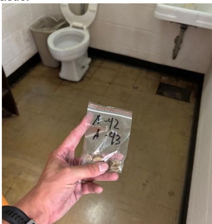
Photo #11 Samples A-42, A-43, A-44. Asbestos containing 9" x 9" tan floor tile and black mastic.
