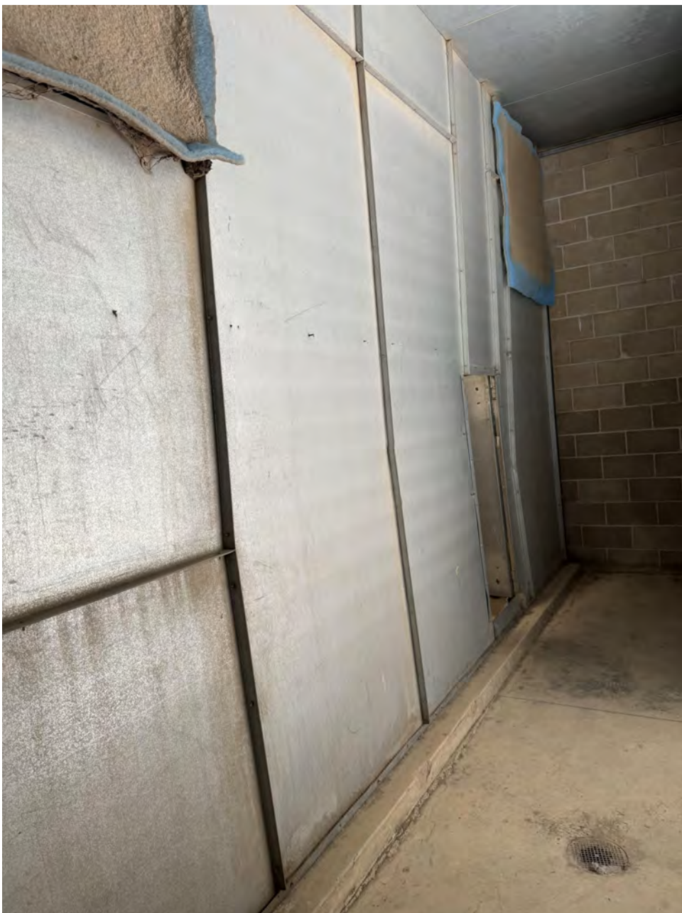
PHOTO 11 FACING NORTH EAST INSIDE PLENUM
