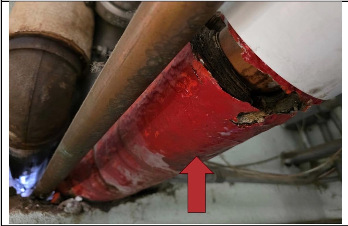
Photo 1: View of HA-3, asbestos-containing TSI layered paper pipe insulation and mudded fitting.
