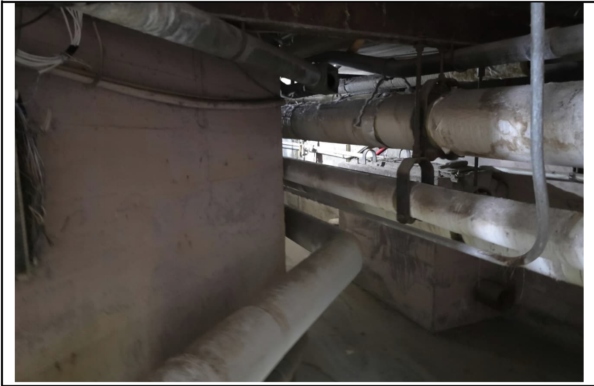
Photo 3: View of PC-1, pink lead-containing paint, located on the Powerhouse tunnel walls.
