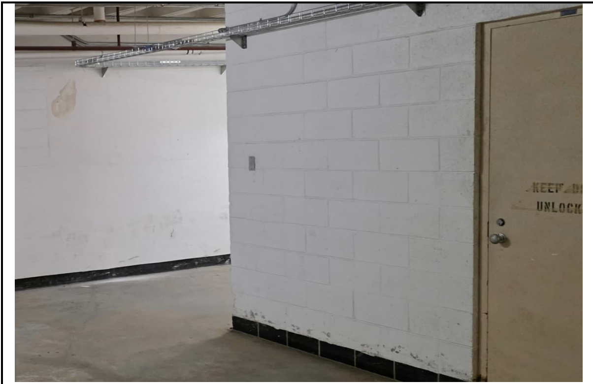
Photo 6: View of PC-4, white lead-containing paint, located on the Main building basement walls.
