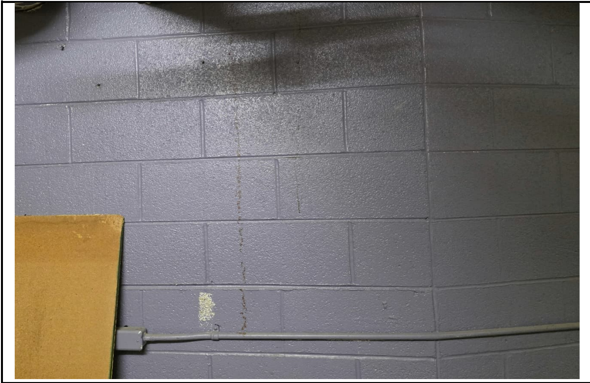
Photo 5: View of PC-3, purple lead-containing paint, located on the east wing basement walls.
