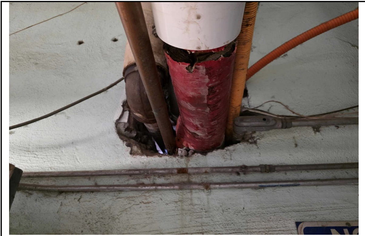
Photo 2: View of HA-3, asbestos-containing TSI layered paper pipe insulation and mudded fitting.
