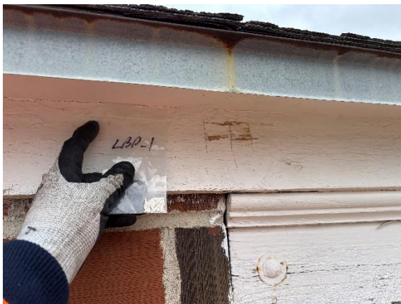
Photo #3 Lead-based paint (white) – CHMHI Fleet Garage exterior soffit. (3.7%)
