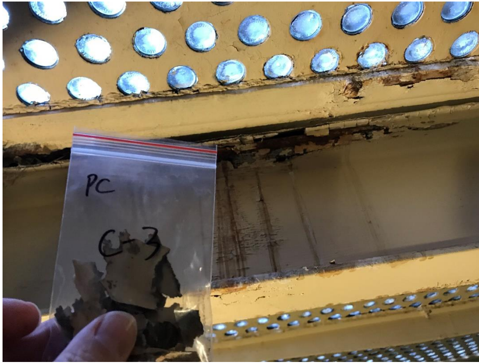
View of the Yellow Paint under the South Steps. (PC-C-3, 5.2 % Pb)
