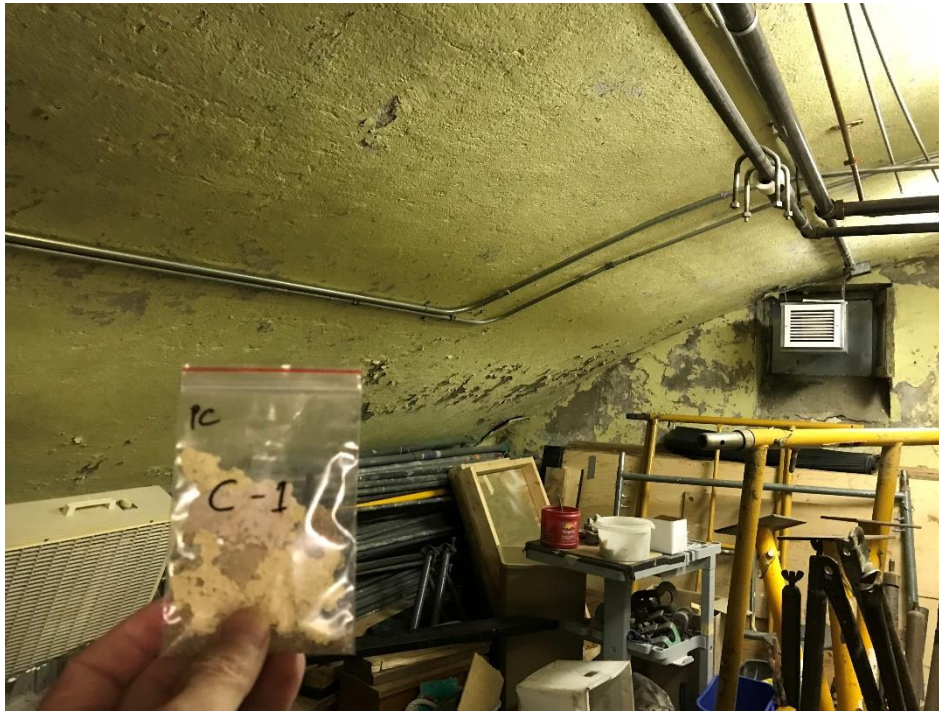
View of the Yellow Paint in Storage Tunnel. (PC-C-1, 0.22 % Pb)
