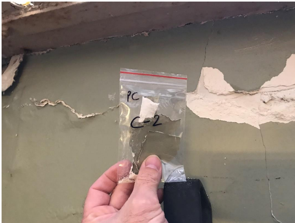
View of the Green Paint under the South Steps. (PC-C-2, 0.009 % Pb)
