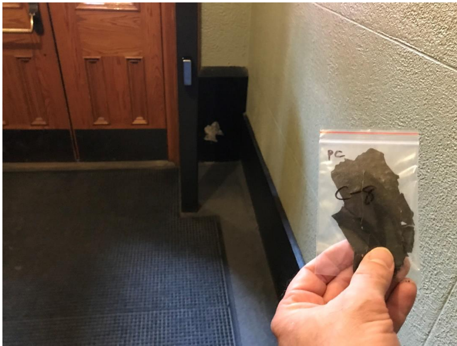
View of the Black Paint in the West Entrance. (PC-C-8, 2.7 % Pb)
