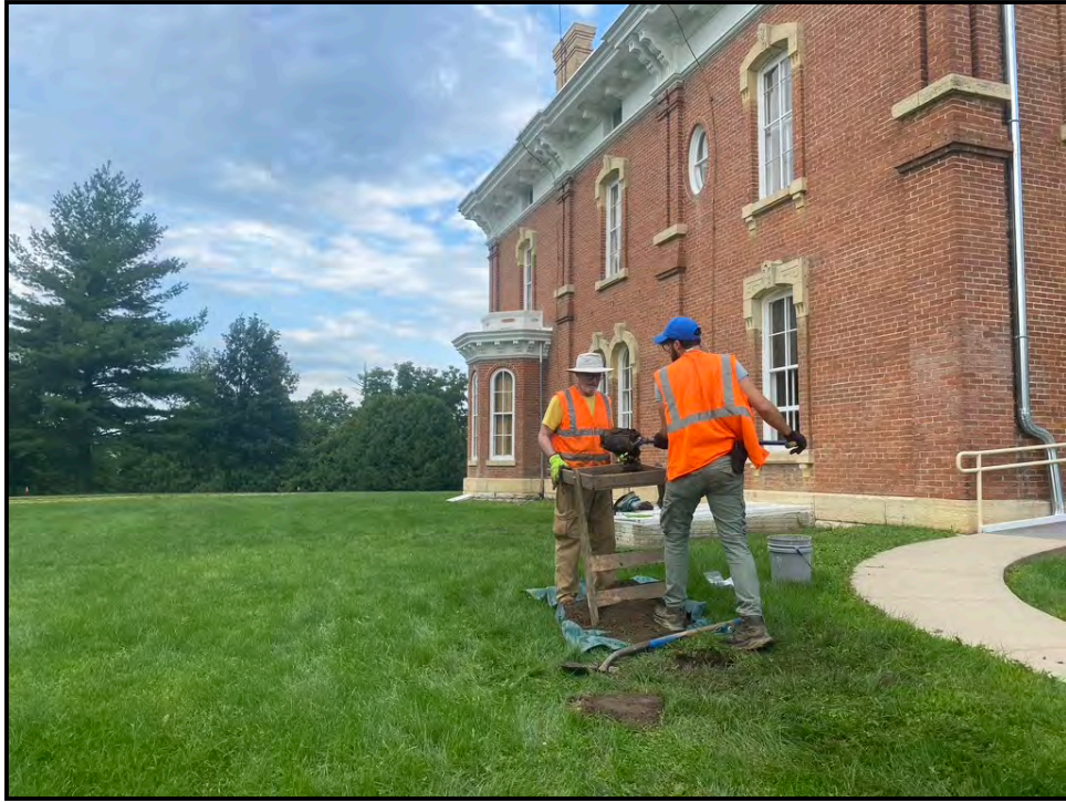
Figure 8. View of the East Yard and Auger Test T-17, view to the south.
